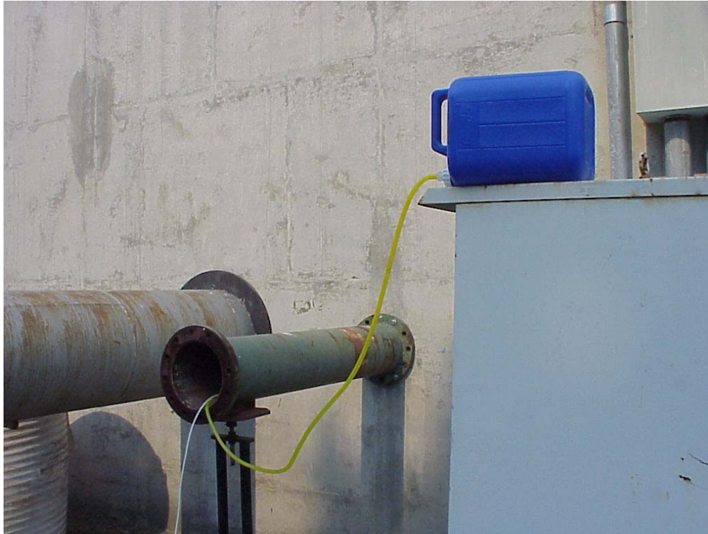
Figure 13. Fuel Tank and Feeding Line
