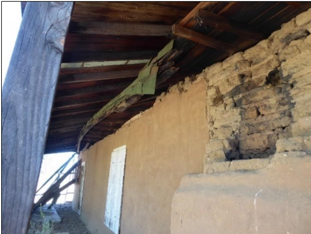
Figure 96. Collapsed roof under the top layer roof on the south side of the José María Gil Adobe, 2021. (ERDC-CERL)
