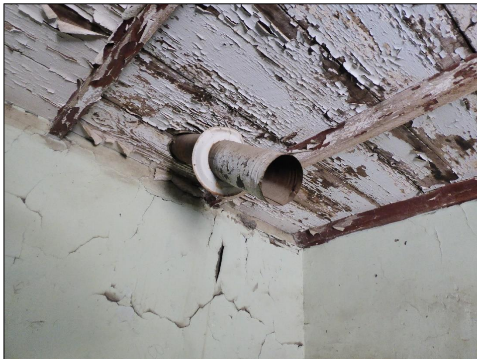
Figure 73. Existing stovepipe connection protruding from inner ceiling edge in the José María Gil Adobe, 2021. (ERDC-CERL.)
