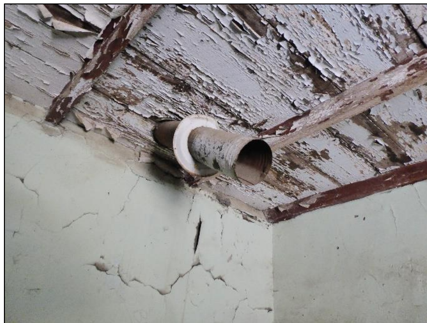
Figure 176. Metal stovepipe connection remaining in the south wing of the José María Gil Adobe, 2021. (ERDC-CERL.)
