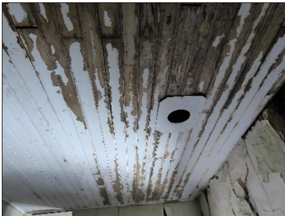
Figure 110. Beadboard ceiling in the northern portion of the José María Gil Adobe, 2021. (ERDC-CERL.)
