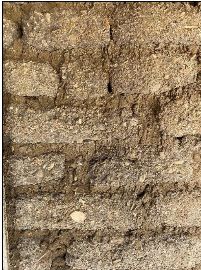
Figure 85. Exposed adobe bricks and mortar on the José María Gil Adobe, 2021. (ERDC-CERL.)
