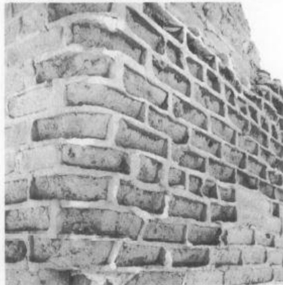
Cement Mortar Incompatibility. The stronger and less flexible cement mortar has caused the softer adobe bricks to crumble thus leaving a "honeycomb" of cement mortar joints. (National Park Service)
