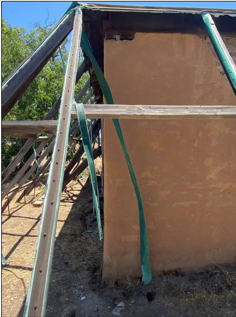
Figure 61. Uneven surface and flare of adobe wall at the base on the north corner of the José María Gil Adobe, 2021. (ERDC-CERL.)
