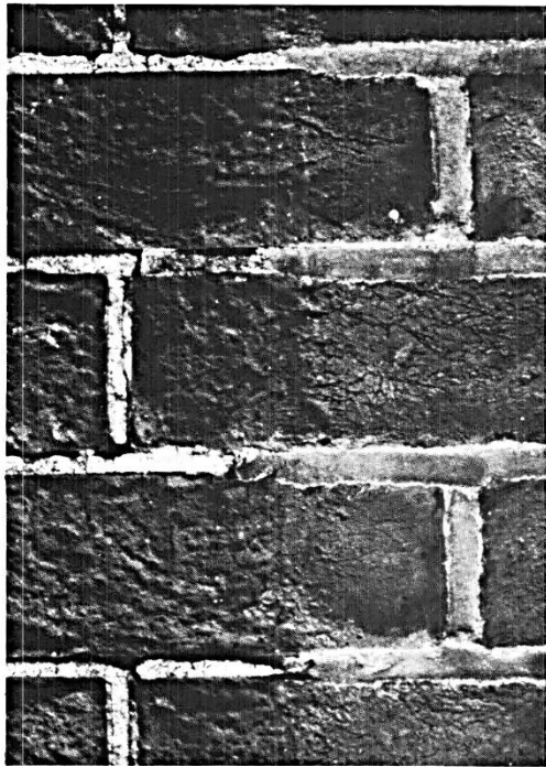
Abractively Cleaned vs. Untouched Brick. Two brick rowhouses with a common façade provide an excellent point of comparison when one of the houses has been sandblasted. It is clear that abrasive blasting, by removing the outer surface, has left the brickwork on the left rough and pitted, while that on the right still exhibits an undamaged and relatively smooth surface. Note that the abrasive cleaning has also removed a considerable portion of the mortar from the joints of the brick on the left side, which will require repointing.
