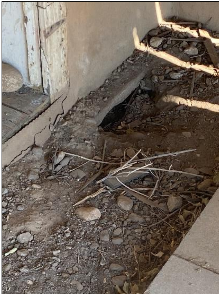
Figure 103. Wooden sill supporting the base of the adobe wall at grade level of the José María Gil Adobe, 2021. (ERDC-CERL.)
