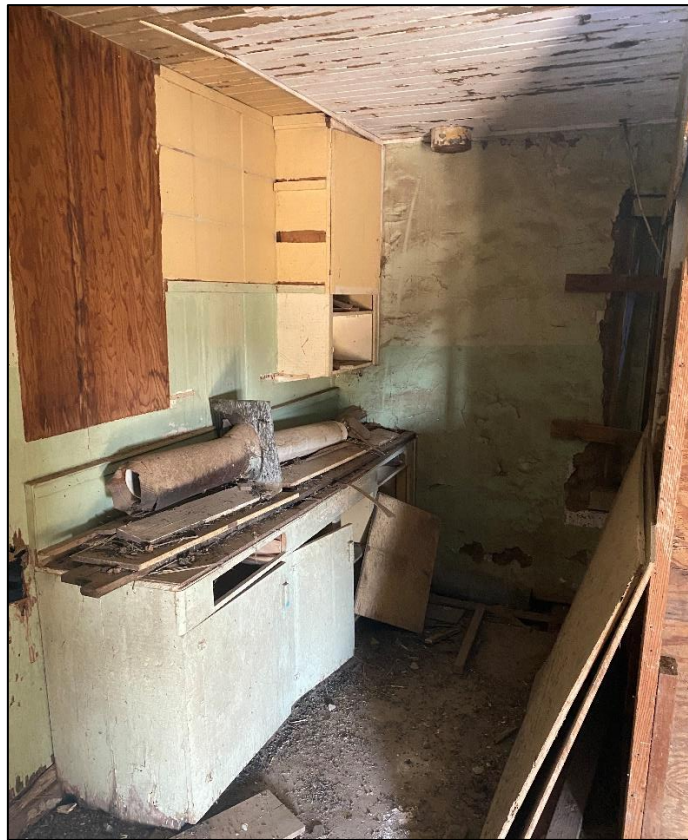
Figure 70. Kitchen components in the north wing of the José María Gil Adobe, 2021. (ERDC-CERL.)
