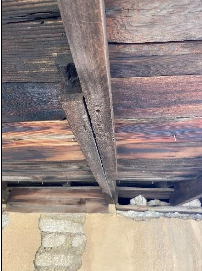
Figure 95. Looking at the connection between the veranda roof to the roof of the José María Gil Adobe, 2021. (ERDC-CERL.)
