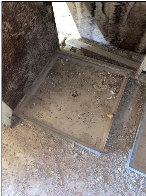
Figure 170. Square, metal shower floor covered in guano in the north wing of the José María Gil Adobe, 2021. (ERDC-CERL.)
