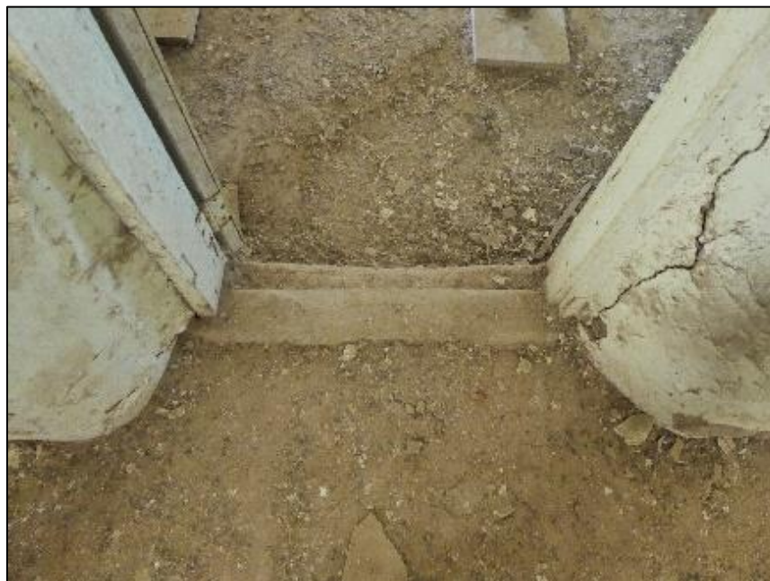
Figure 124. Wooden threshold transition between two rooms in the south wing of the José María Gil Adobe, 2021. (ERDC-CERL.)
