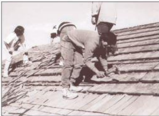
3. Drive in or pull out existing nails and repair or replace damaged purlins.
