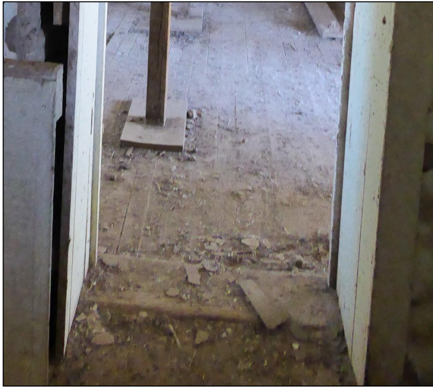
Figure 66. Wooden floor with extensive dirt and guano in the south wing of the José María Gil Adobe, 2021. (ERDC-CERL.)
