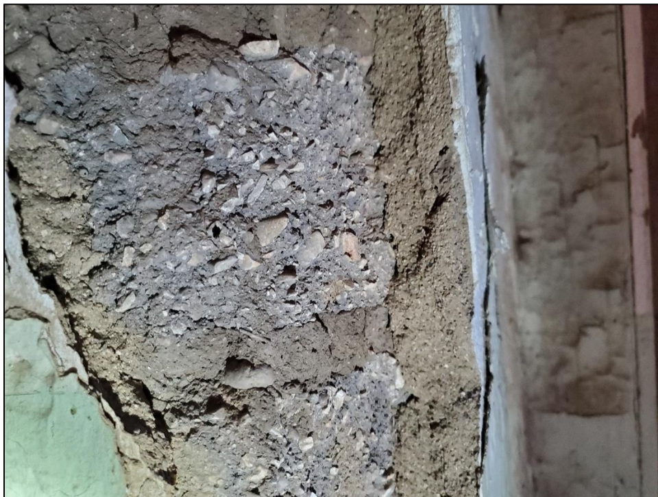
Figure 193. Bricks (sample 9) on the west side of the main structure, having light-gray color with angular aggregates and lacking straw reinforcement.
