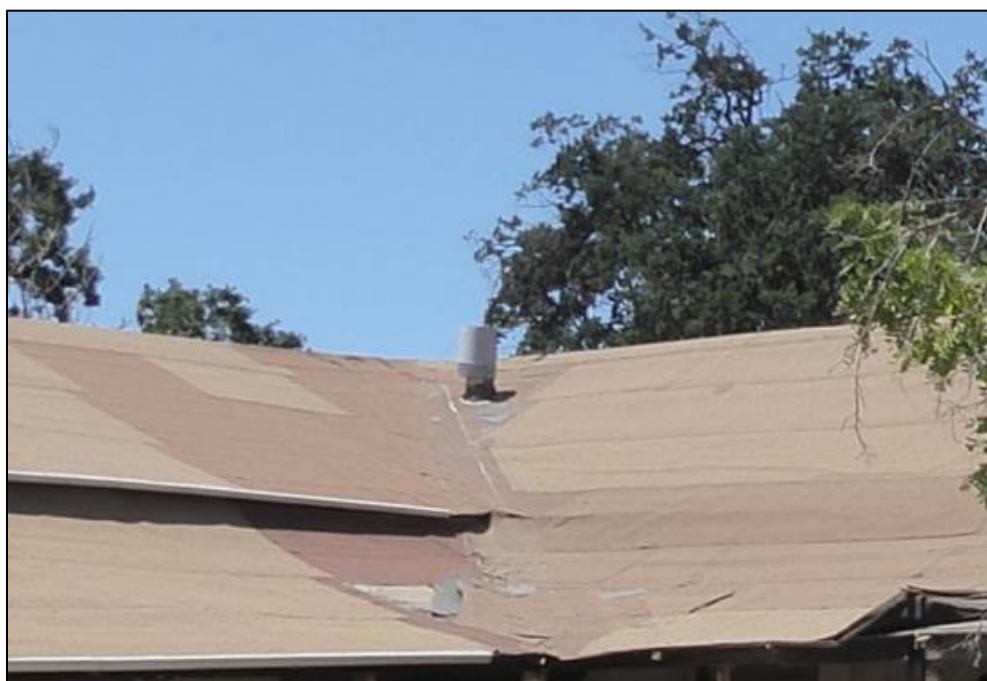
Figure 160. Metal stovepipe in the inner corner of the intersection of the north and south wings of the José María Gil Adobe, 2021. (ERDC-CERL.)
