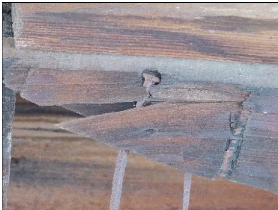
Figure 161. Rusted square nails on an exterior support frame of the José María Gil Adobe, 2021. (ERDC-CERL.)
