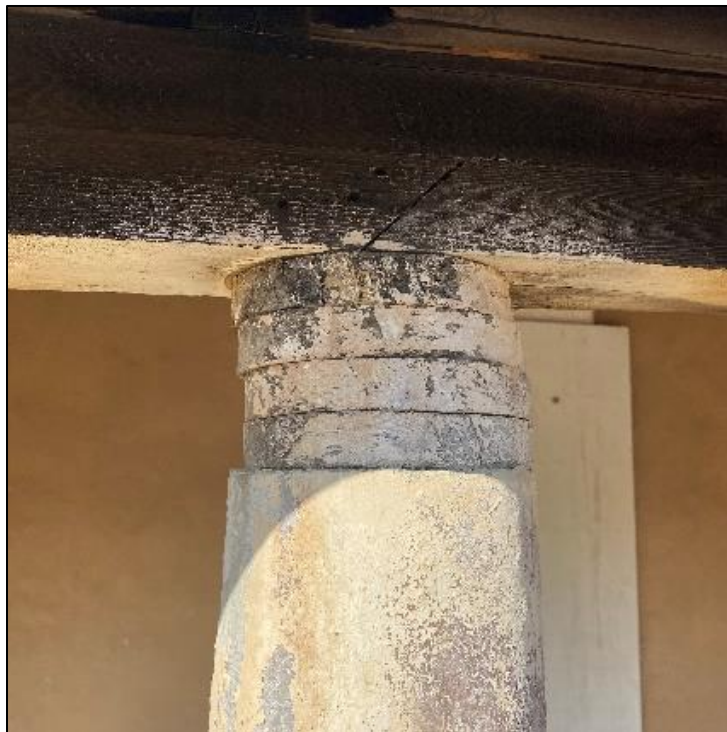
Figure 105. Wooden disks on top of the concrete columns supporting the veranda roof, possibly for leveling purposes, on the José María Gil Adobe, 2021. (ERDC-CERL.)
