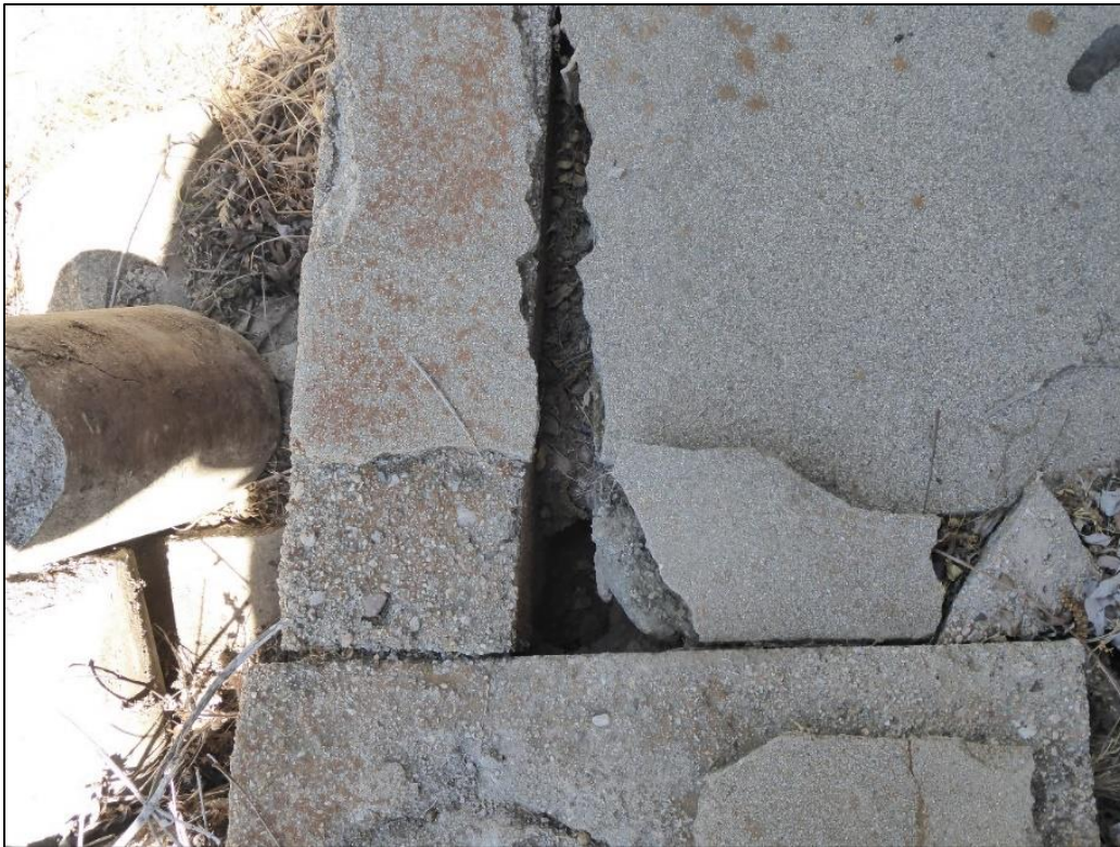
Figure 135. Spalling and cracking of concrete on the south side of the porch floor of the José María Gil Adobe, 2021. (ERDC-CERL.)
