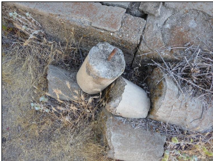
Figure 137. Crumbled concrete column showing metal reinforcement, on the southwest side of the José María Gil Adobe, 2021. (ERDC-CERL.)
