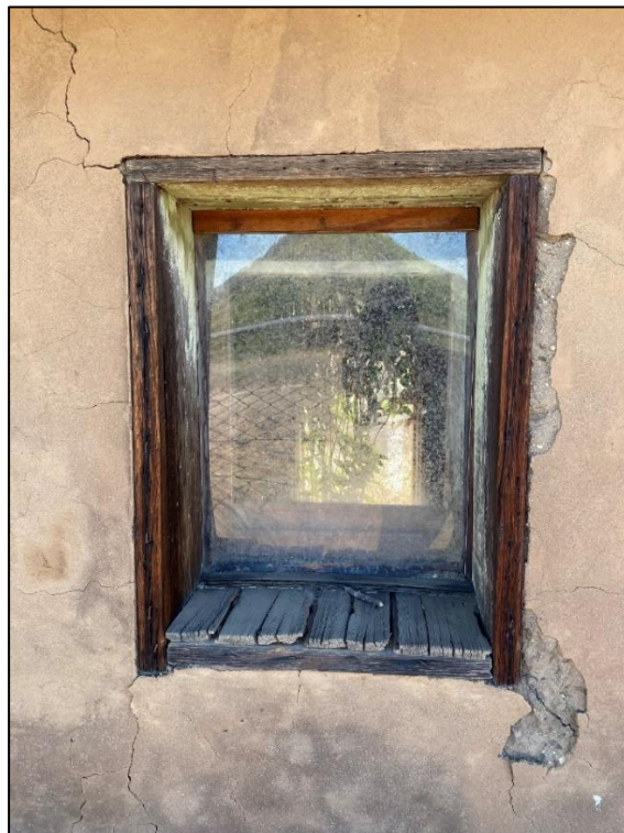
Figure 49. Wooden window trim and sill boards on the cold storage building, 2021. (ERDC-CERL.)
