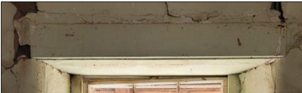
Figure 121. Wooden window header covered with wooden trim in the south wing in the José María Gil Adobe, 2021. (ERDC-CERL.)
