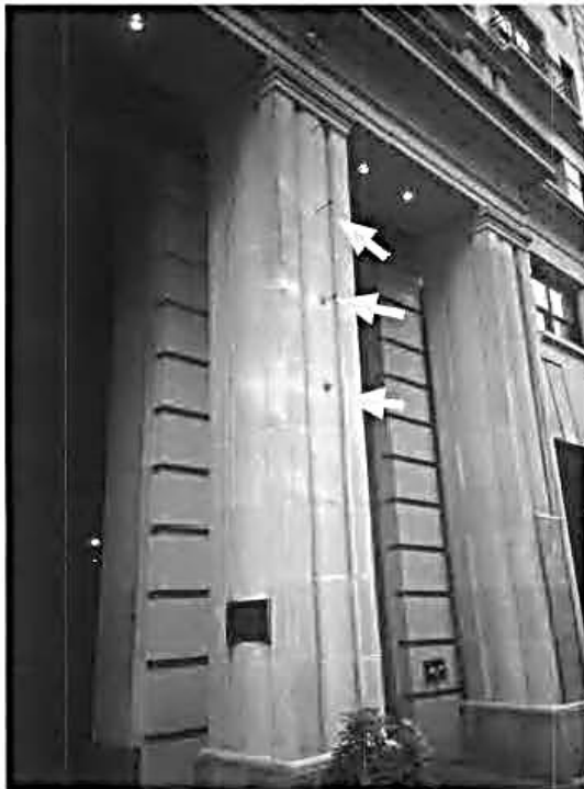
Figure 10. High-pressure water washing too close to the surface has abraded and, consequently, marred the limestone on this early-20th century building.
