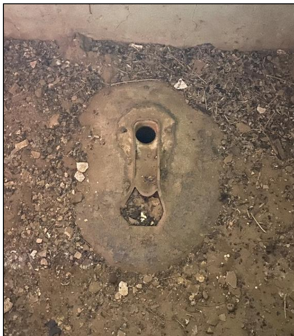
Figure 171. Metal toilet plumbing connection near the shower floors in the north wing of the José María Gil Adobe, 2021. (ERDC-CERL.)
