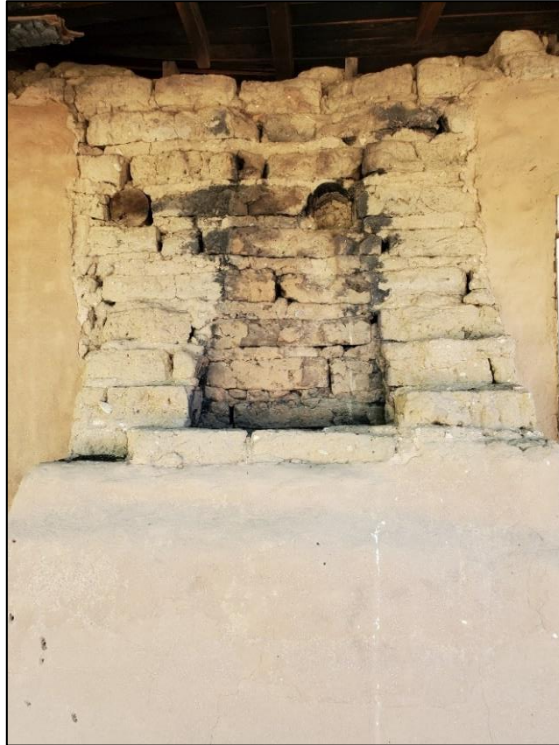
Figure 191. Two stuccos ( top and bottom ) (samples 17b and 18) of different color and edge quality on the south exterior wall, indicating different time periods of application.
