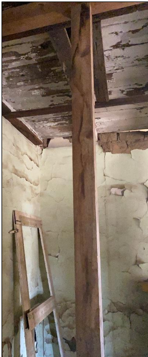
Figure 111. Wooden 4 × 4 in. post supporting the ceiling in the José María Gil Adobe, 2021. (ERDC-CERL.)
