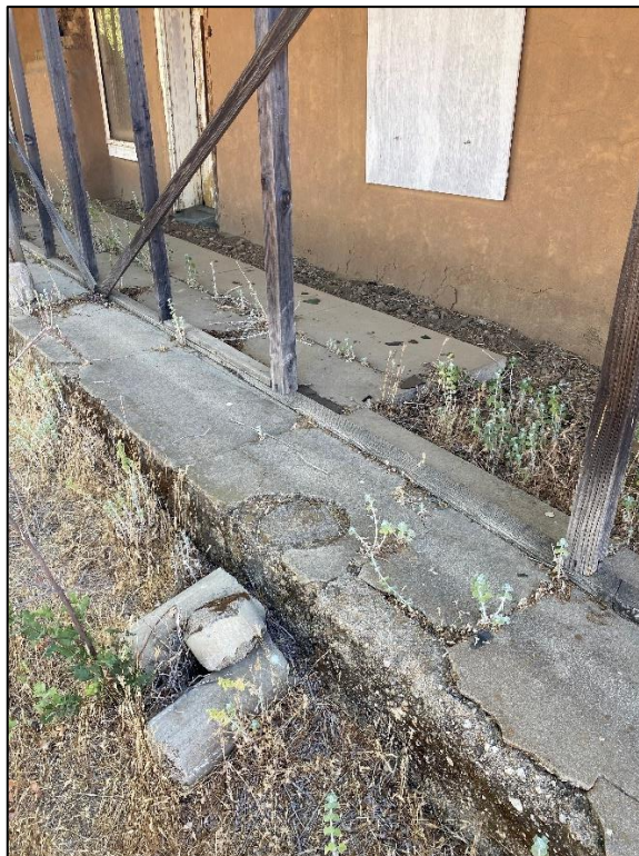
Figure 134. Raised concrete porch floor on the southwest side of the José María Gil Adobe, 2021. (ERDC-CERL.)
