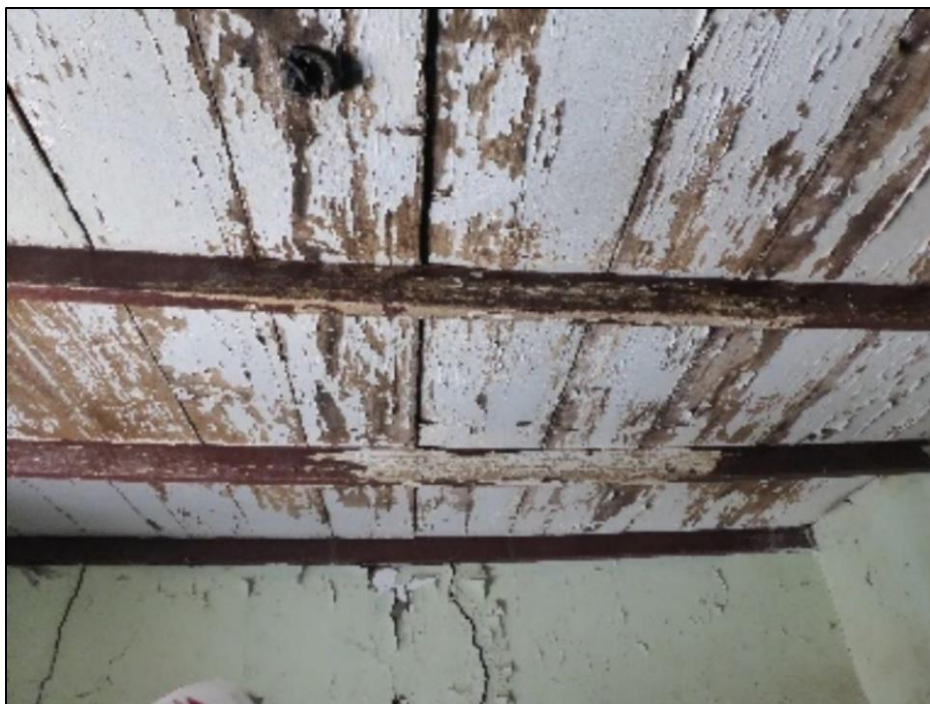
Figure 109. Wooden ceiling joists, 2 × 4 in., supporting wooden ceiling boards in the José María Gil Adobe, 2021. (ERDC-CERL.)
