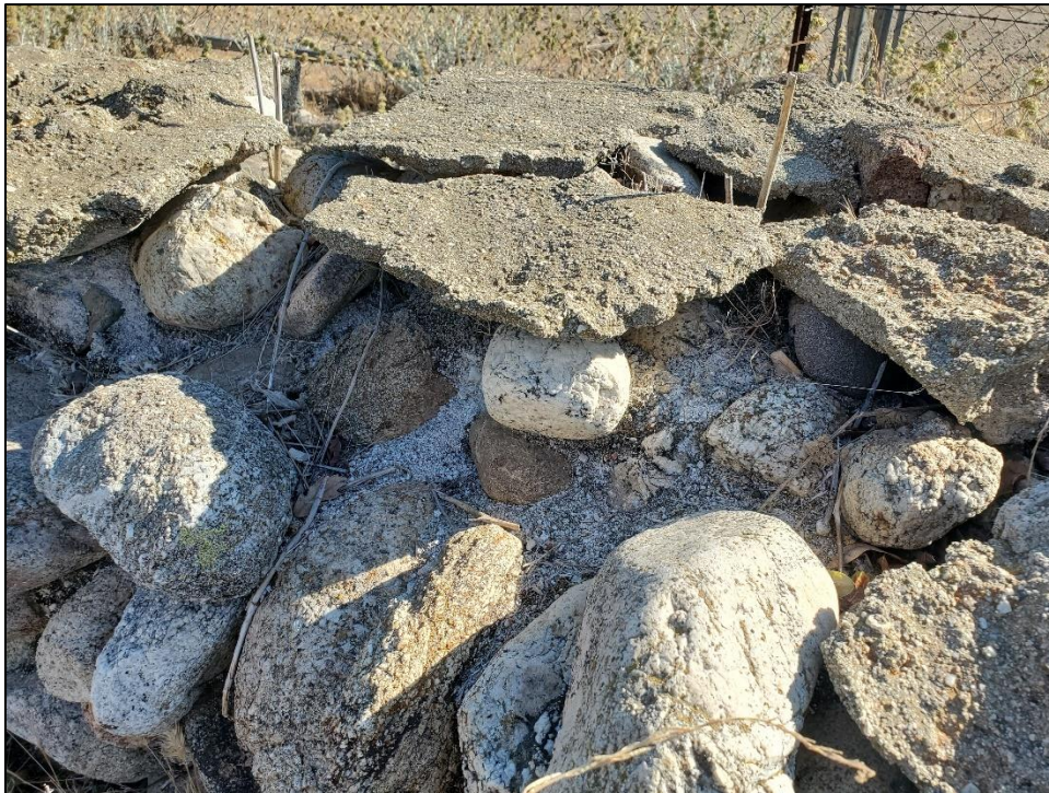
Figure 183. Broken top pieces of perimeter wall (sample 1).
