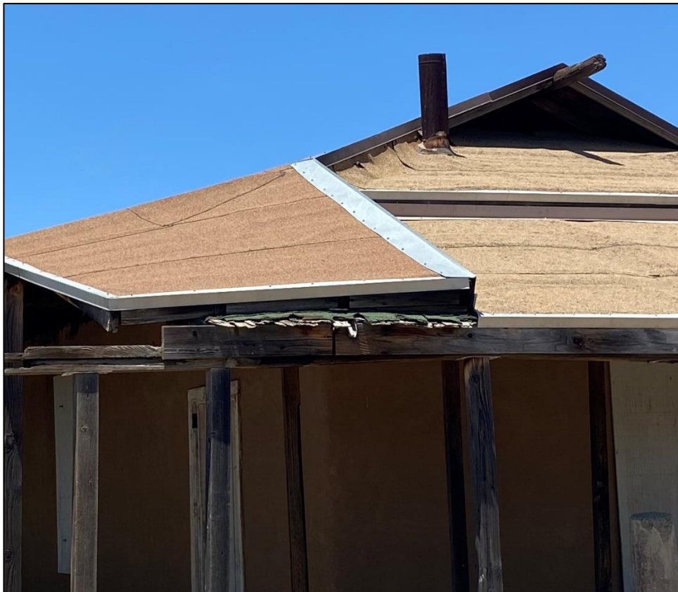
Figure 55. Multiple roof layers showing green asphalt shingles and brown asphalt paper on the south corner of the José María Gil Adobe, 2021. (ERDC-CERL.)
