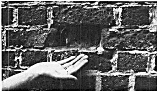
Spalling Brick. This soft, early 19th-century brick was sandblasted in the 1960s; consequently, severe spalling has resulted. Some bricks have almost totally disintegrated, and will eventually have to be replaced. (Robert S. Gamble)
