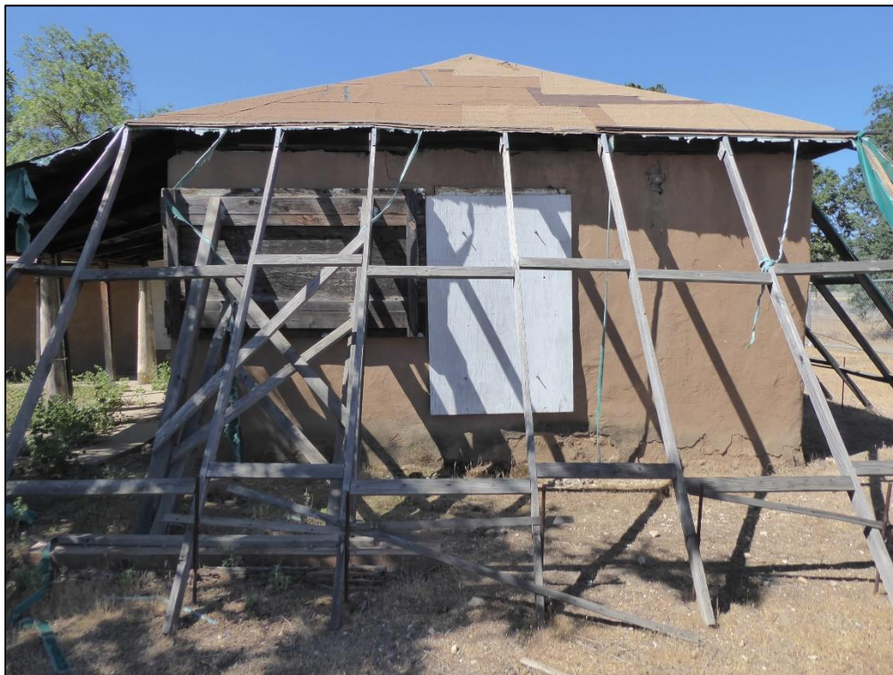
Figure 104. Wooden support braces supporting the northeast wall of the José María Gil Adobe, 2021. (ERDC-CERL.)
