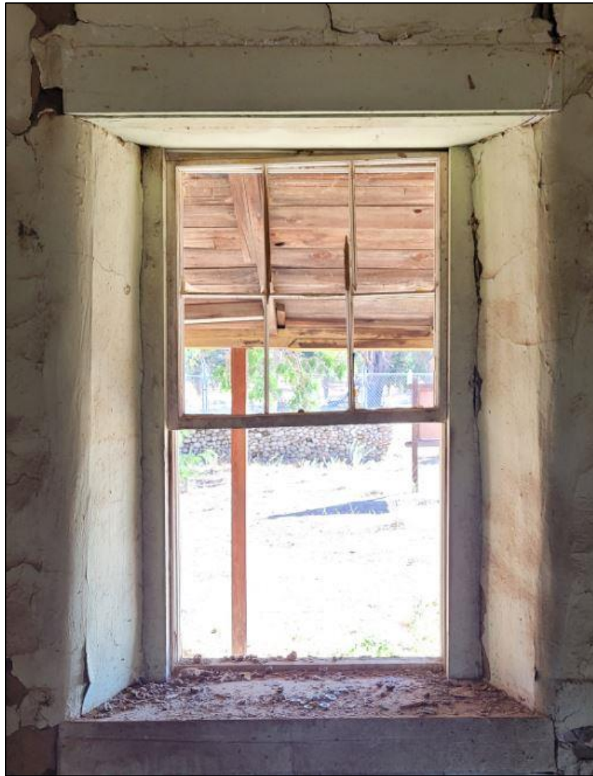
Figure 120. Remnants of a six-over-six, wood-sash, double-hung window on the south wing of the José María Gil Adobe, 2021. (ERDC-CERL.)
