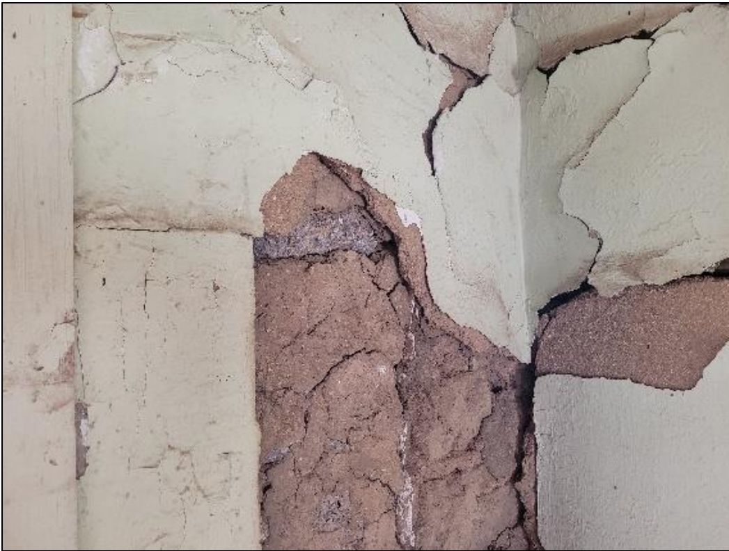
Figure 89. Cracked plaster and paint exposing adobe brick in the south wing of the José María Gil Adobe, 2021. (ERDC-CERL.)
