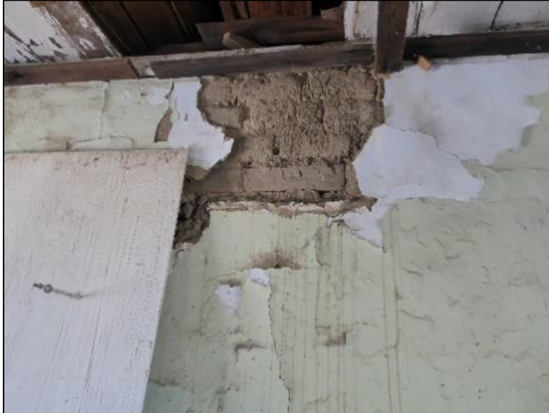
Figure 125. Wooden element embedded within the adobe wall in the south wing of the José María Gil Adobe, 2021. (ERDC-CERL.)
