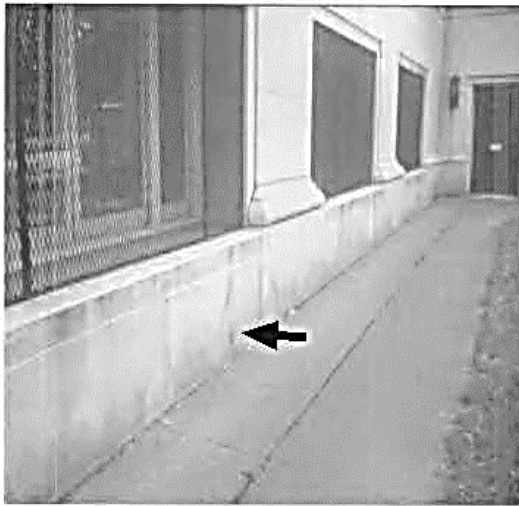
Figure 2. Biological growth as shown on this marble foundation can usually be removed using a low-pressure water wash, possibly with a non-ionic detergent added to it, and scrubbing with a natural or synthetic bristle brush.
