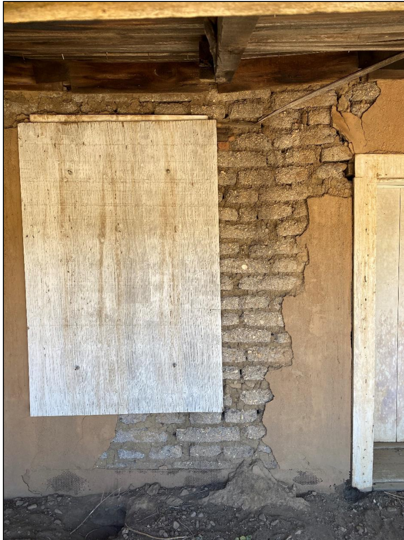
Figure 60. Plaster coating and exposed adobe brick on the north wing of the José María Gil Adobe, 2021. (ERDC-CERL.)
