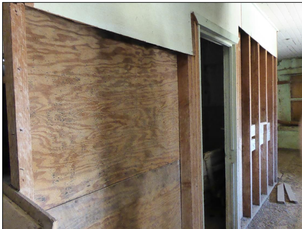
Figure 69. Wooden partition walls in the north wing of the José María Gil Adobe, 2021. (ERDC-CERL.)
