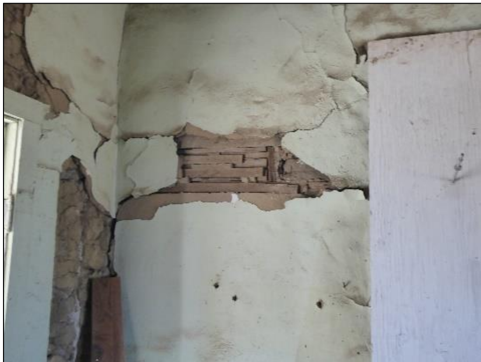
Figure 90. Cracked plaster and paint exposing wooden elements in the south wing of the José María Gil Adobe, 2021. (ERDC-CERL.)
