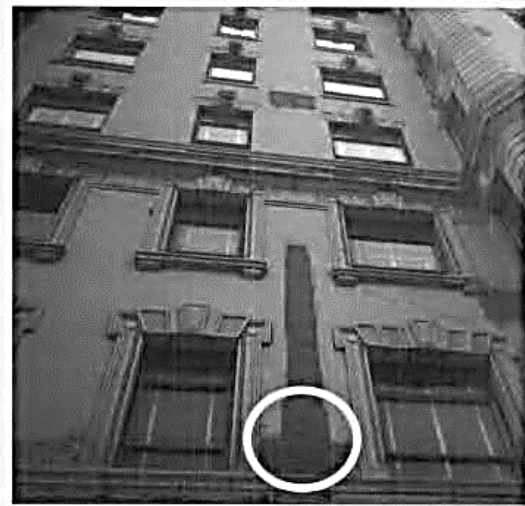
Figure 3. This small test area has revealed a red brick patch that does not match the original beige brick. This may explain why the building was painted, and may suggest to the owner that it may be preferable to keep it painted.
