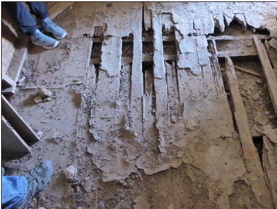
Figure 113. Wood strip flooring with breakthrough areas in a central location of a floor in the José María Gil Adobe, 2021. (ERDC-CERL.)
