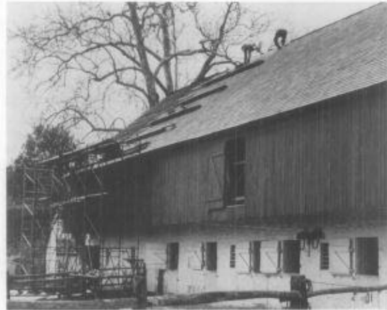
11. The replacement sawn red cedar shingles matched the deteriorated shingles exactly for this barn re-roofing. The old shingles, seen to the far left, were removed as the new shingles were installed. Even the horizontal coursing matched because the exposure length for both old and new shingles was the same. Photo: Williamsport Preservation Training Center.
