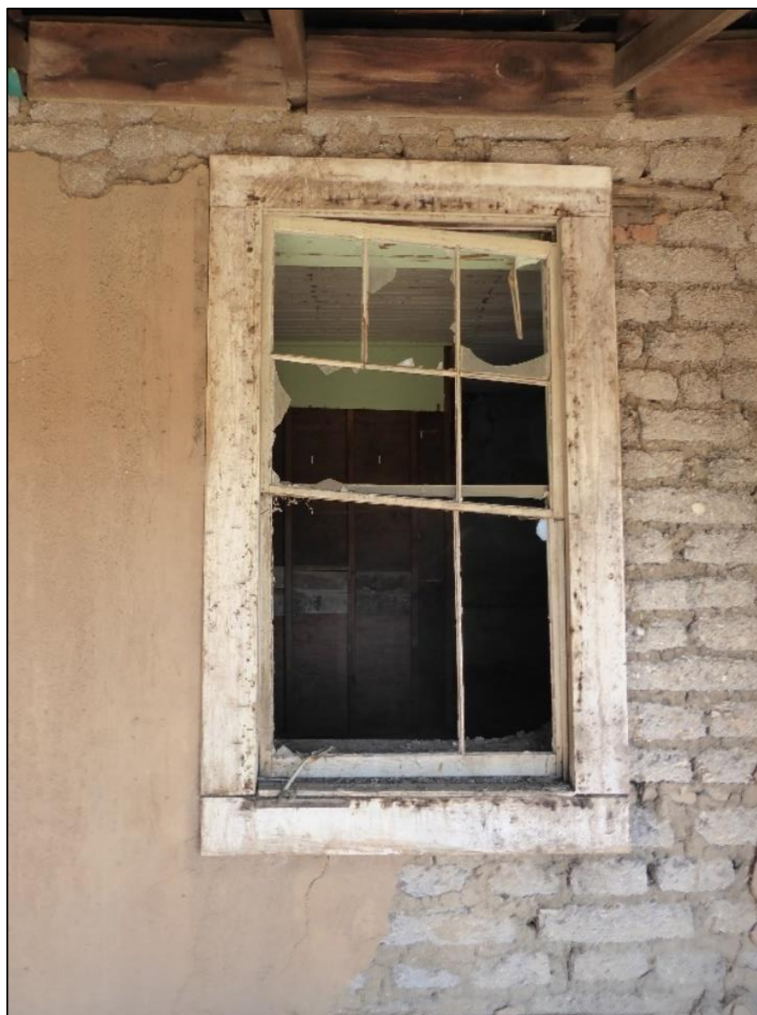
Figure 99. Sagging windows and missing muntins on the west side of the José María Gil Adobe, 2021. (ERDC-CERL.)
