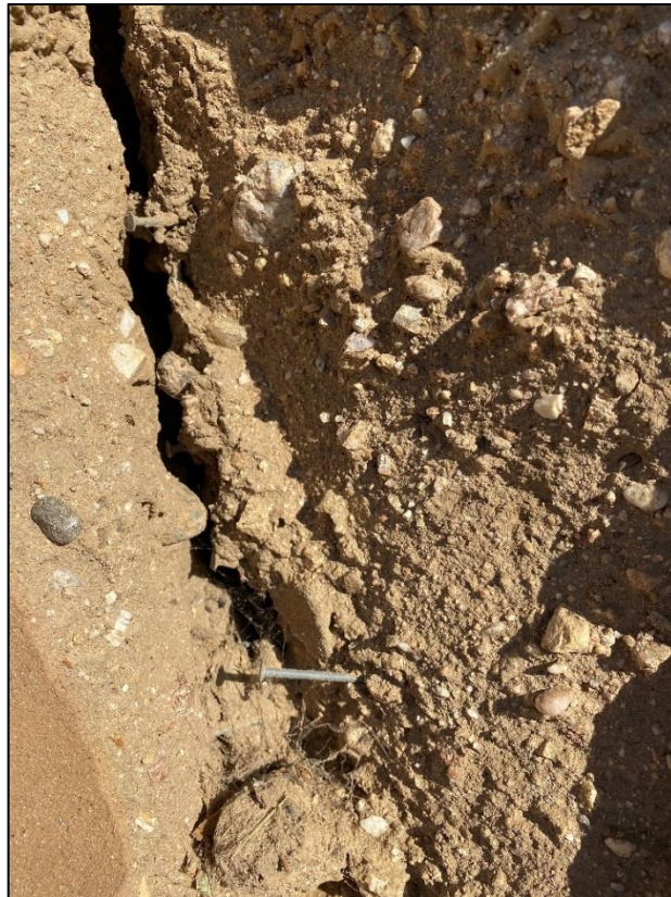
Figure 43. Rammed earth material exposed in crack on the southeast side of the cold storage building, 2021. (ERDC-CERL.)
