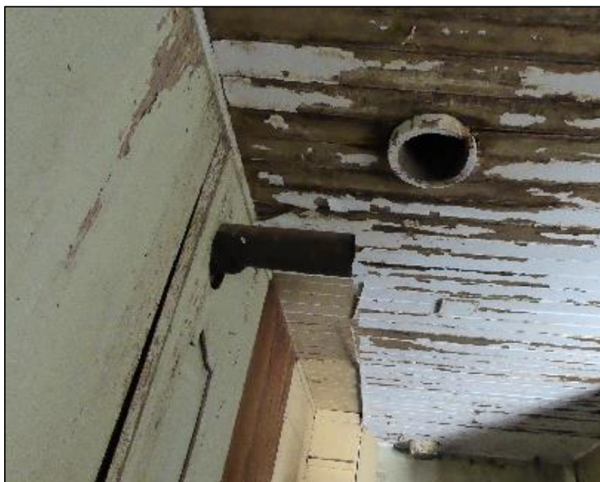
Figure 177. Metal stovepipe connection remaining on a wall and a chimney pipe remaining in the ceiling in the north wing of the José María Gil Adobe, 2021. (ERDC-CERL.)
