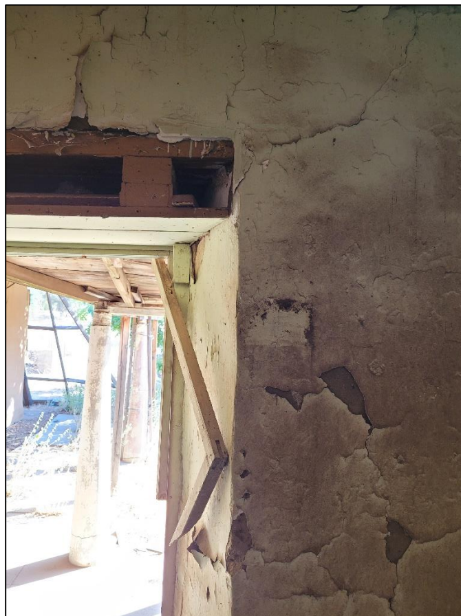
Figure 122. Exposed wooden window header in the south wing of the José María Gil Adobe, 2021. (ERDC-CERL.)
