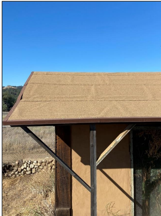
Figure 42. Brown asphalt paper on the roof of the cold storage building, 2021. (ERDC-CERL.)
