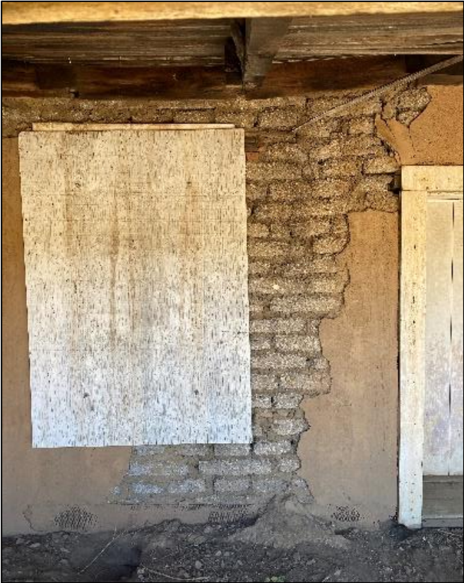
Figure 86. Large section of adobe brick between a door and window on the southeast side of the José María Gil Adobe, 2021. (ERDC-CERL.)
