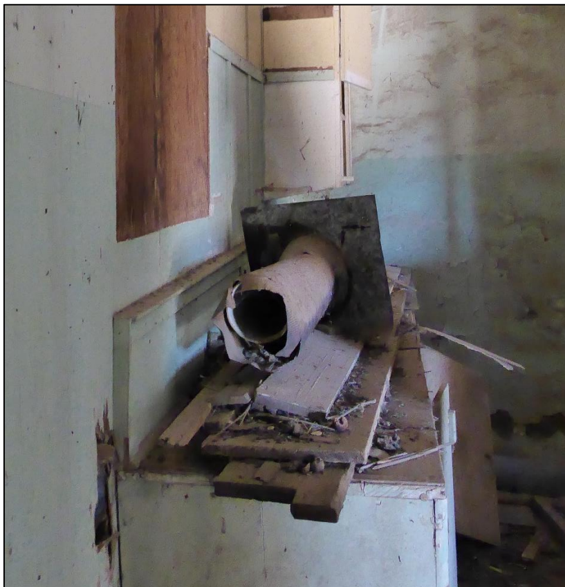
Figure 179. Metal stovepipe now on counter in the north wing of the José María Gil Adobe, 2021. (ERDC-CERL.)
