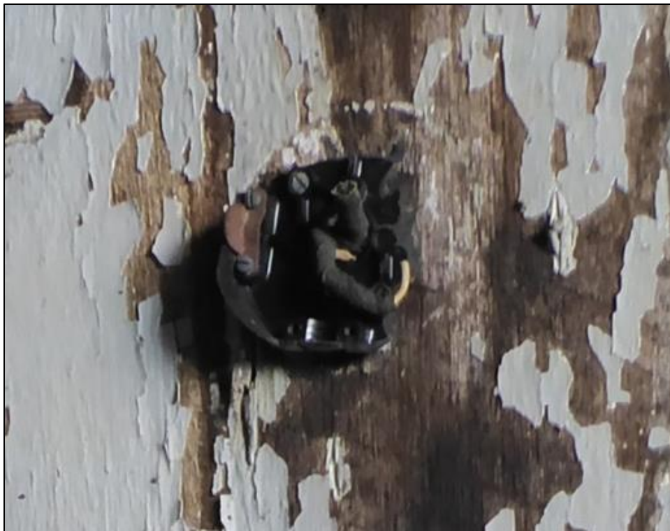
Figure 72. Electrical sockets on ceilings of various rooms of the José María Gil Adobe, 2021. (ERDC-CERL.)
