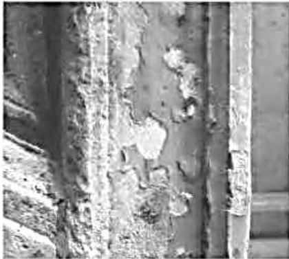
Figure 25. The clear coating applied to this limestone molding has failed and is taking off some of the stone surface as it peels. Photo: Frances Gale.
