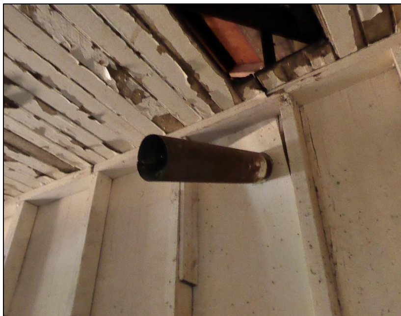
Figure 178. Metal stovepipe protruding from the wall in the north wing of the José María Gil Adobe, 2021. (ERDC-CERL.)
