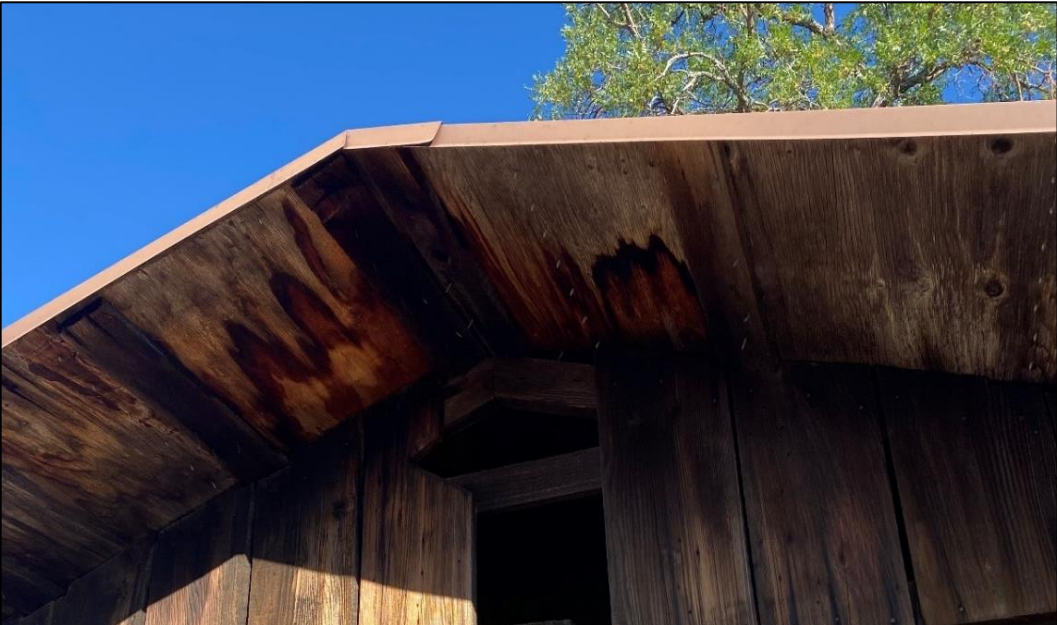
Figure 46. Wooden soffits under the roof overhang of the cold storage building, 2021. (ERDC-CERL.)
