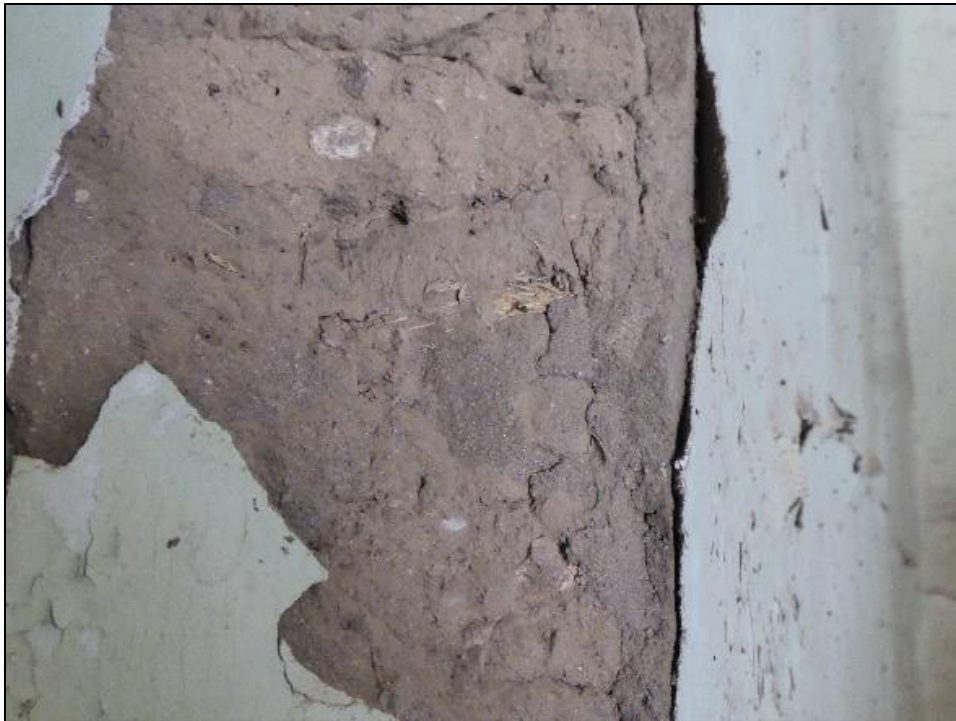
Figure 91. Intact plaster with peeling paint in the south wing of the José María Gil Adobe, 2021. (ERDC-CERL.)
