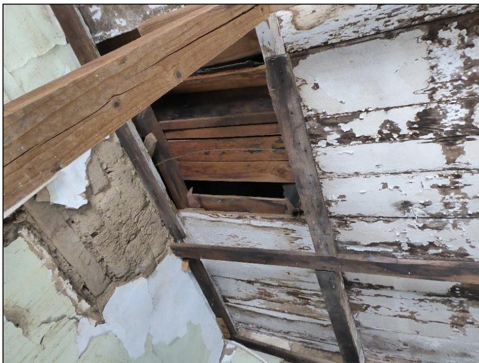
Figure 108. Multisized and multiaged wooden members supporting the ceiling within the José María Gil Adobe, 2021. (ERDC-CERL.)
