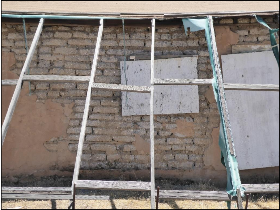
Figure 87. Large section of adobe brick around two windows on the northwest side of the José María Gil Adobe, 2021. (ERDC-CERL.)
