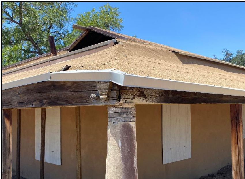
Figure 156. Aluminum drip edge that lines the edge of the roof of the José María Gil Adobe, 2021. (ERDC-CERL.)
