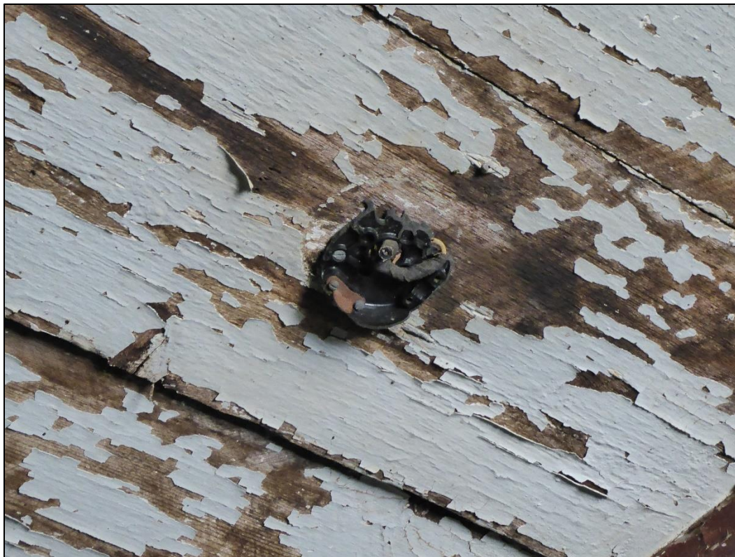
Figure 180. Remaining light fixture attachment in the south wing of the José María Gil Adobe, 2021. (ERDC-CERL.)
