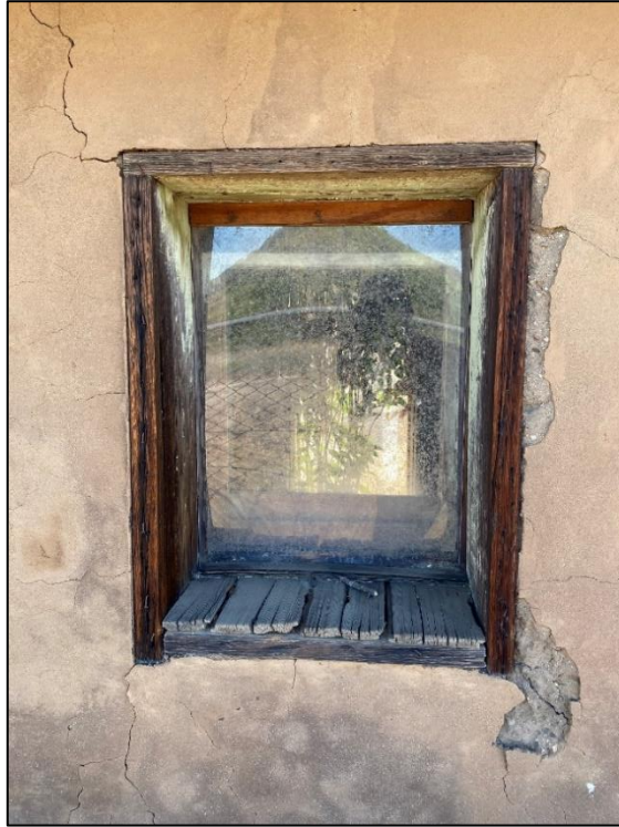
Figure 41. Plexiglass in the window opening on the southwest side of the cold storage building, 2021. (ERDC-CERL.)
