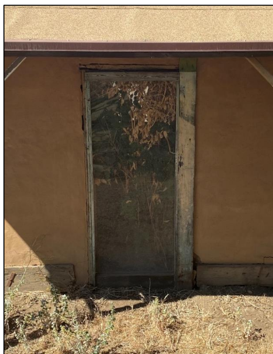
Figure 40. Plexiglass in the door opening on the northeast side of the cold storage building, 2021. (ERDC-CERL.)
