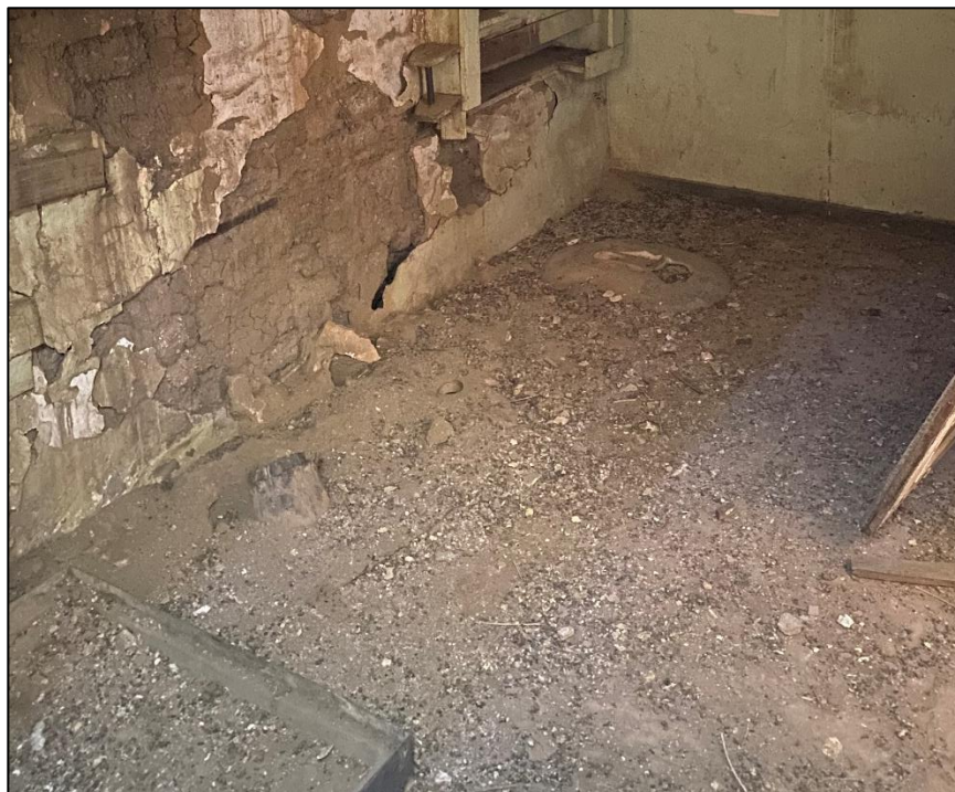
Figure 67. Floor that appears to be dirt due to excessive coverage of dirt and guano in the north wing of the José María Gil Adobe, 2021. (ERDC-CERL.)
