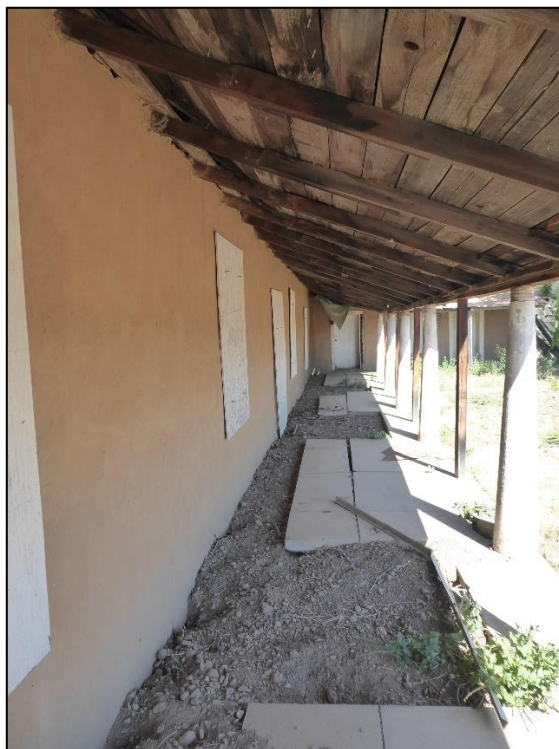
Figure 59. Looking northwest at the concrete veranda floor on the east side of the José María Gil Adobe, 2021. (ERDC-CERL.)
