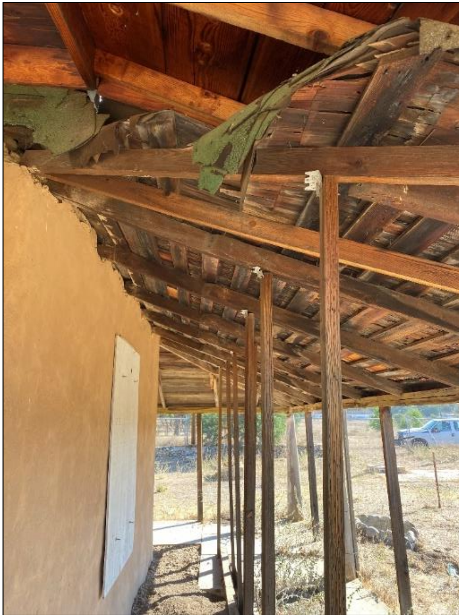
Figure 93. All wood support types, 2 × 4 in. and 4 × 4 in., as structural components for the veranda roof of the José María Gil Adobe, 2021. (ERDC-CERL.)
