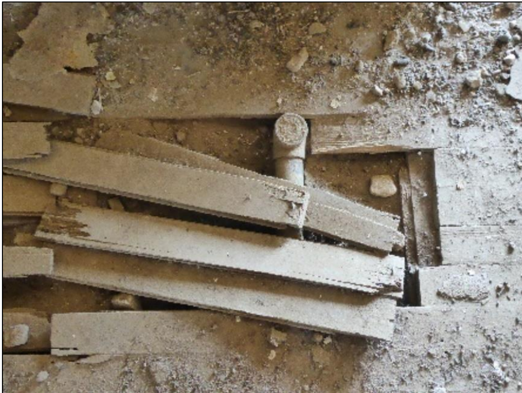
Figure 114. Broken wood strip flooring piled near exposed plumbing in the José María Gil Adobe, 2021. (ERDC-CERL.)
