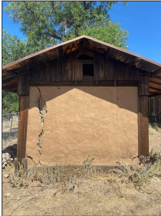
Figure 48. Wooden trim boards along base and corners of the cold storage building, 2021. (ERDC-CERL.)
