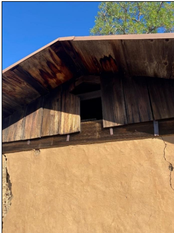
Figure 45. Vertically placed boards cladding the gable opening on the north and south sides of the cold storage building, 2021. (ERDC-CERL.)
