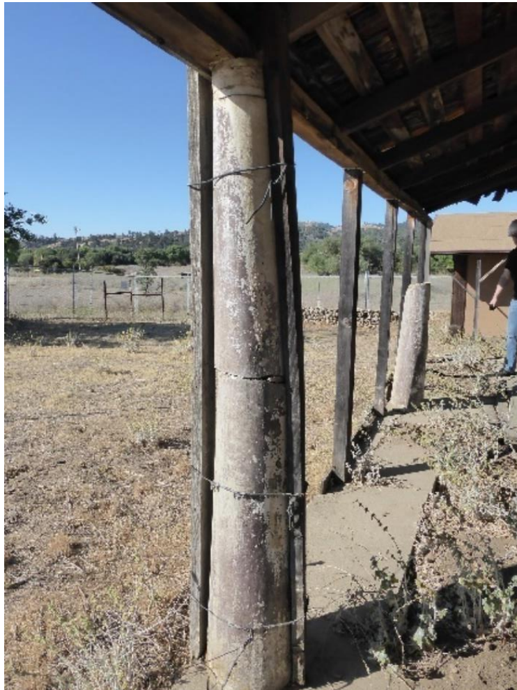
Figure 106. Two wooden 2 × 4 in. boards supporting a concrete column that is cracked in multiple places, 2021. (ERDC-CERL.)
