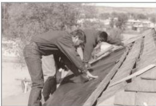
5. Carefully remove kraft paper from underside of the shield. Work from one end to the other. Carefully place the shield on roof surface.
