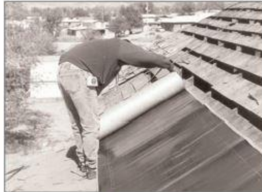
4. Ice and water shield should be installed on all overhangs. Roll out shield, cut to a workable length, and cut to fit at the hip if a hip exists.
