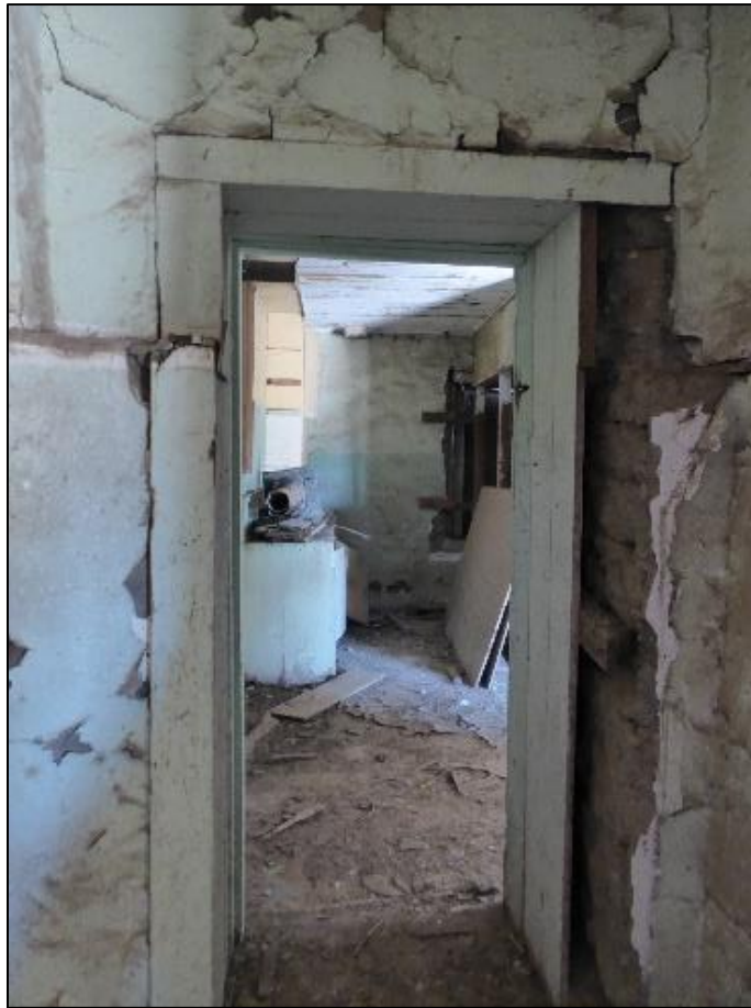
Figure 119. Interior wooden door trim with a missing board on the right side in the José María Gil Adobe, 2021. (ERDC-CERL.)
