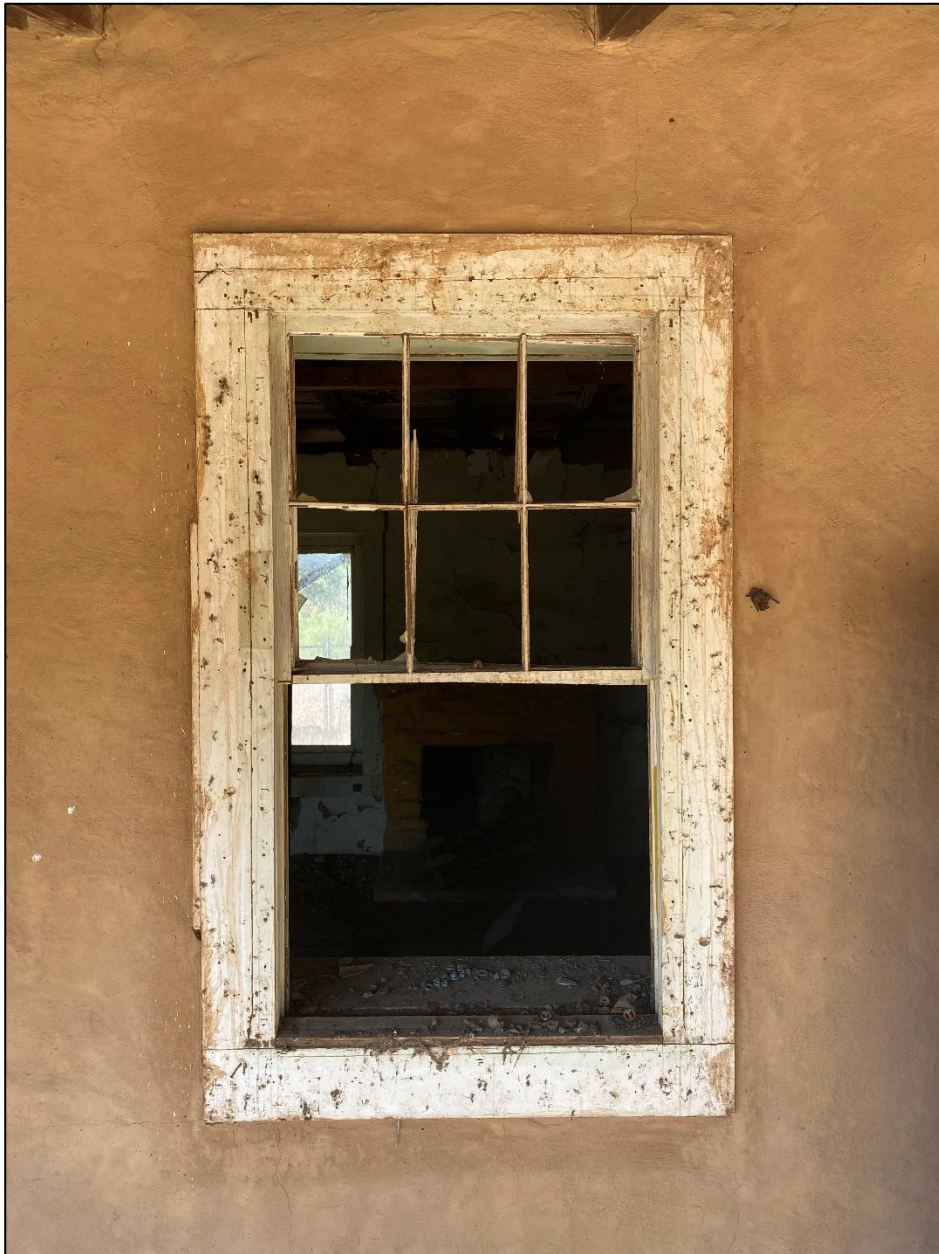
Figure 62. Example of a six-over-six, wood-sash, double-hung wood window that is missing muntins on the east side of the José María Gil Adobe, 2021. (ERDC-CERL.)
