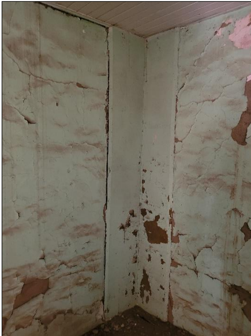
Figure 131. Floor to ceiling wooden element in the northmost corner of the José María Gil Adobe, 2021. (ERDC-CERL.)
