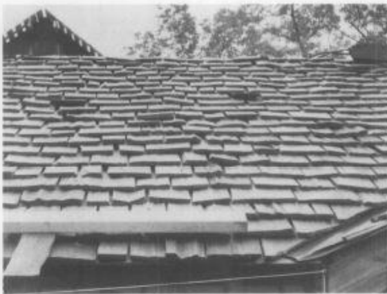
15. These commercially available roofing products with rustic split faces are not appropriate for historic preservation projects. In addition to the inaccurate appearance, the irregular surfaces and often wide spaces between shingles will allow wind-driven moisture to penetrate up and under them. The excessively wide boards will tend to cup, curl and crack. Moss, lichens and debris will have a tendency to collect on these irregular surfaces, further deteriorating the roofing. Photo: Sharon C. Park.
