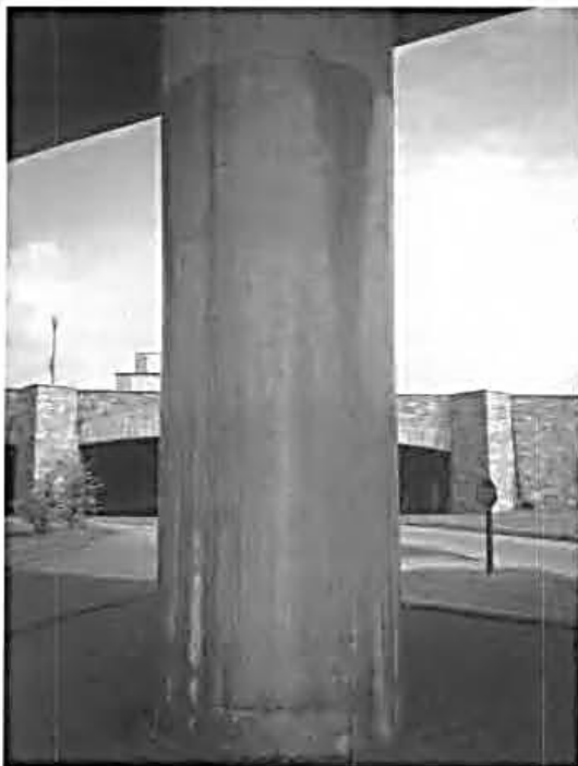
Figure 26. The anti-graffiti or barrier coating on this column is very shiny and would not be appropriate to use on a historic masonry building. The coating has discolored as it has aged and whitish streaks reveal areas of bare concrete where the coating was incompletely applied.
