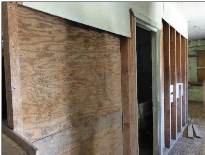
Figure 129. Wooden partition wall using plywood and studs, framing the bathroom space in the north wing of the José María Gil Adobe, 2021. (ERDC-CERL.)
