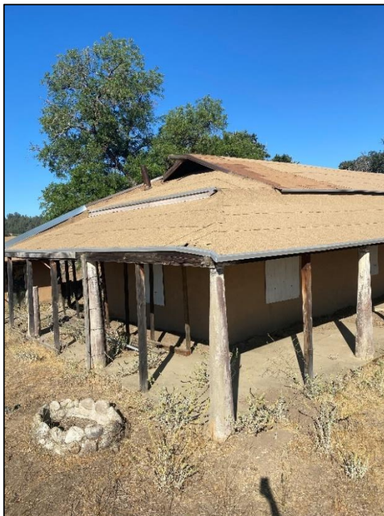
Figure 58. Concrete columns and wooden braces supporting the veranda of the José María Gil Adobe, 2021. (ERDC-CERL.)
