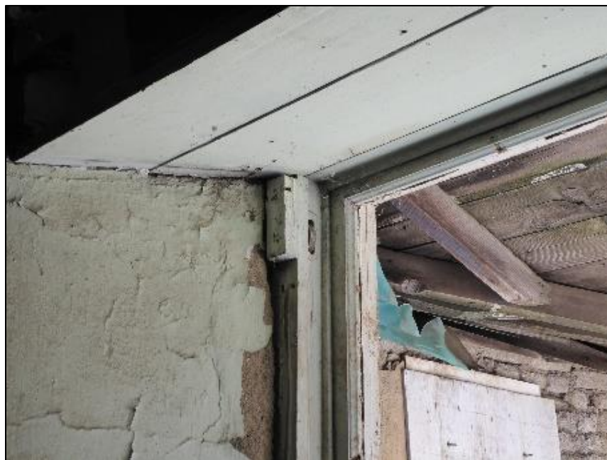
Figure 123. Wooden door header in the south wing of the José María Gil Adobe, 2021. (ERDC-CERL.)
