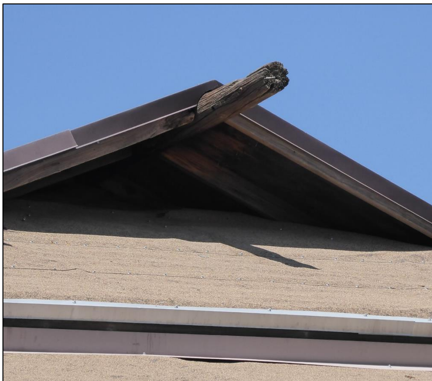
Figure 157. Brown aluminum fascia cladding on the upper layers of the roof of the José María Gil Adobe, 2021. (ERDC-CERL.)
