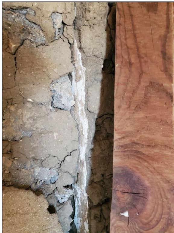
Figure 203. East room wall material. ( right , samples 16a and 17a) with smooth, white coating ( center , sample 12) against entry door jamb filler with gray bricks and mortar ( left , samples 9 and 10).
