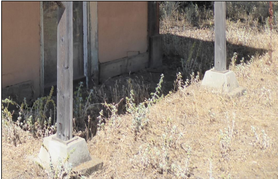
Figure 144. Concrete blocks supporting front wooden posts on the veranda of the cold storage building, 2021. (ERDC-CERL.)
