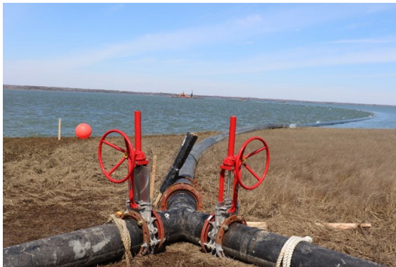
a. Viewing upstream of Y valve between valve and dredge (in background)
