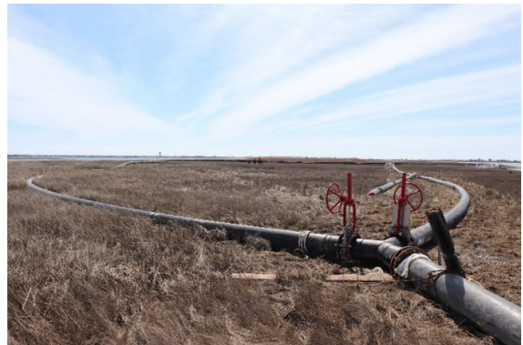
b. Downstream of Y valve between valve and placement areas
