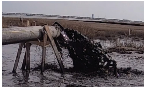
b. Sturgeon Island, New Jersey low-pressure (spreader plate) discharge Source: USACE–Philadelphia District
