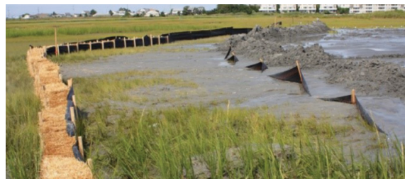
f. Straw bales, silt curtain, and earthen containment dike, Ring Island, New Jersey Source: Timothy Welp, ERDC
