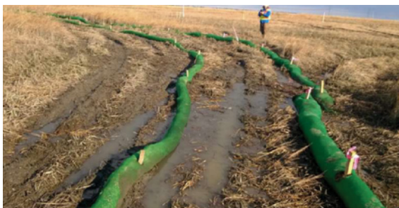
c. Filter Soxx, Fortescue, New Jersey Source: NJDOT
