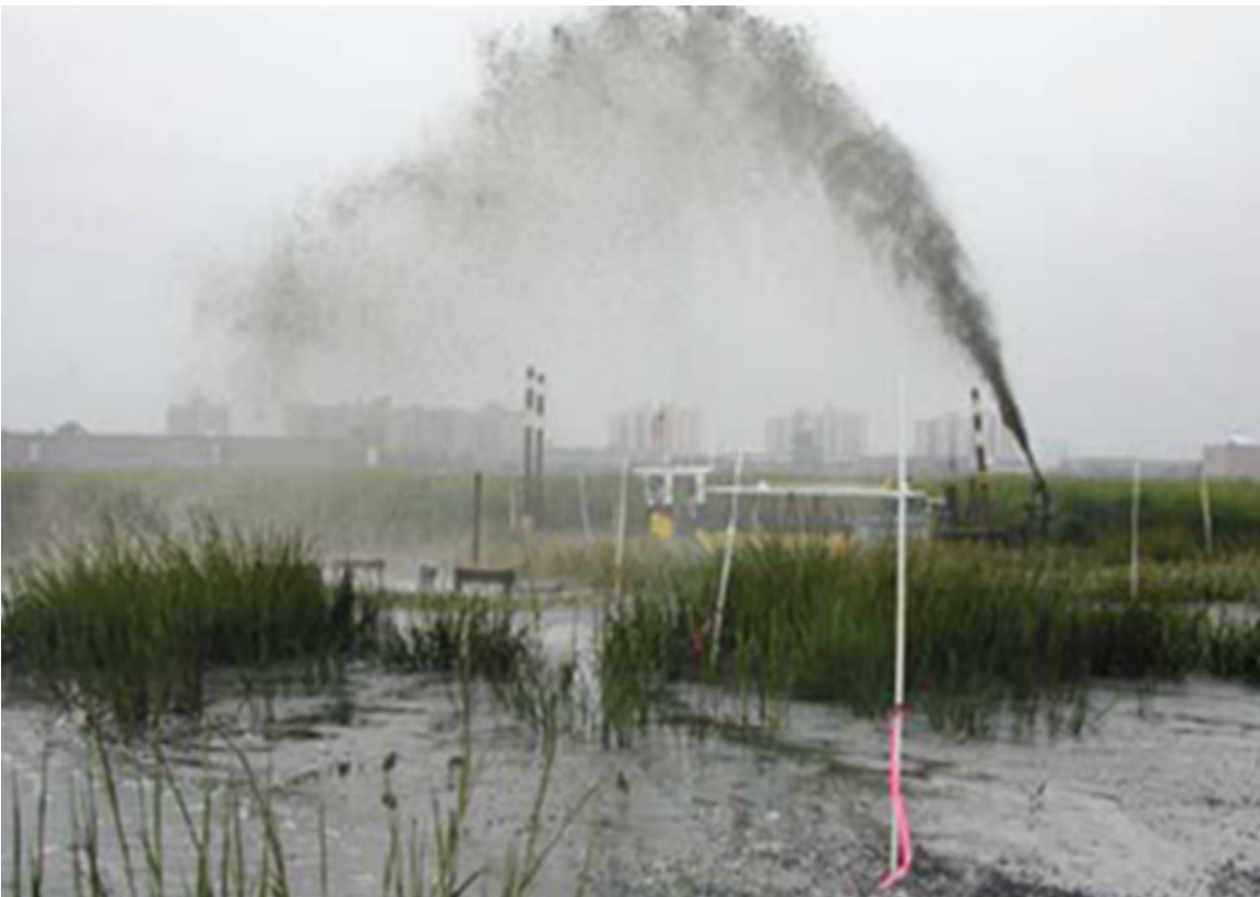
Figure 5.7. Modified Grade Stakes Used to Ascertain Attainment of DM Grade at First Blackwater NWR TLP Project
