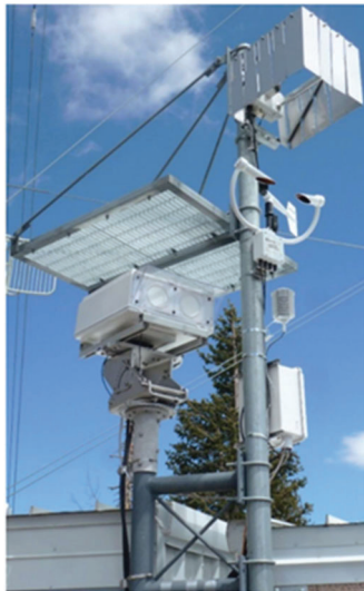
Figure 61. WTLE Transmitter, Weather Station, and Disdrometer
