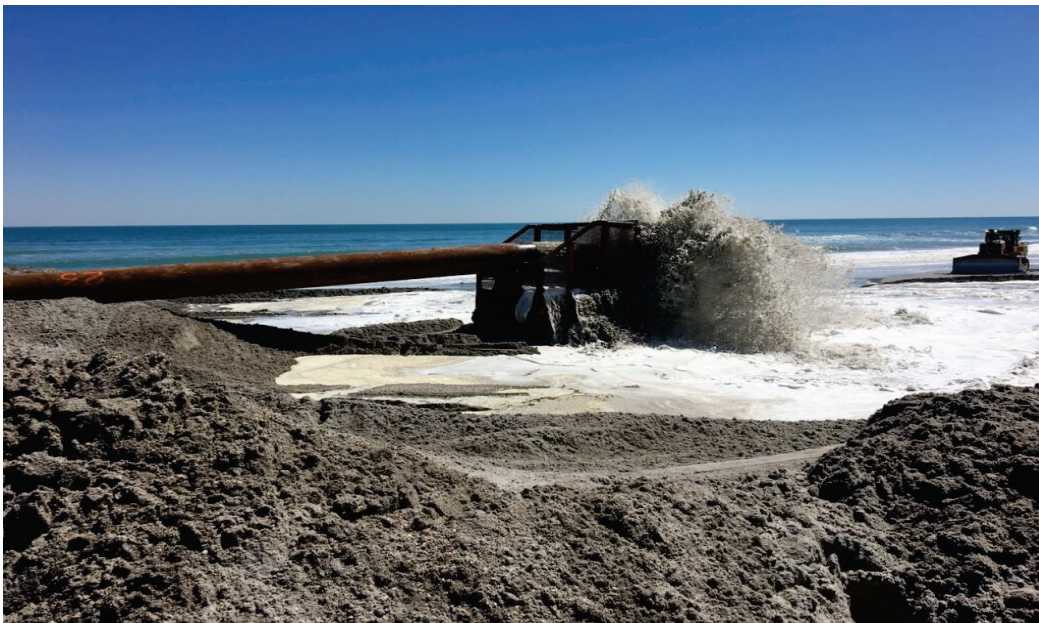
Figure 2-3. Segment of pipeline and other equipment on a beach during beach nourishment. Photo credit: USACE: New York District.
