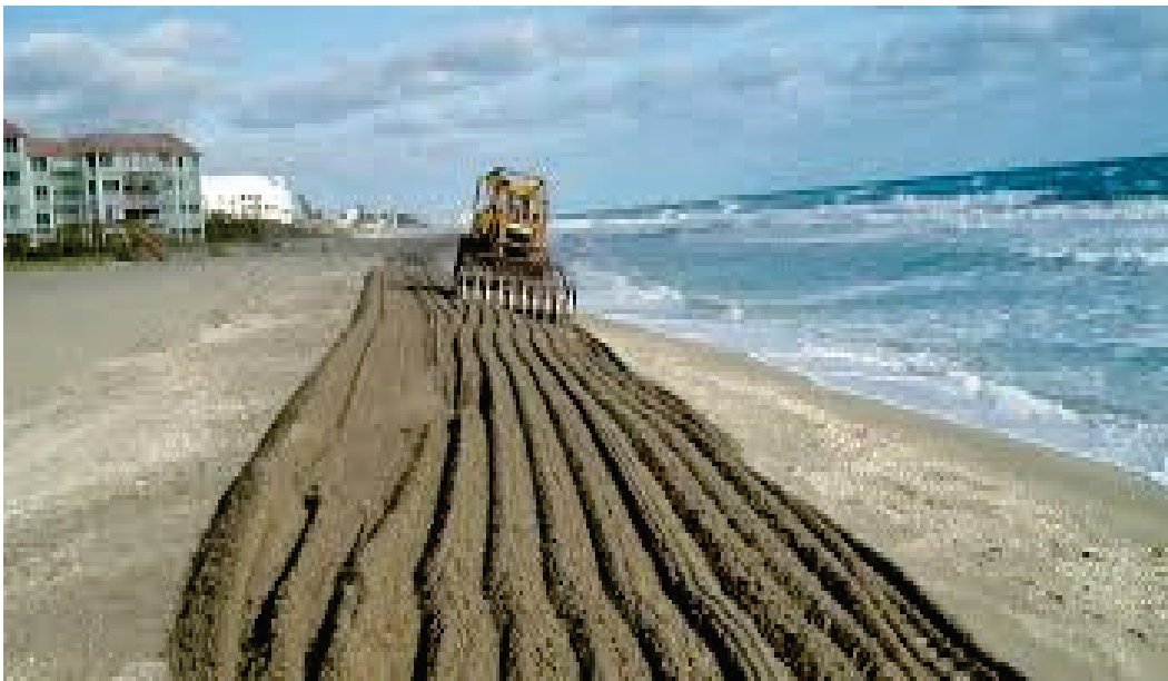
Figure 2-9. Tilling a newly renourished beach in Martin County, FL. Photo credit: USACE: Jacksonville District.
