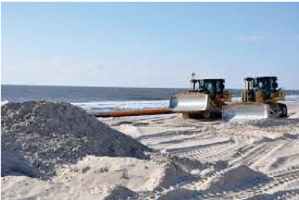
Figure 2-4. Bulldozers moving sand creating the new beach profile. Photo credit: USACE: New York District.
