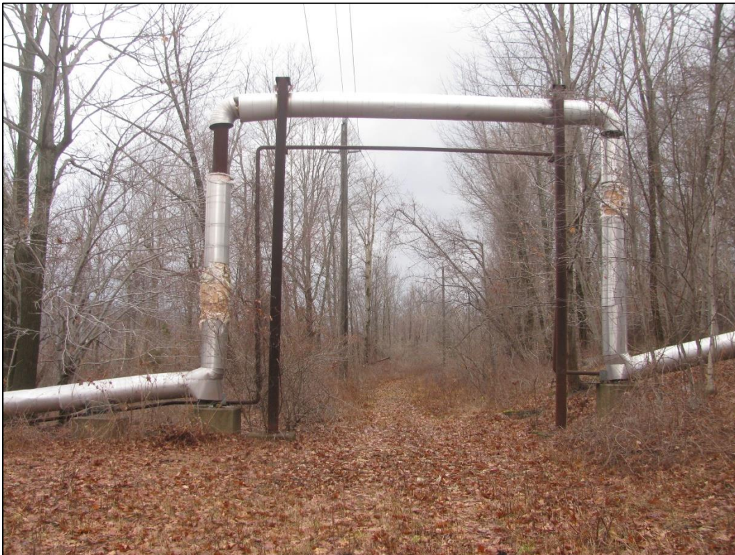
Figure 73. Looking northeast along the ROW near the former 1010 Area and just downhill from Building 3002.
