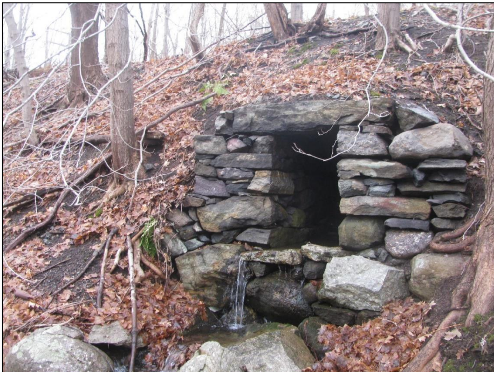
Figure 75. Looking west, just off the ROW, at a stone culvert in a section of woods in the 900 Area of the Arsenal.
