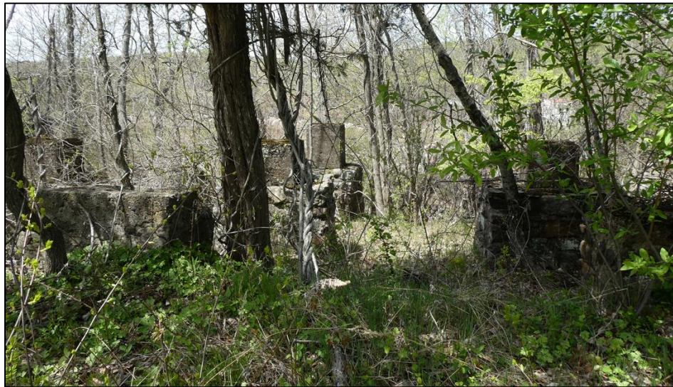
Figure 79. Piers to support the platform at the Factory Railroad Station (Site number: 28-Mr-345).
