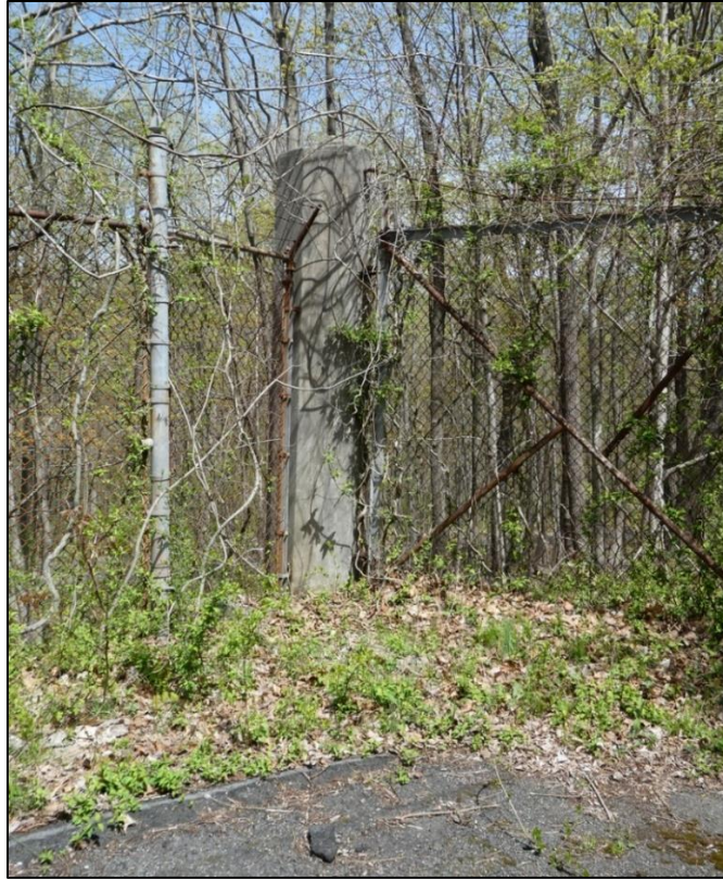
Figure 84. Concrete pylon and gate between Picatinny Arsenal and the former Navy Depot.
