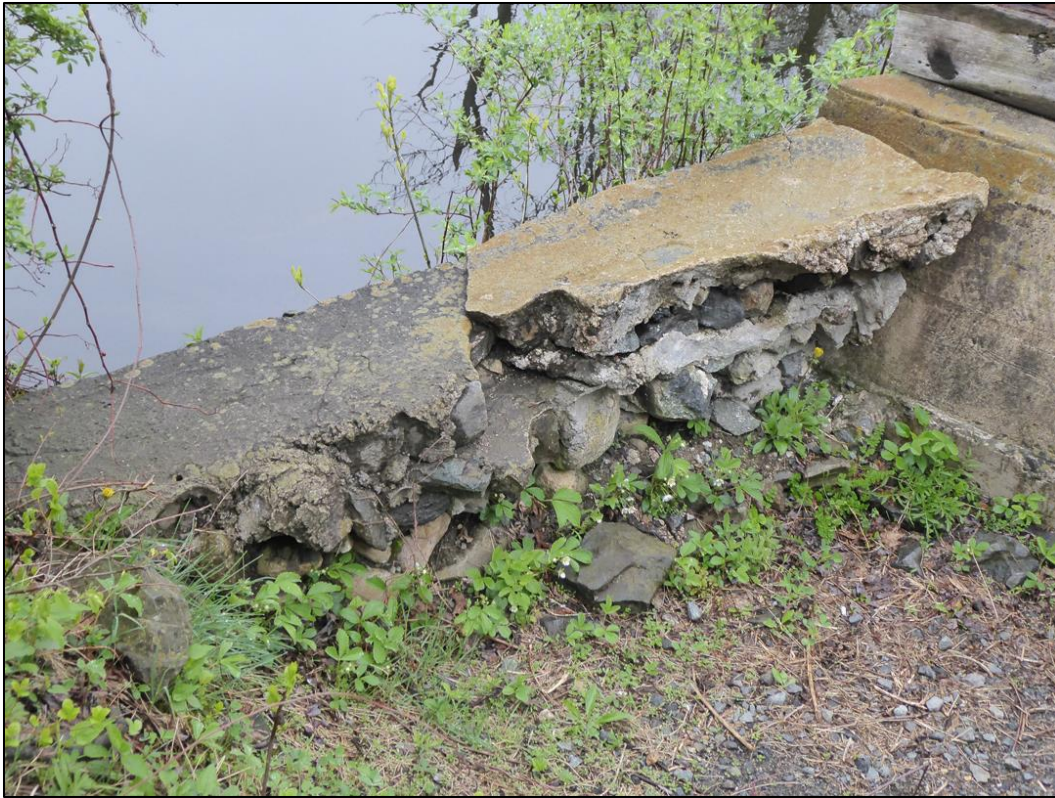
Figure 51. Looking northeast at detail of the west abutment on the Rockaway River bridge.
