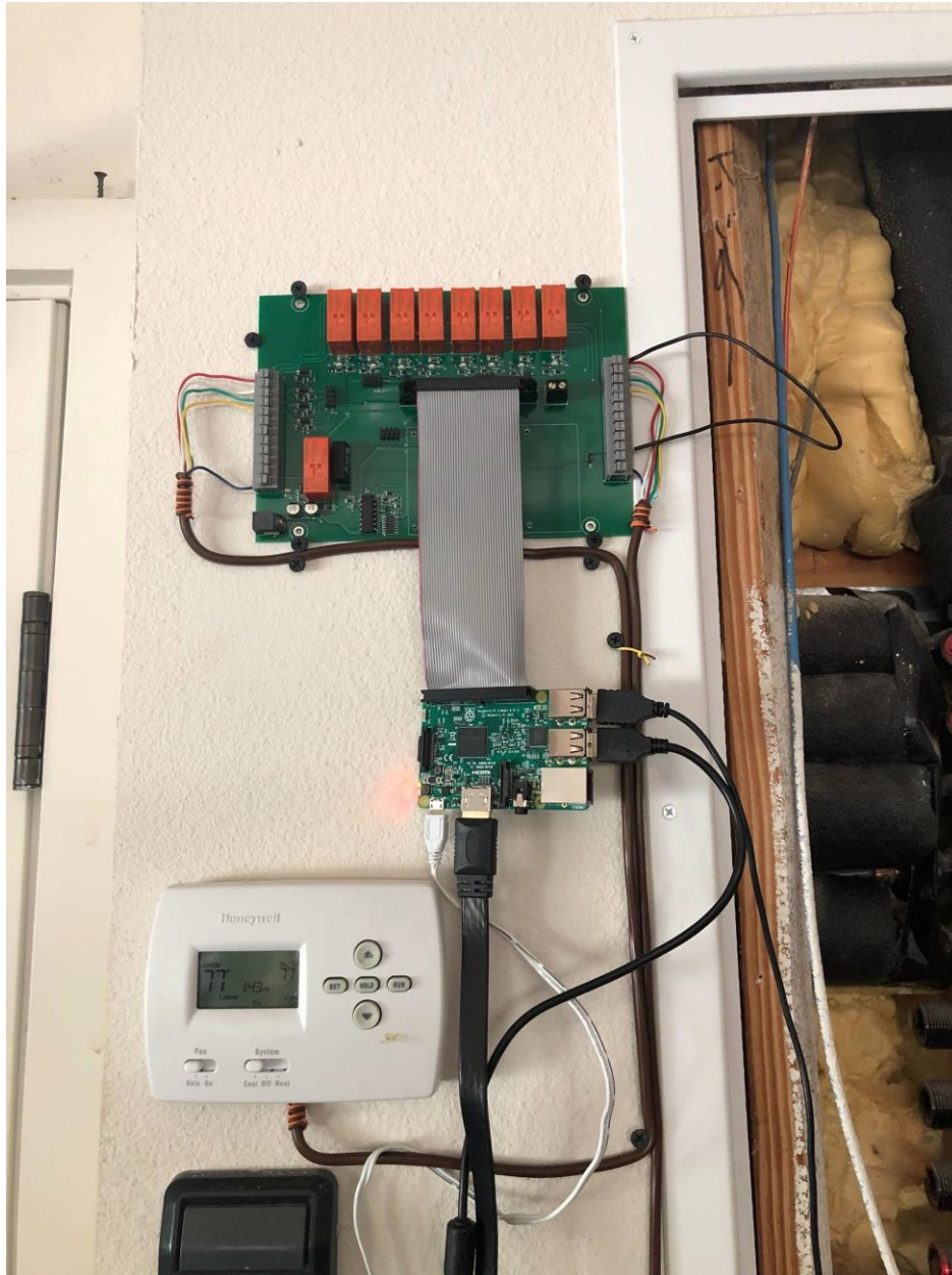
Photographic evidence of the HVAC test set at the PSI lab, including HVAC follower board, single board computer, and thermostat
