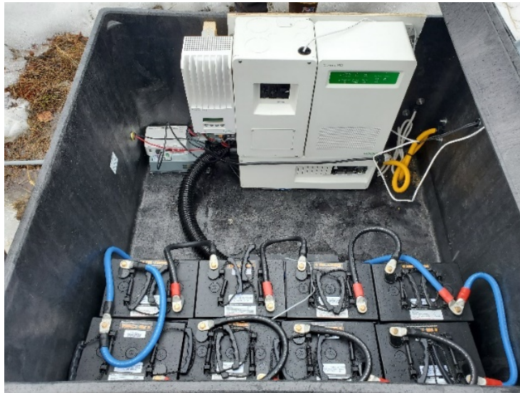
Figure 9. Conext ComBox communication and data monitoring system and the battery bank.
