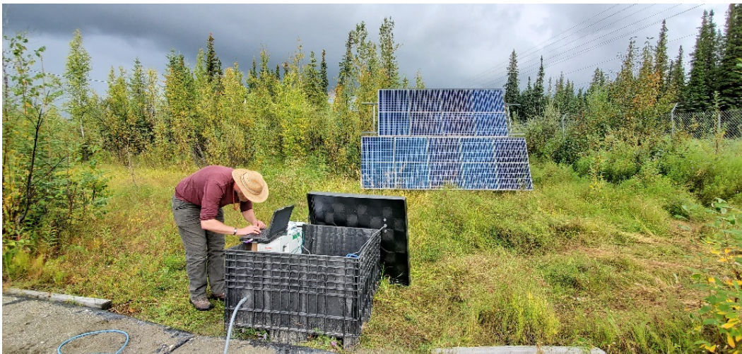
Figure 8. Solar panel array.
