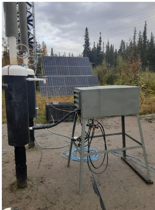
Figure 16. Refrigeration and solar panel installed at the frozen barrier field site.
