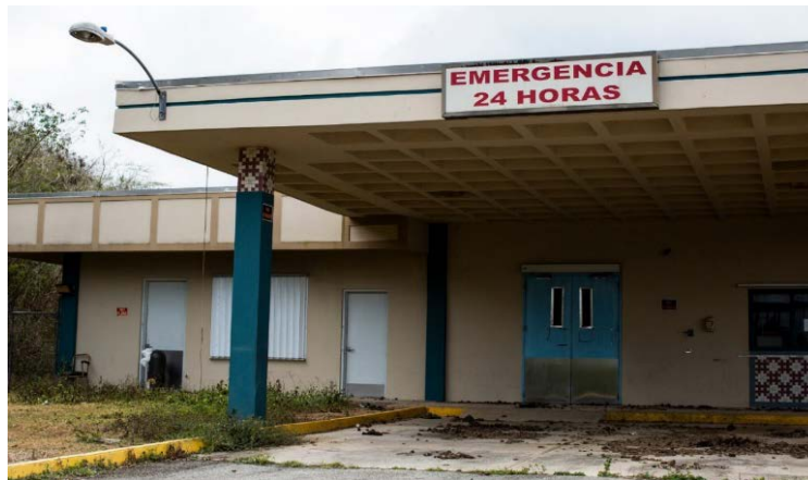
Figure 2. The Primary Hospital on the Island of Vieques, Shuttered and in Disrepair as of April 2019. 286
