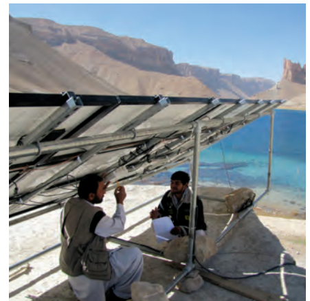
USAID is supporting electrification, here via photo-voltaic panels, in Afghanistan, through projects like ACEP, a program on which SIGAR published a financial audit report this quarter. (USAID photo)
