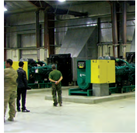
SIGAR's inspection found that generators, like those pictured, were improperly connected to a transformer, causing damage to two transformers. (SIGAR photo by Brian Flynn)
