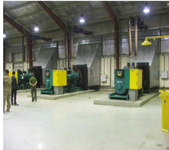
Photo 1 - Power Plant with Generators
