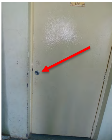
Photo 6 - Missing Door Lock
