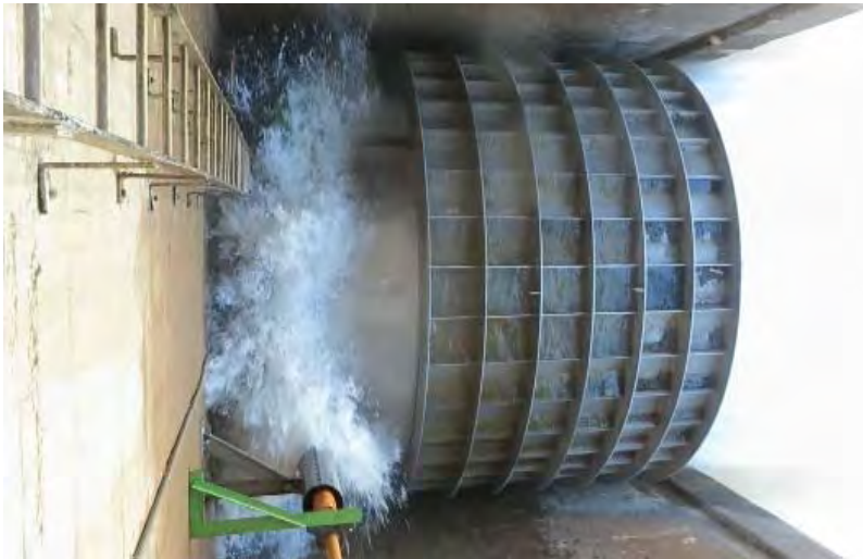
Photo 1 - New Cone Valve with Excessive Backsplash
