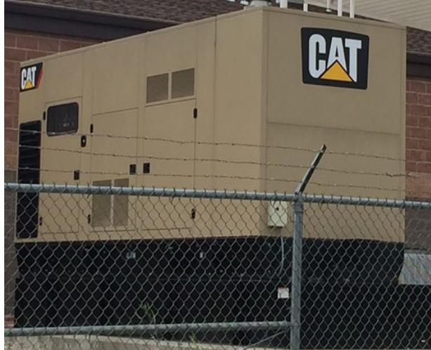
Figure 4. Building 2295 CAT Generator
