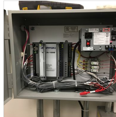
Allerton BMS controller
