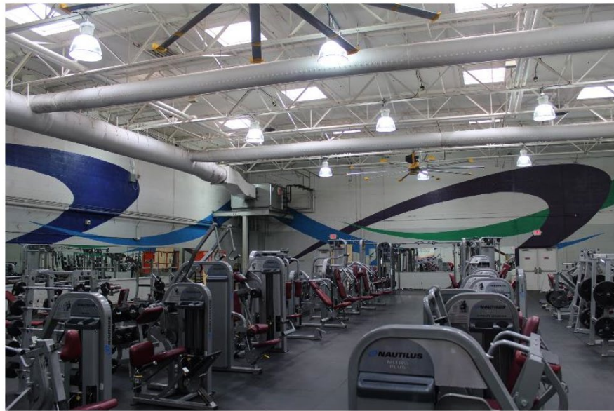
Completed weight room with 20 DC lights and 2 DC ceiling fans
