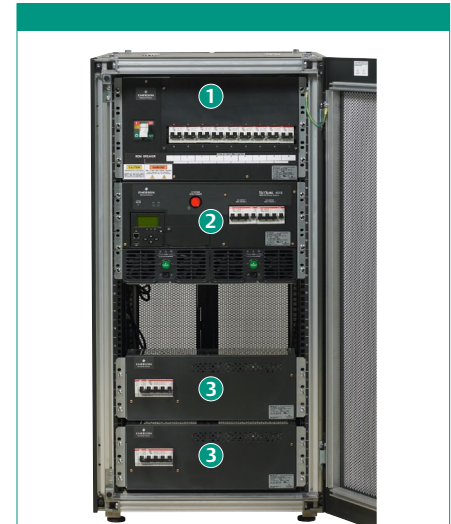
System Shown in a 24U Rack
