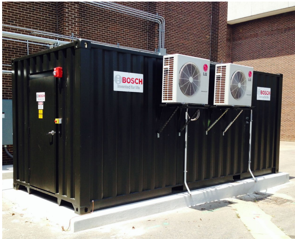
Figure 6. Battery Energy Storage System (BESS)
