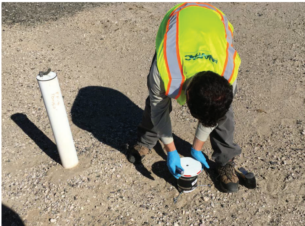
Tim Appleman installing Carbon Traps
