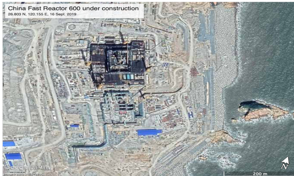
Figure 4.02: China's 600-MWe breeder reactor power plant, the CFR-600, under construction near Xiapu, China. The outline of the top of the cylindrical reactor containment vessel is visible in the center of the building. There are four cranes on yellow towers around the outside of the building plus one based inside the containment. Cooling water pipes are also visible. To the west of this site, excavation is underway to prepare for construction of a second CFR-600. 216
