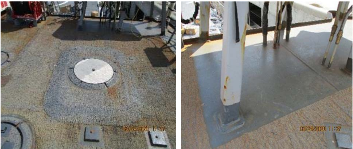
Figure 42 – Close-up of section 2 that received 100% SP6 Grit surface preparation of the deck and appendages
