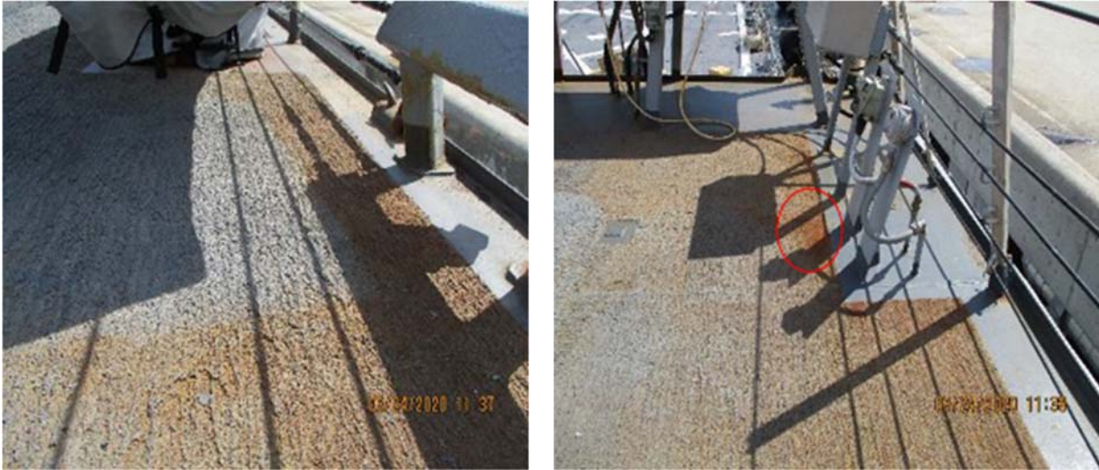
Figure 43 – Close-up of section 3 that received 20% SP10 Grit/80% UPHWJ surface preparation of the deck and power tool cleaning of deck edges and appendages not accessible by UHPWJ
