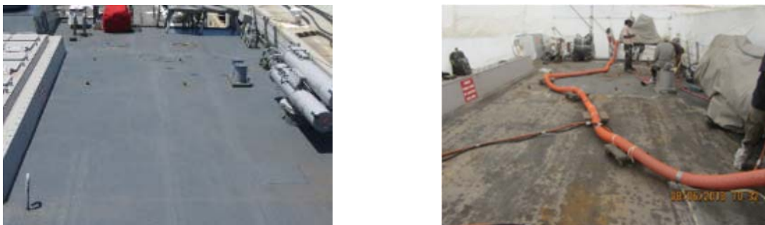
Figure 5 – Initial condition of DDG missile deck (left) and after UHPWJ (right) to remove nonskid coating
