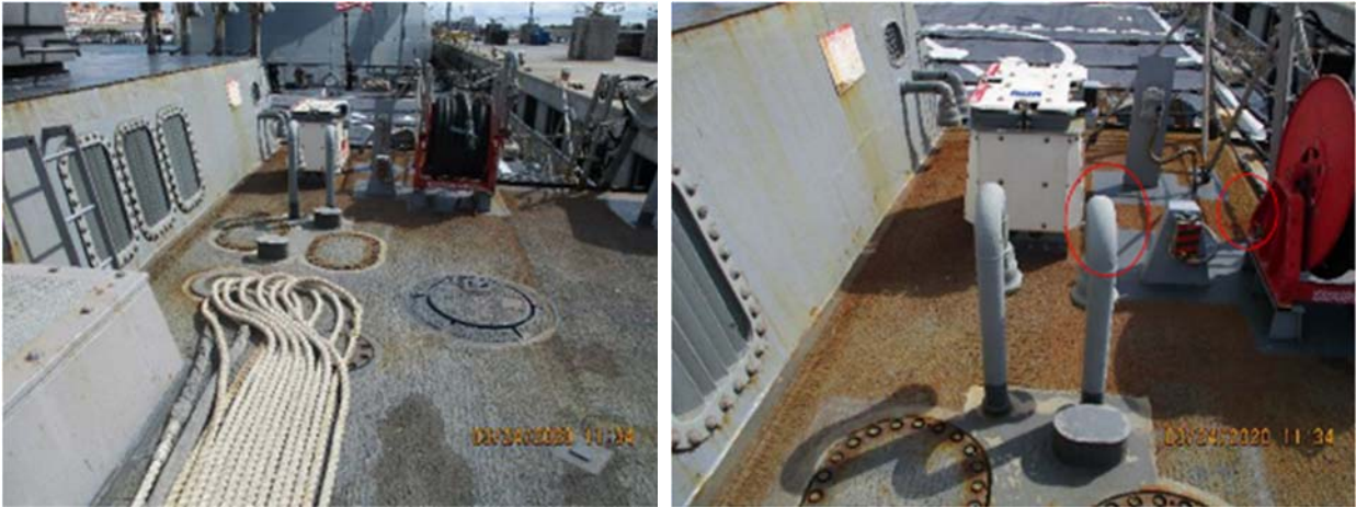
Figure 41 – Close-ups of section 1 that received 100% SP10 Grit surface preparation of the deck and appendages
