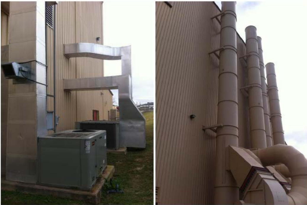
Figure 4-4. B-59; Left: Packaged Units Supply many of the Office Spaces, Right: Exhaust Fans
