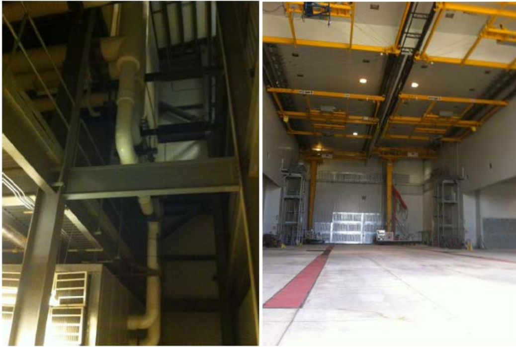
Figure 4-3. B-59; Left: Large Multi-floor Air Handling Unit Systems are used to condition the air to the Paint/Depaint Space, Right: One of Two Paint/Depaint Spaces
