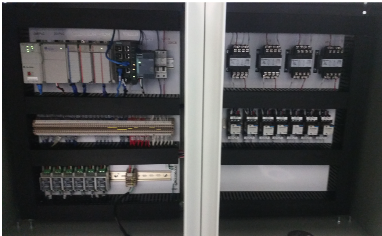
Figure 5: Cabinet-view of the power transmission and distribution simulator
