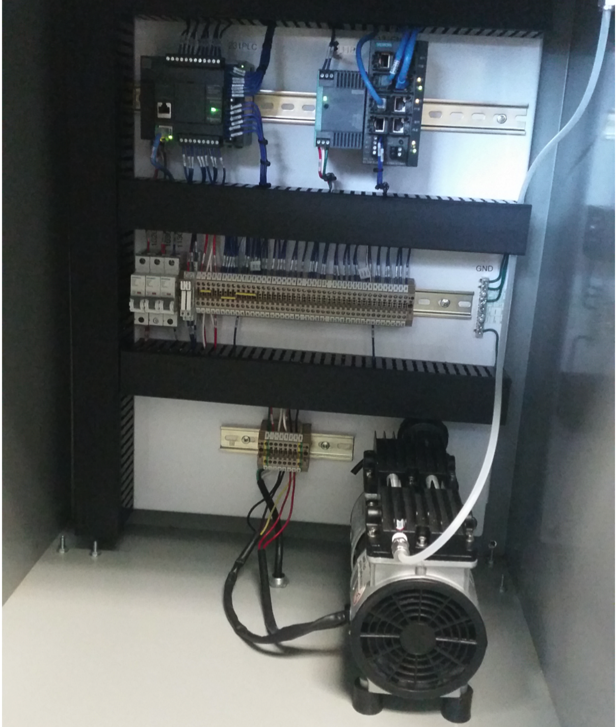
Figure 3: Cabinet-view of the gas pipeline simulator
