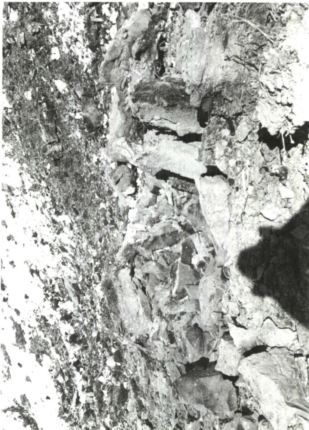
Fig 31 Shot #15: Result of 30 lb of liquid explosive in a 6" dia by 10' deep-bored shot hole
