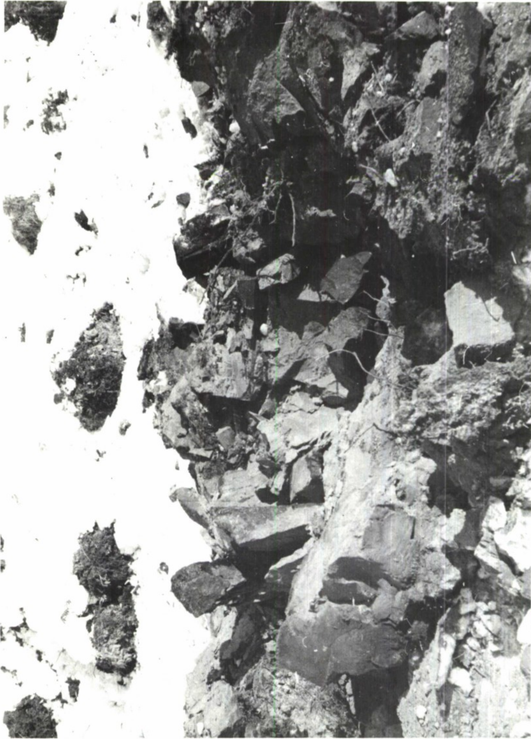
Fig 30 Shot #14: Result of 16 lb of liquid explosive in a 4" dia by 9' deep-bored shot hole
