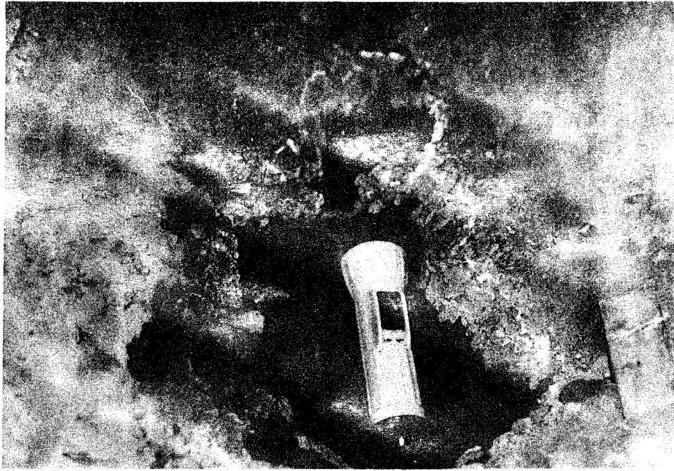
Figure 47. Hole through conduit at invert, Mulberry Dam
