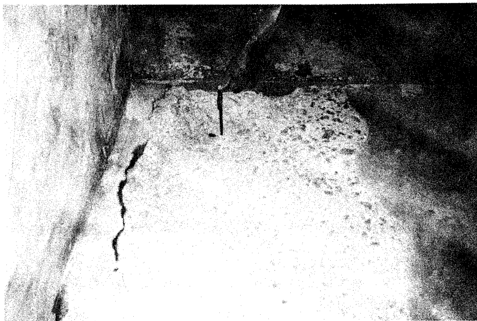
Figure 40. Erosion damage, Isabella Dam, December 1983
