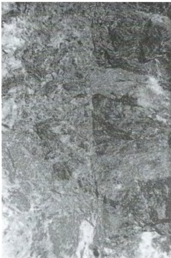
Figure 7.5: Photograph of the tunnel wall crossing a cut-off screen, after the 2 kt explosion. Broken rocks on the left filled the screen (gap) as a result of the explosion, while the rocks on the right are only slightly deformed. The boundary between the zones is the opposite wall of the screen (the wall that is further away from the explosion source).
