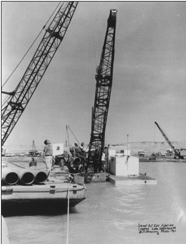
Figure 2 - In 1961, cranes and barges worked offshore to help lay the Signal Oil pipeline across the bottom of Lake Sakakawea (North Dakota State University, 2011).
