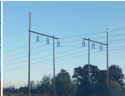
(c) H-frame transmission towers.
