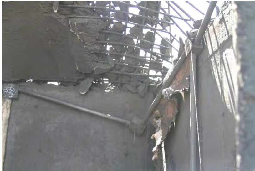
FIGURE V-8. West Wall (Right), South Wall (Lower Left), Roof (Upper Left), and Rebar That Had Attached Roof to West Wall (Test 4).
