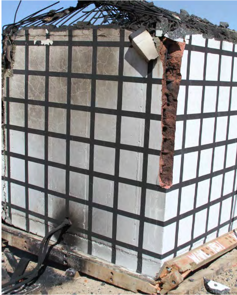
FIGURE V-27. West Wall, South Wall, and Damaged Roof (Test 4).
