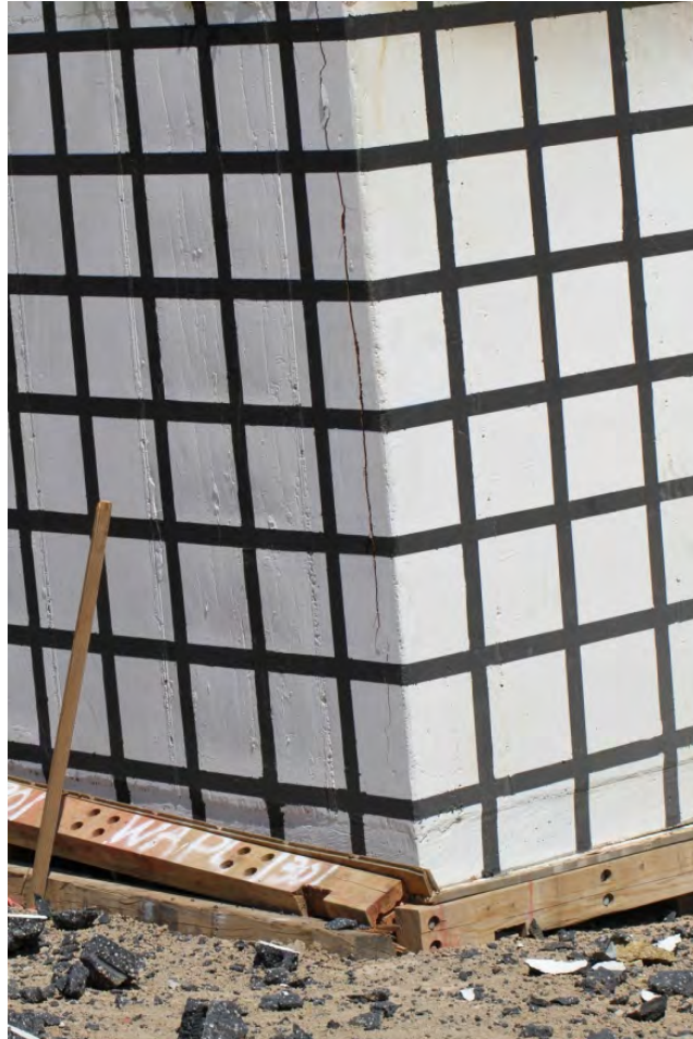
FIGURE V-32. South Wall (Left)/East Wall (Right) Corner With Crack in South Wall (Test 4).
