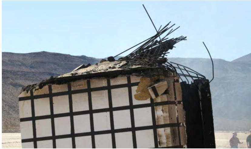
FIGURE V-33. East Wall/North Wall Roof Junction at End of Test 4.
