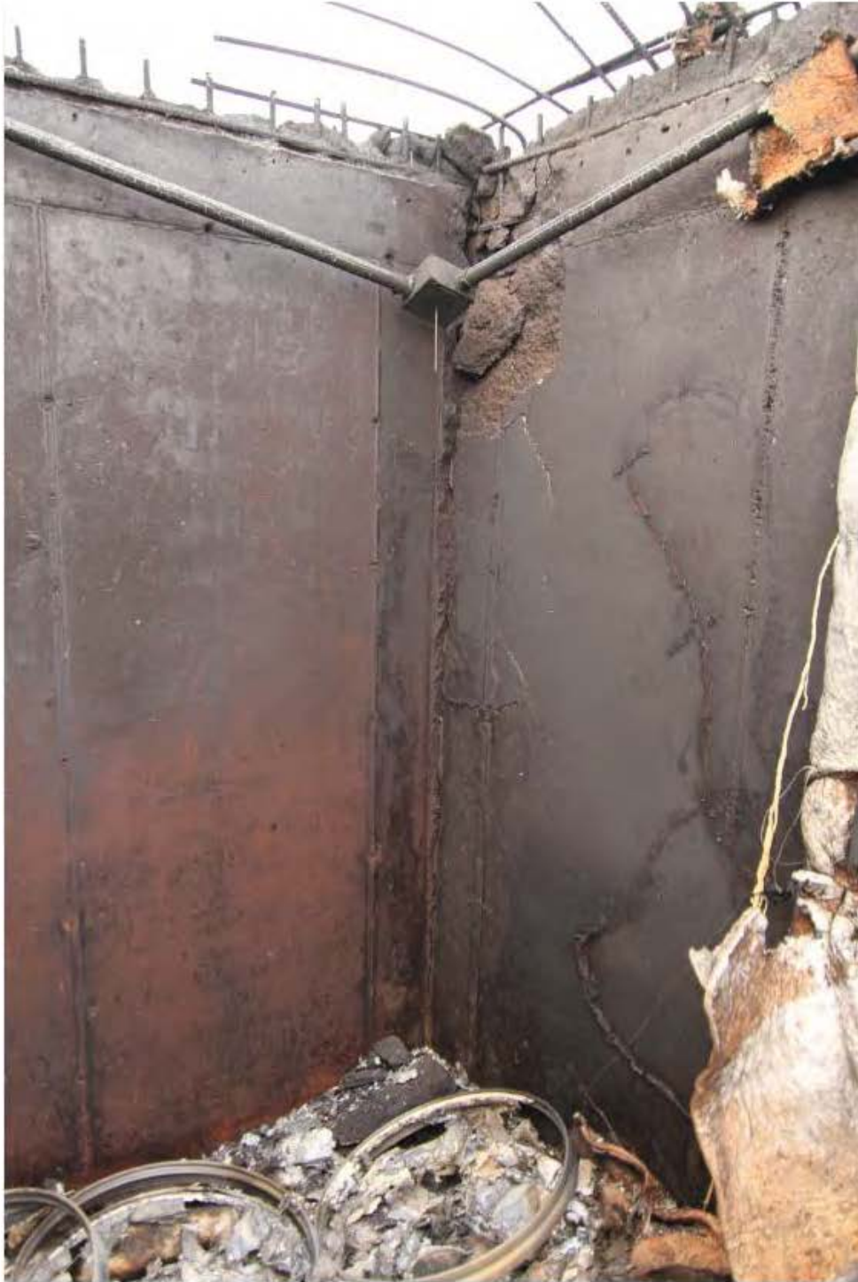
FIGURE III-12. Intersection of West Wall (Right) and South Wall (Left) (Test 2).
