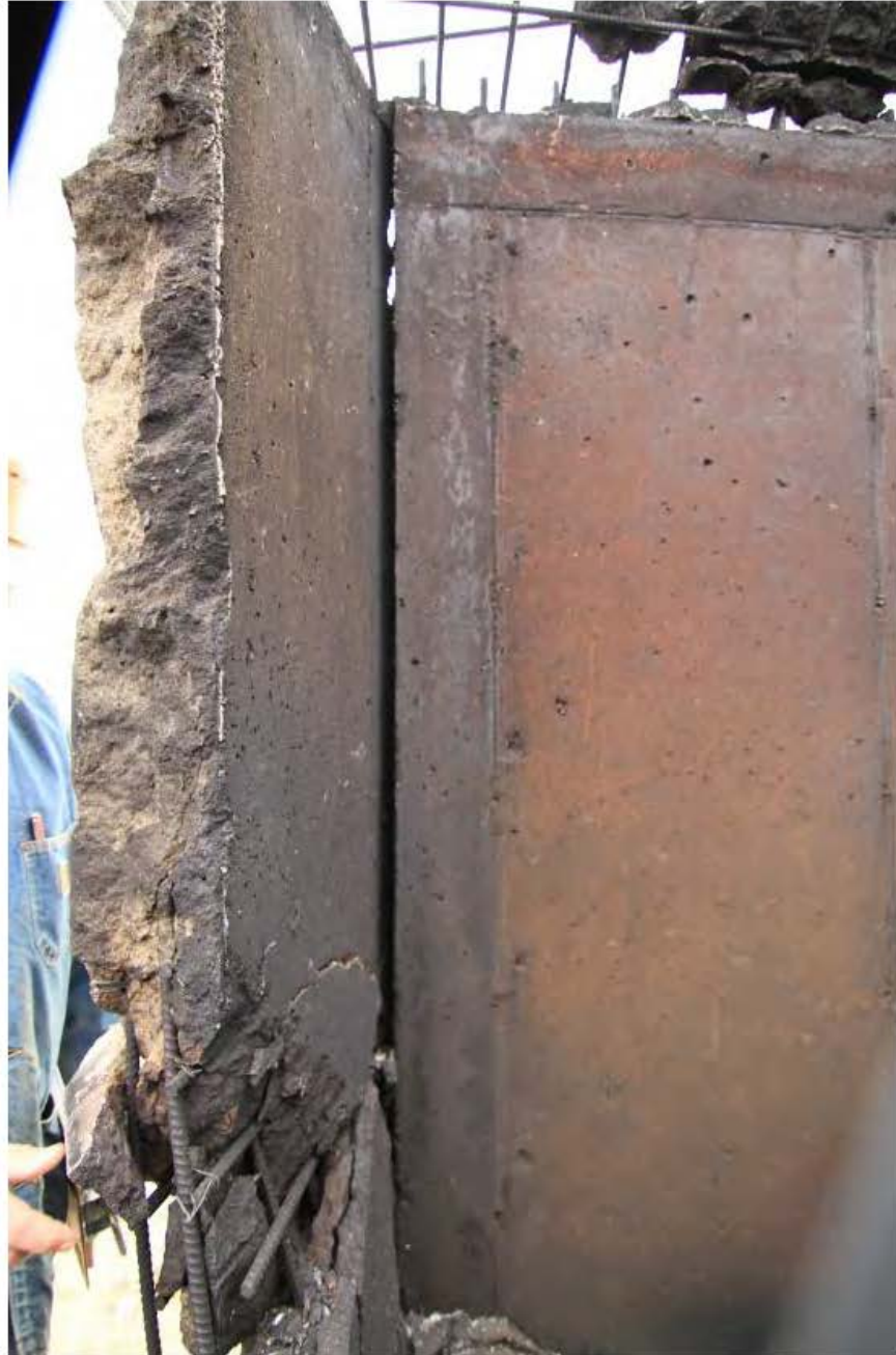
FIGURE III-14. Intersection of Eastern Wall and What Was Left of Northern Wall (Test 2).
