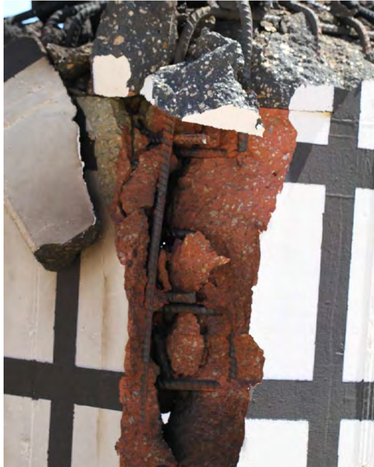
FIGURE V-28. Close-Up Photograph Showing Damage at Roof, South Wall (Red), West Wall (Green Attached Fragment) (Test 4).
