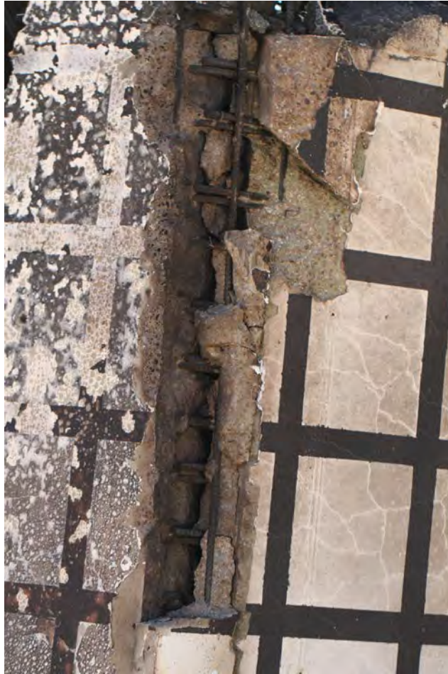
FIGURE V-31. Damage at North Wall (Left)/ West Wall (Right) Junction at End of Test 4.
