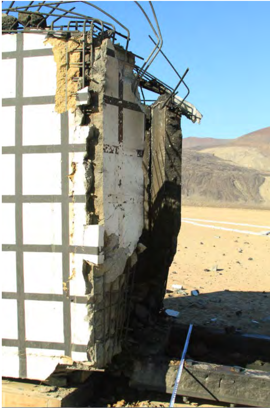
FIGURE III-21. Two Parts of North Wall Bowed Out and Door Frame and Plate Resting on Ground in Front (Test 2). This figure also shows the damage to the east wall and north wall junction.
