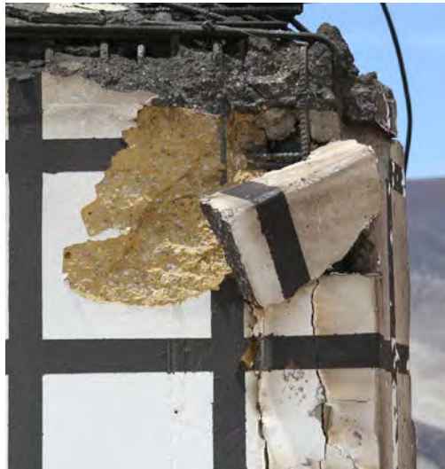
FIGURE V-34. Close-Up of East Wall Roof/North Wall Junction (Test 4).
