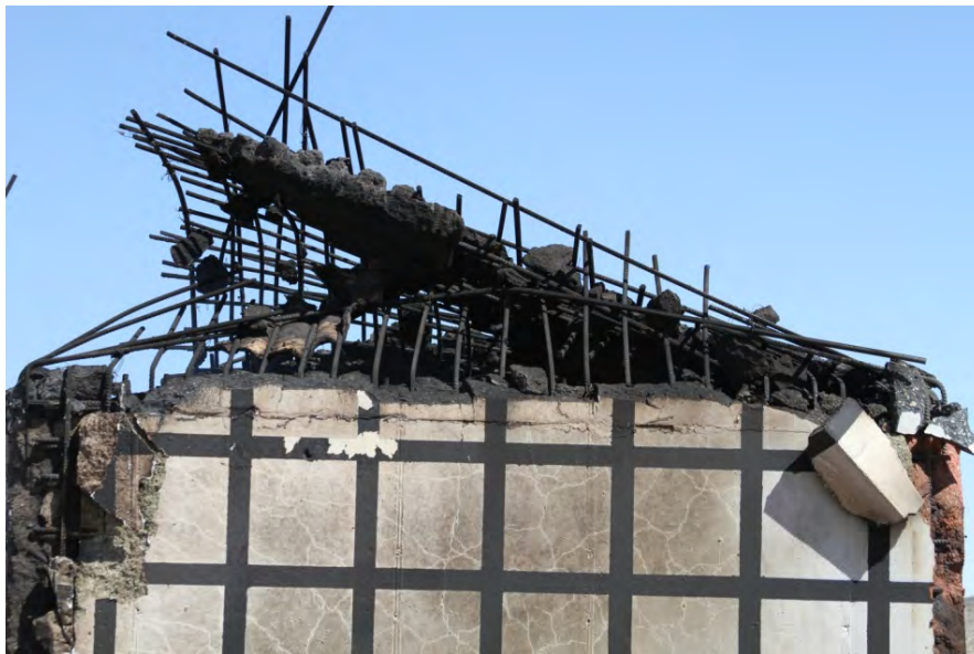
FIGURE V-30. West Wall and Damaged Roof After Test 4.
