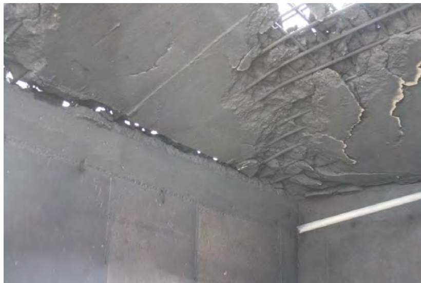
FIGURE V-9. East Wall (Lower Left), South Wall (Lower Right With Conduit) and Roof (Upper Portion of Figure) (Test 4).
