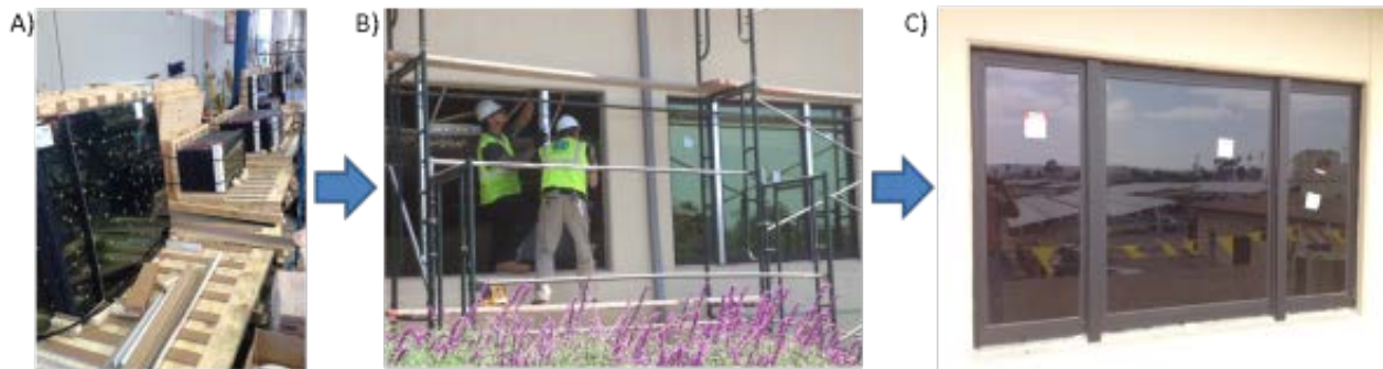
Figure 5. A) View dynamic glass IGUs received at Miramar. B) Construction crew removing old window frames. C) Final installed dynamic windows.
