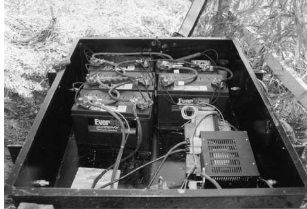
Figure 4. Batteries and regulator/charger
