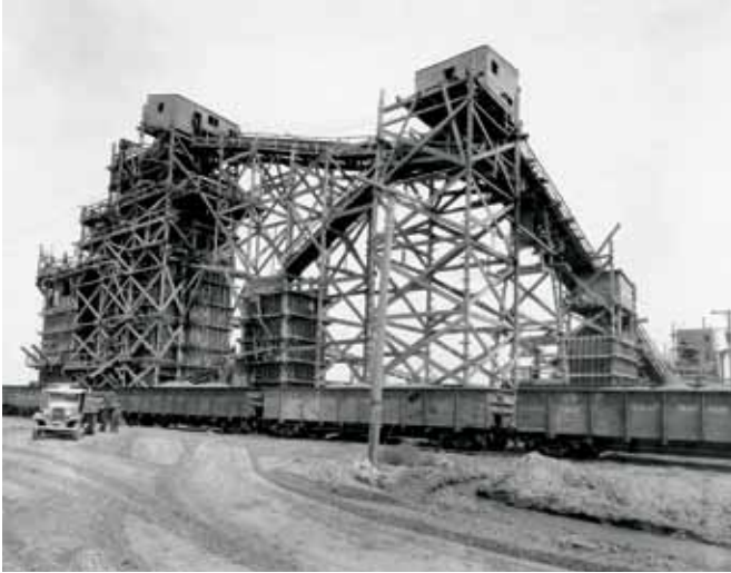
Above: The huge gravel plant was capable of producing 100 train carloads of screened and washed gravel each day.
