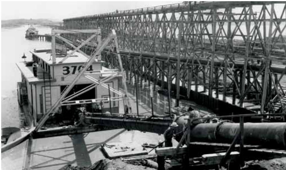
Workers connecting the newly relocated pump boat 3704 back into the pipeline. The pump boat is in the core pool, on what is now the top of the dam. Timber cut in the area that would become the reservoir was used to build the support trestles for the 28-inch pipeline.
