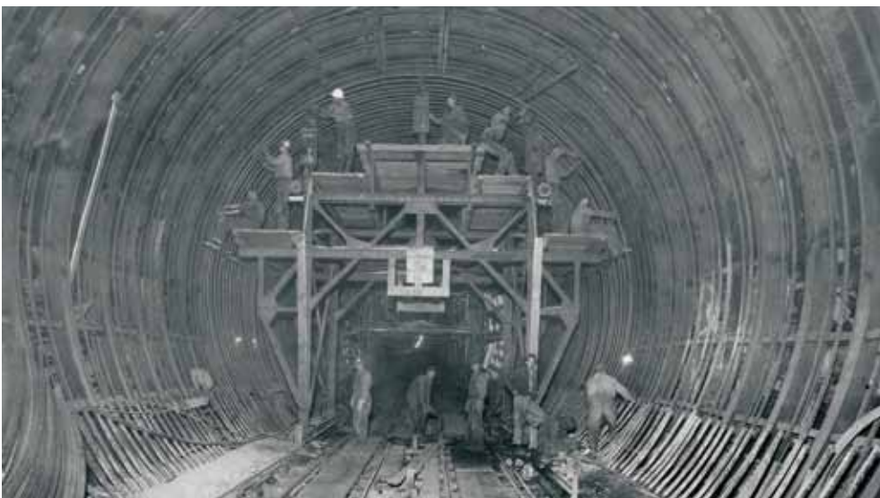
Tunnel # 1 under construction in 1936. Workers place steel reinforcing for sidewall and arch of the tunnel. This tunnel would be steel lined, unlike the other three tunnels, in preparation of a powerhouse to be built at the outlet of the tunnel.
