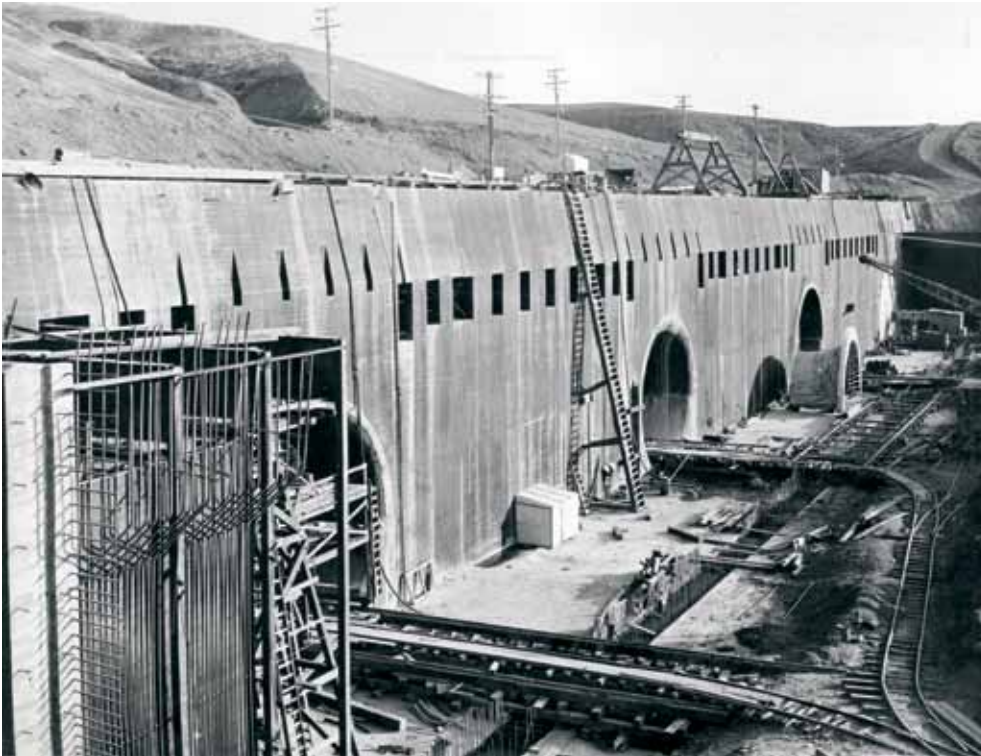
The tunnel intakes under construction in 1936. These intakes are now submerged under 200 feet of water at the bottom of Fort Peck Lake.
