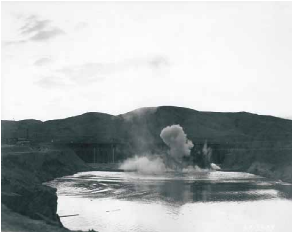
June 24, 1937, at 4:20 a.m. the dike in front of the tunnel intake portals was blasted allowing water to flow into the tunnels for the first time. The final work on the tunnels had only been completed the night before.
