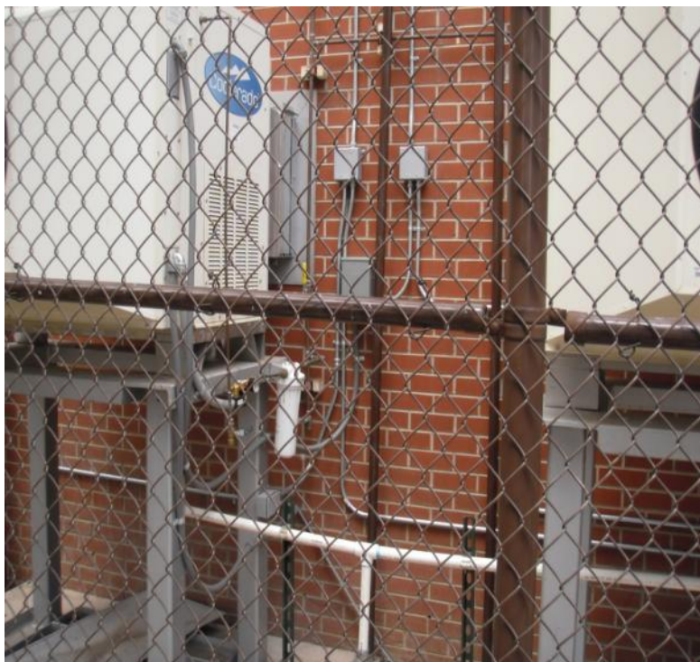
Figure 9. Coolerado drain water piping.
