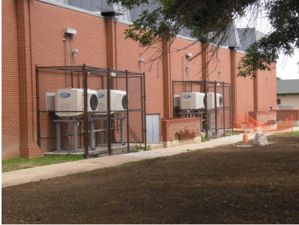
Figure 10. Coolerado units and manhole over water storage tank. (Source: Jesse Dean, NREL)
