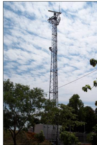
Indonesia - Communication Radar Tower
