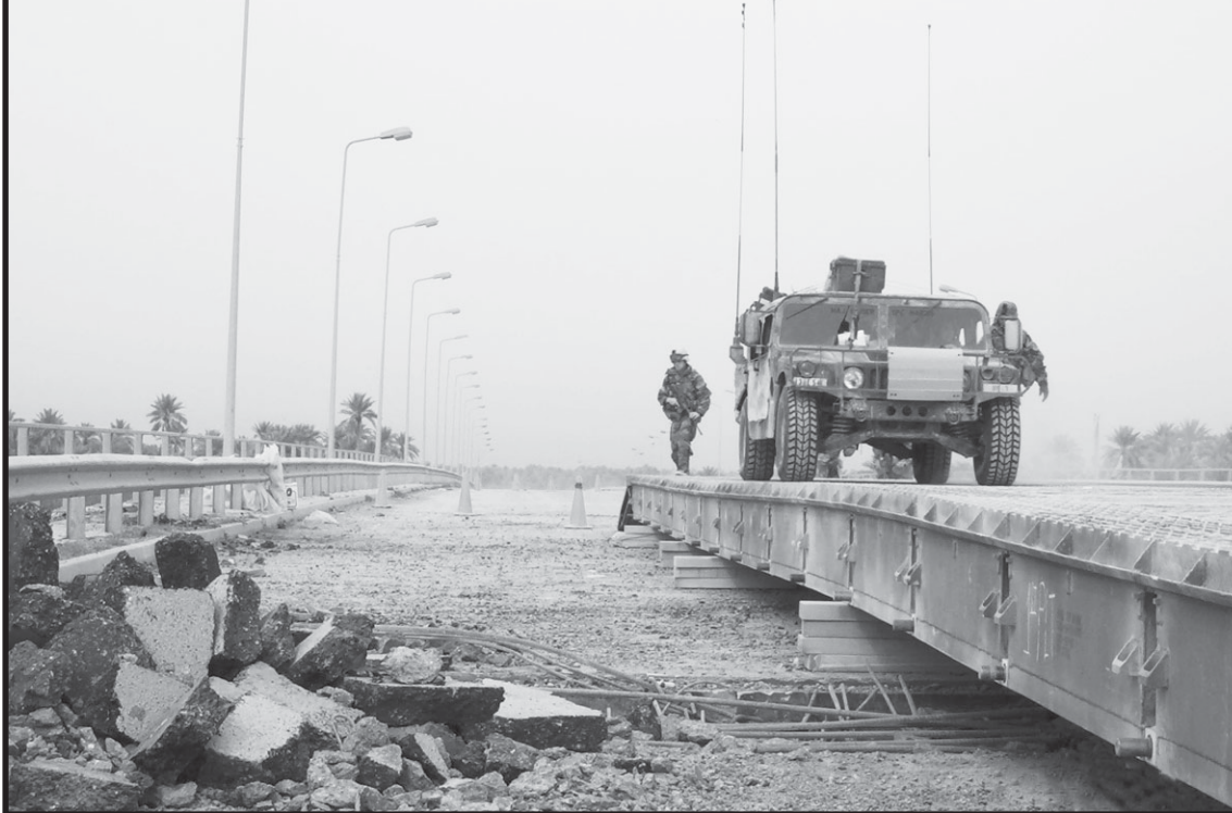
A HMMWV crosses a newly completed medium girder bridge at Objective Peach.
