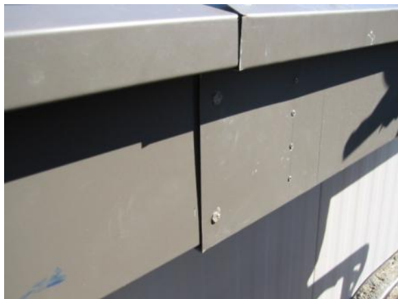
RE-H-4: Rake flashing has open joint or butt joints.
