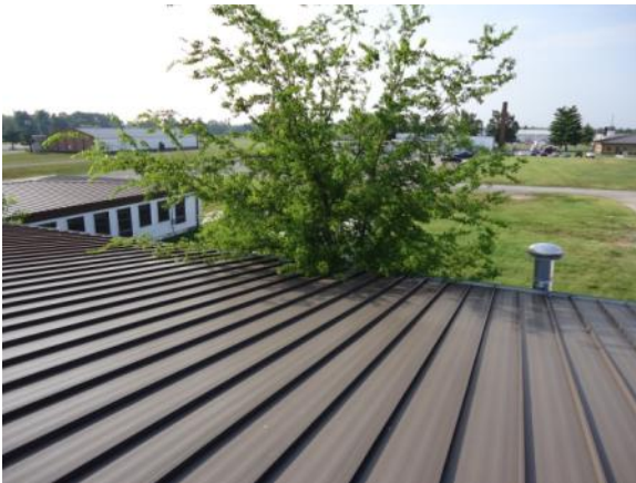
DV-M-2: Evidence of tree branches making contact with the roofing system.
