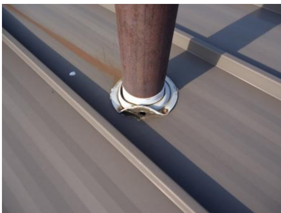
FB-H-2: Flexible boot flashing has deformed securement ring, allowing water to penetrate the roofing system.
