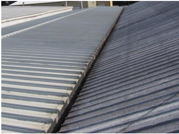
IG-L-1: Interior gutter is lined with elastomeric membrane or coating and appears to be watertight.
