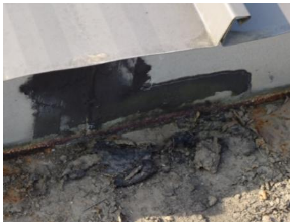
IG-H-1: Interior gutter is not lined with elastomeric membrane or coating and has holes, splits or open joints.
