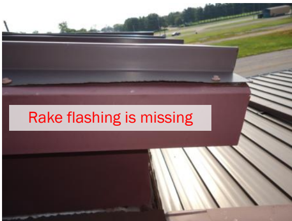
RE-H-2: Rake flashing is loose, displaced or missing, allowing water to penetrate the roofing system and/or compromising panel securement.
