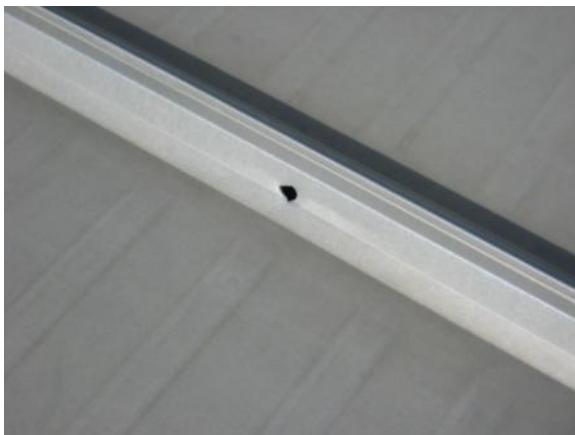
DP-H-1: For panel system that has mechanically interlocked seams, panel has holes, splits, or tears that require localized repairs.
