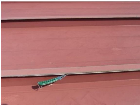
MS-H-1: Seam is open or allowing water to penetrate the roofing system; or seam is disengaged.
