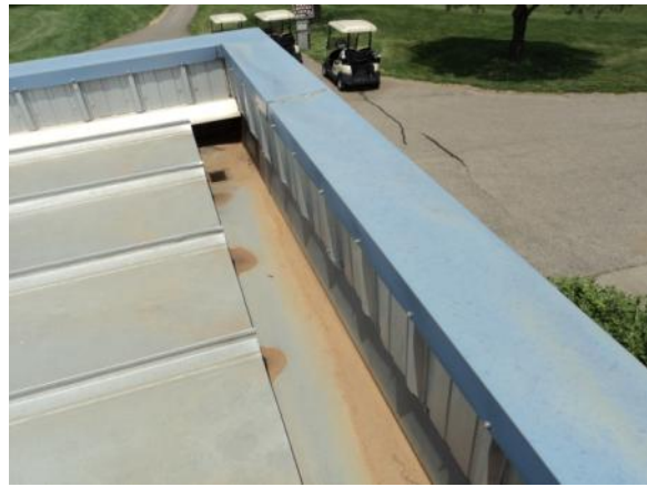
IG-M-1: Interior gutter is not lined with elastomeric membrane or coating and appears to be watertight.
