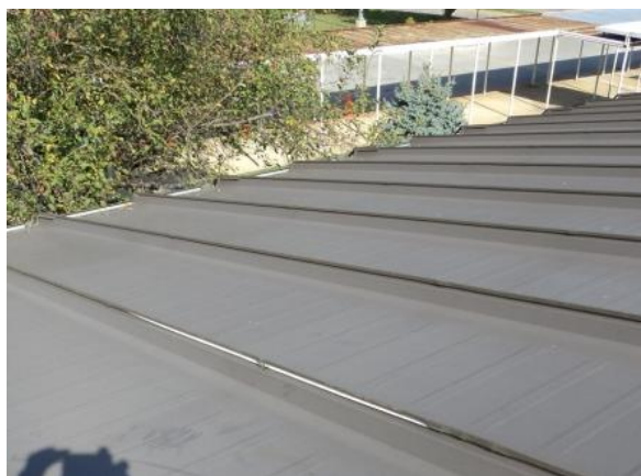
MS-H-1: Seam is open or allowing water to penetrate the roofing system; or seam is disengaged.
