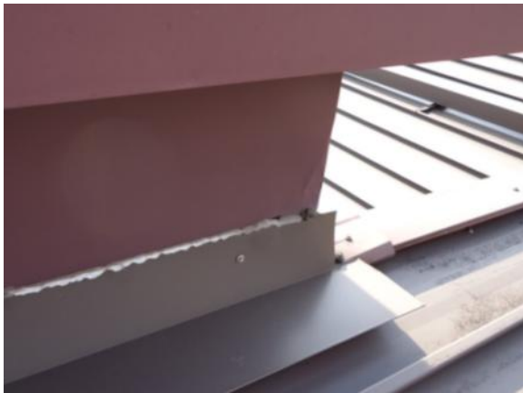
AF-H-6: Sealant at reglet, top of counterflashing, or sealed joint is missing or no longer functioning.
