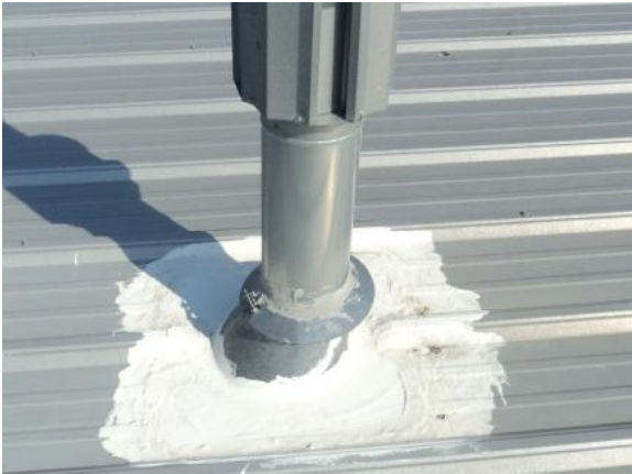
FR-L-1: Flashing patch appears to be performing a waterproofing function and appears to be watertight and does not require a more permanent repair.
