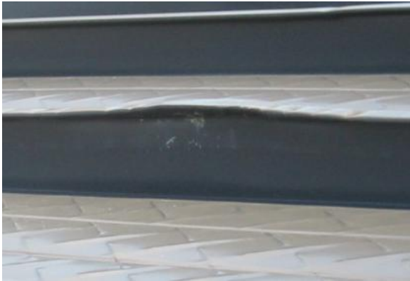
MS-L-1: Seam is deformed or flattened but appears to be watertight.
