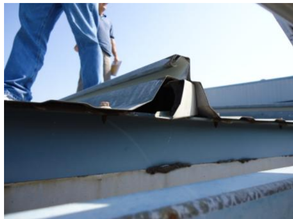
PC-H-1: Non-metal panel closure is deformed, misaligned, damaged or missing; allowing water to penetrate the roofing system.
