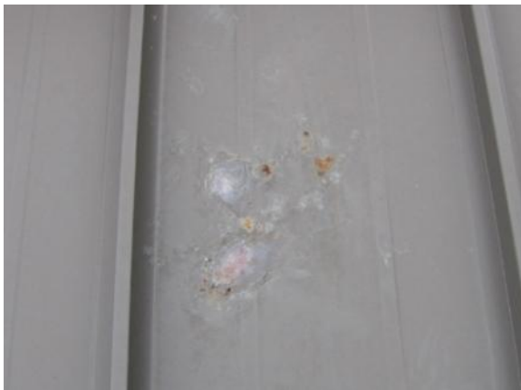
SD-H-1: For panel system that has mechanically interlocked seams, panel has corrosion holes that require localized repair .
