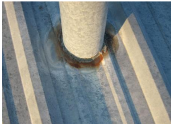
FB-H-1: Flexible boot is missing or has holes; or flexible boot flashing interferes with a panel seam and is allowing water to penetrate the system.
