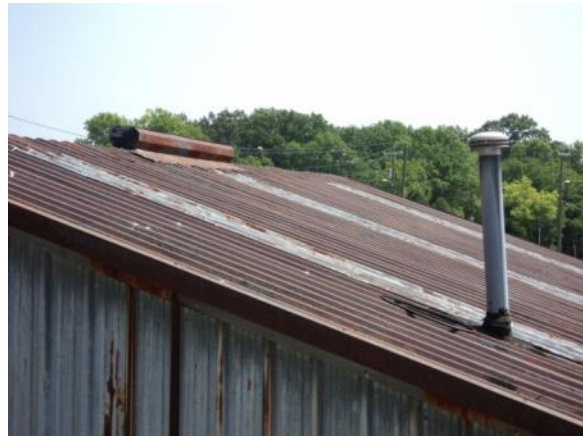
SW-H-1: Base metal exhibits corrosion over the entire roof section requiring a roof replacement.
