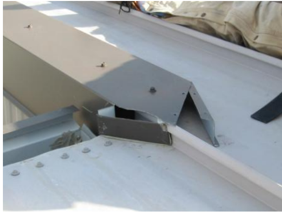
RE-H-2: Rake flashing is loose, displaced, or missing, allowing water to penetrate the roofing system and/or compromising panel securement.
