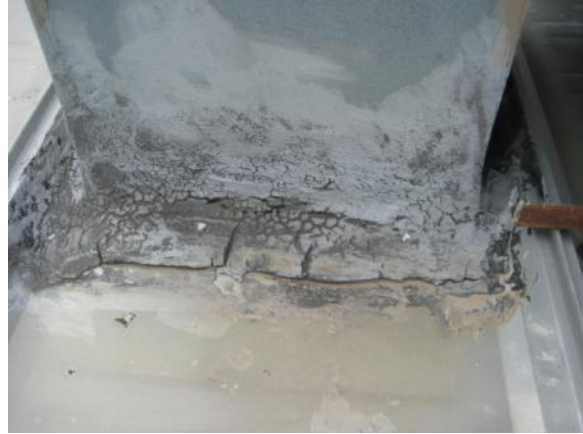
FR-H-1: Flashing patch is allowing water to penetrate the roofing system.
