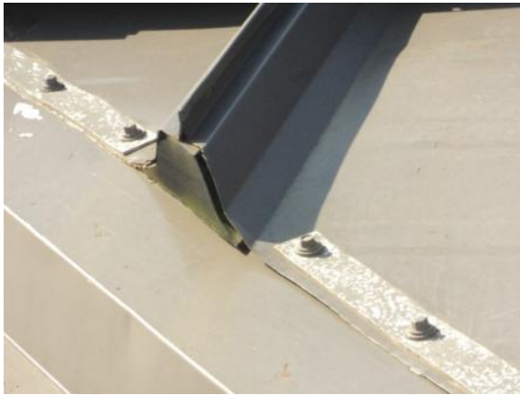
PC-M-1: Panel closure is misaligned but appears to be watertight.
