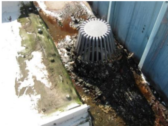
IG-H-3: Interior gutter or drain is clogged.
