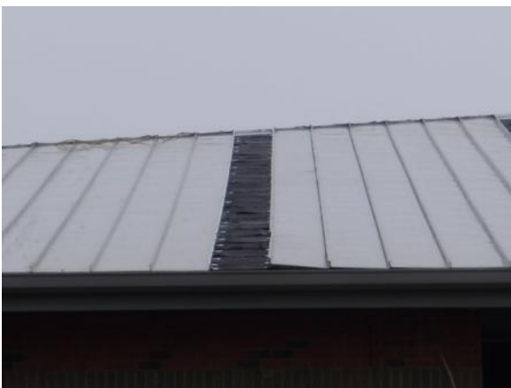
DL-H-2: Panel is missing and requires replacement.
