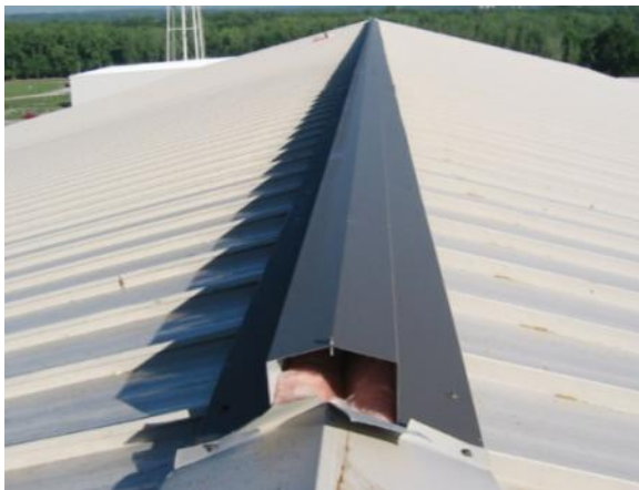
CP-H-3: Ridge or hip cap flashing is missing.
