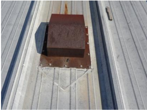
FM-M-1: Flashing flange on upslope side is mounted on top of panel, bucking water, but appears to be water-tight.
