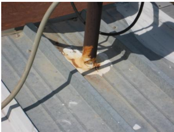
FB-H-1: Flexible boot is missing or has holes; or flexible boot flashing interferes with a panel seam and is allowing water to penetrate the system.
