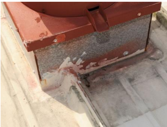
FR-M-1: Flashing patch, which appears to be performing a waterproofing function, appears to be watertight but requires a more permanent repair.
