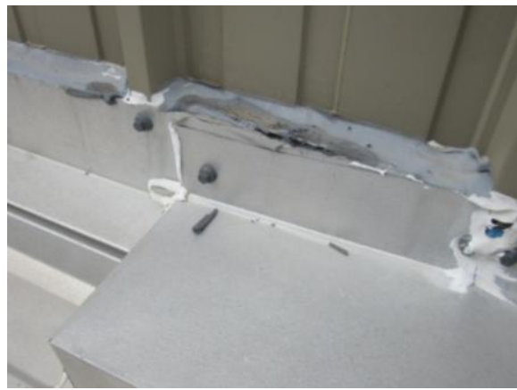
ST-H-3: Transition flashing has open joints or butt joints, or joints that are bucking water.
