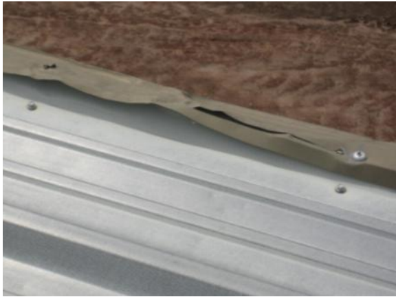
RE-H-1: Rake flashing has holes.
