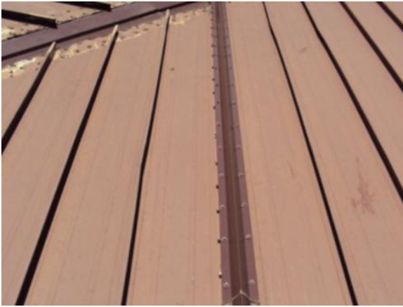
SW-L-1: Applied finish exhibits chalking, fading, or scratching over the entire roof section, but underlying corrosion is not apparent.
