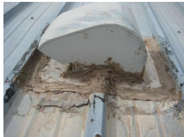
FR-M-1: Flashing patch, which appears to be performing a waterproofing function, appears to be watertight but requires a more permanent repair.
