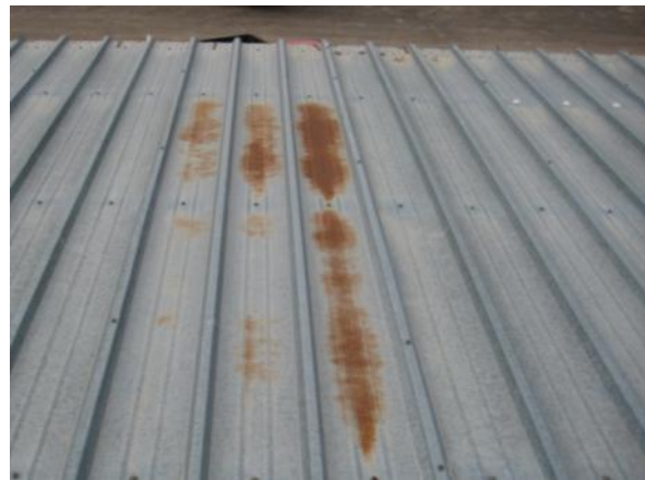
SD-M-1: Localized loss of applied finish or localized metal corrosion.
