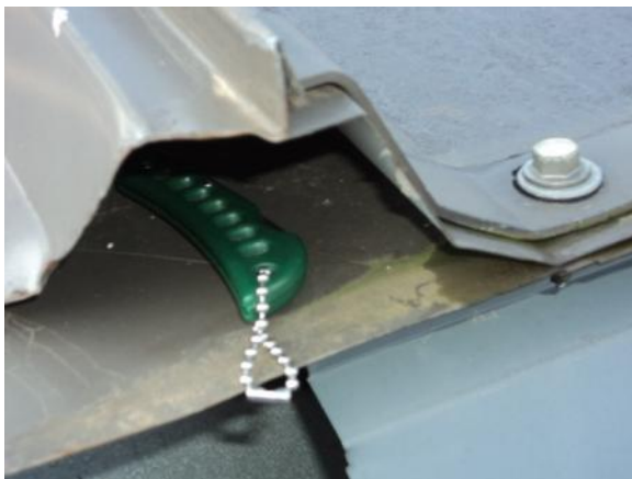
PC-H-1: Non-metal panel closure is deformed, misaligned, damaged or missing; allowing water to penetrate the roofing system.
