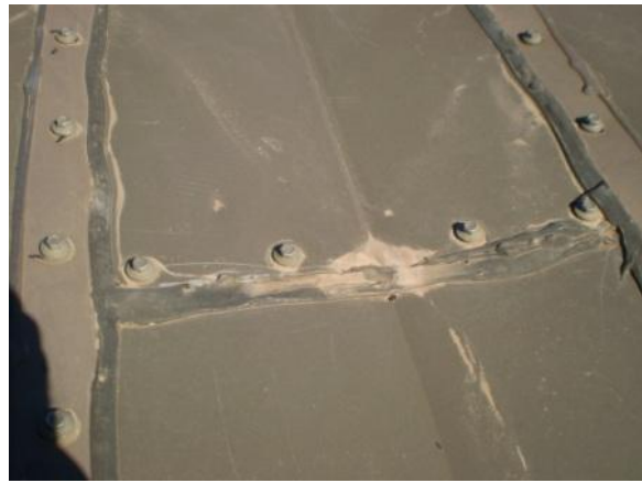
VF-L-1: Valley flashing fastener is located in the valley but appears to be watertight.
