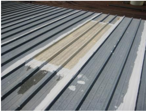
SP-L-1: Integrated skylight panels are rated low severity as a minimum due to their shorter service life as compared to the metal roofing system.
