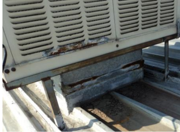
FM-H-1: Flashing impedes drainage.
