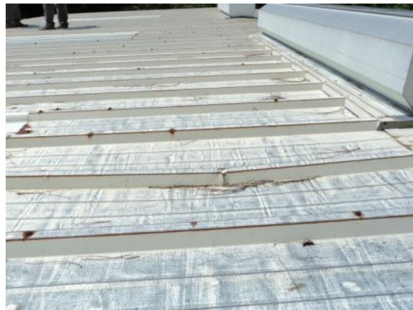
DP-M-1: Panel is dented, deformed or kinked, allowing ponding water and/or corrosion.
