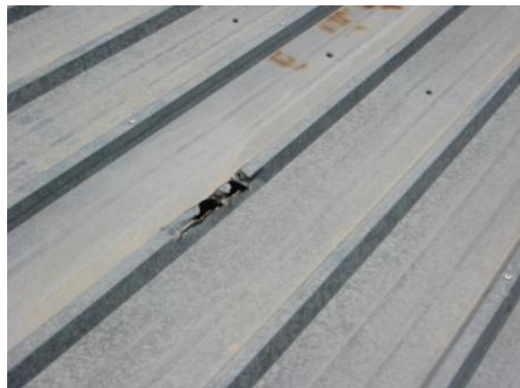
DP-H-2: For panel system that does not have mechanically interlocked seams; panel has holes, splits, or tears that require panel replacement.
