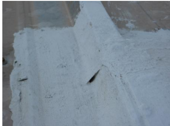
PA-H-1: Panel patch is allowing water to penetrate the roofing system.
