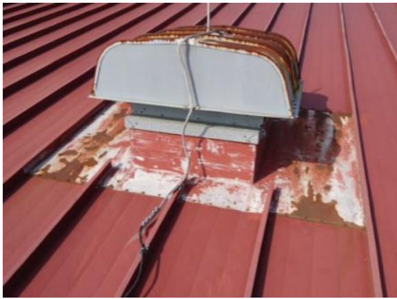
FD-M-1: Flashing has localized loss of applied finish or localized metal corrosion.
