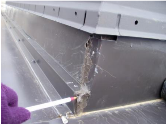
FM-H-2: Flashing has holes.
