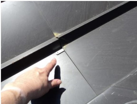
VF-H-3: Valley flashing has open joints or butt joint, or joints that are bucking water.
