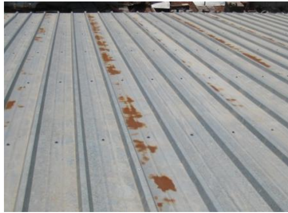
SW-M-1: Base metal or applied finish exhibits chalking, fading, or scratching over the entire roof section, requiring a coating or surface treatment repair.
