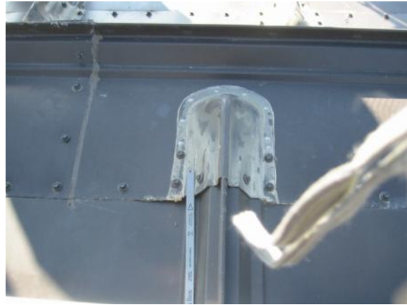
PC-M-2: Pre-manufactured seam cap does not fit properly.
