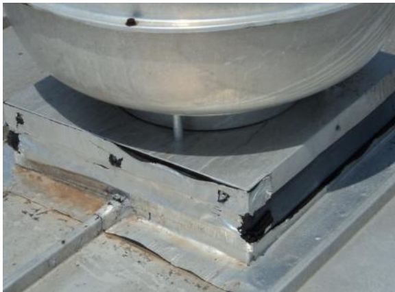
FM-H-7: Flashing flange is open or unsealed.
