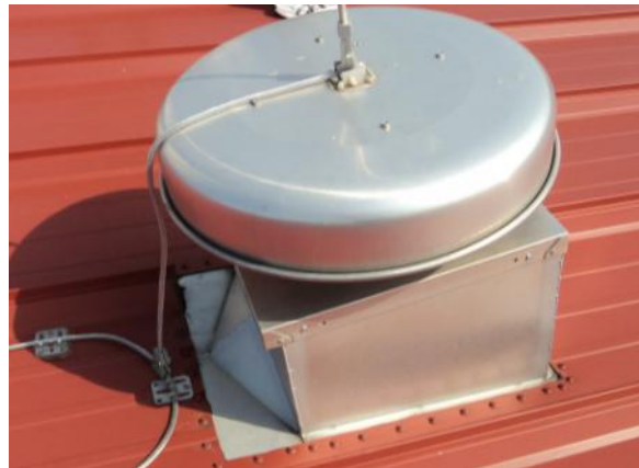
FM-H-5: Flashing flange on downslope side is mounted below panel, bucking water, and is allowing water to penetrate the roofing system.
