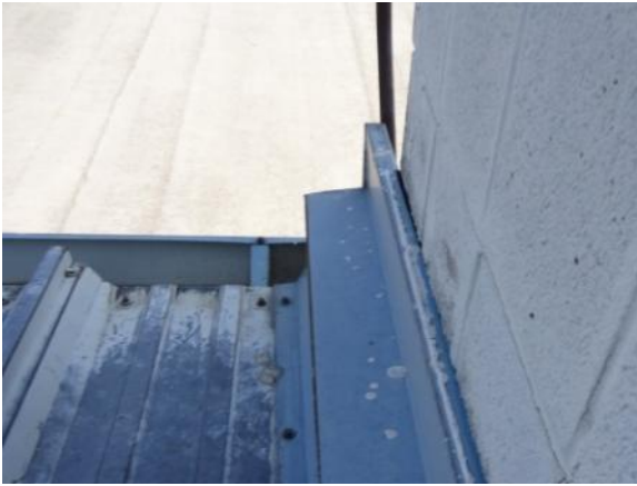
ST-H-2: Transition flashing is disengaged or loose and is allowing water to penetrate the roofing system.
