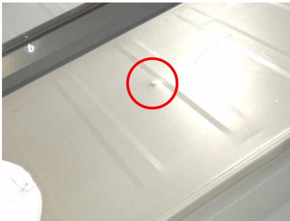
DP-L-1: Panel is dented, deformed, or kinked with no deformation of the seam, no loss of coating, and no corrosion; and appears to be watertight.
