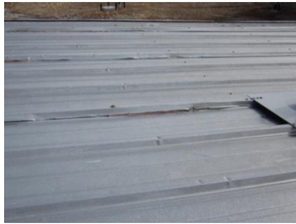
LS-H-2: Seam is open due to panel deformation, requiring panel replacement.
