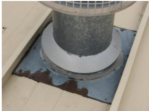
FM-H-9: Sealant around umbrella is missing or is allowing water to penetrate the roofing system.
