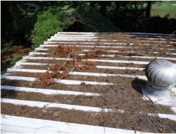
DV-M-1: A collection of foreign objects or vegetation not removed from the roof during the inspection; or grease, solvent, or oil drippings on the roof that cause no degradation of the panel's applied finish.
