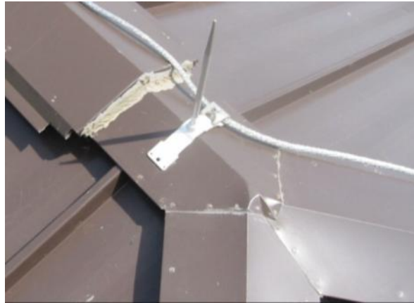
FR-M-1: Flashing patch, which appears to be performing a waterproofing function, appears to be watertight but requires a more permanent repair.
