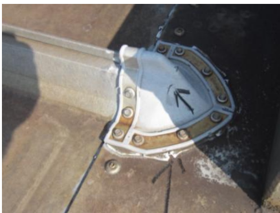
PC-H-2: Metal panel closure is deformed, misaligned, or missing; allowing water to penetrate the system.
