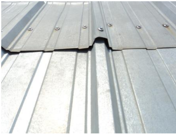
PL-M-2: End lap joint between panels has failed sealant or open fishmouths.
