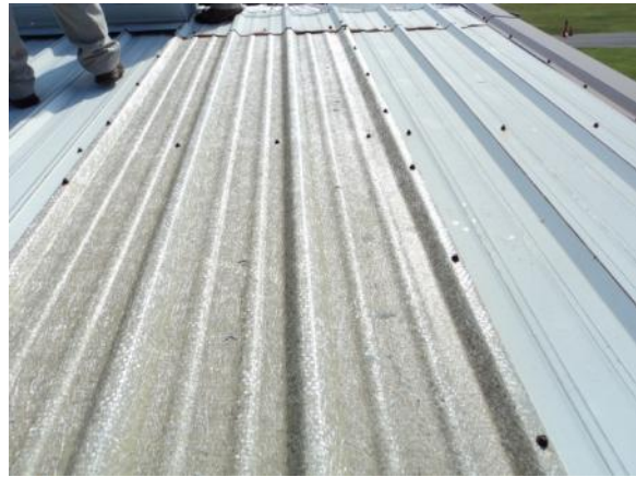
SP-M-1: Skylight composite material exhibits visible fibers, significant discoloration or other signs of degradation.
