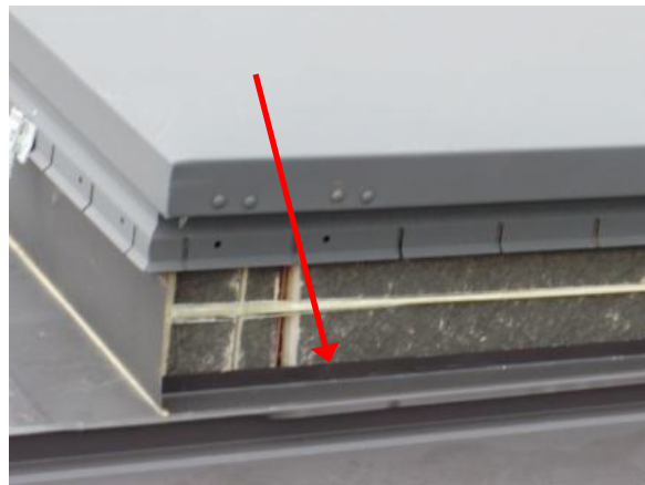
AF-H-9: Top of transition flashing is not properly counterflashed or terminated.
