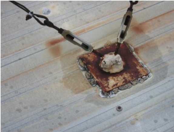
EQ-H-2: The equipment support has caused damage to surrounding panels and is allowing water to penetrate the roofing system.
