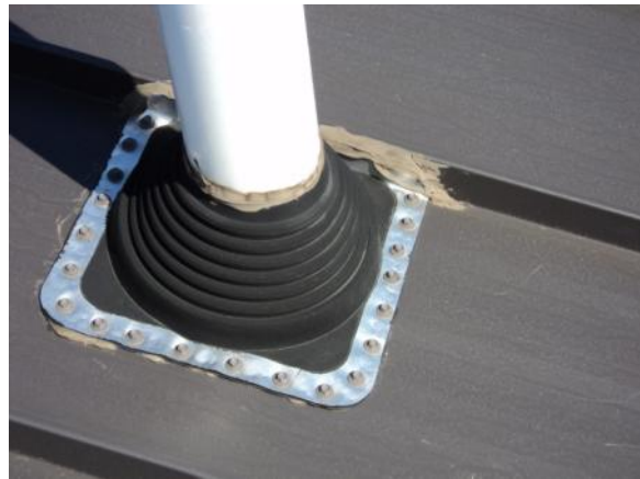
FB-M-1: Flexible boot flashing has loose, missing, corroded or misaligned draw band.
