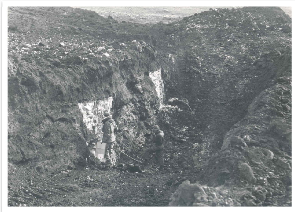
Figure 5. Ice wedges excavated at Thule in the 1960s (CRREL photo). Ice wedges such as these, located under the runway, are the cause of many previous localized depressions on the runway. Depressions that currently exist at 62+00 and 70+00 were drilled in 2009 and wedge ice was found at the 6 ft depth.
