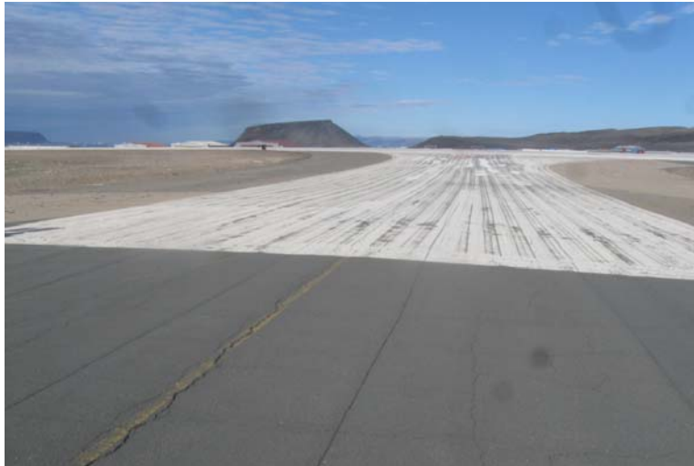
Figure 23. Old white paint transitioning to never painted surface at Txyw Bravo Extension. The white albedo measured 0.44 and the thaw depth measured 5.1 ft, while the black surface measured 0.15 and the thaw depth measured 6.5 ft.
