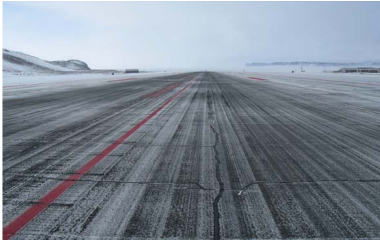
Figure 18. View of the 26 end of the runway April 2011. The winter maintenance has removed the white wash coating applied the previous summer. This state persists through the warm period of June, July and early August before repainting.
