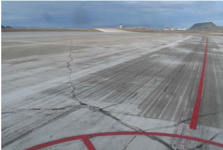
Figure 21. Brushed and faded milled surface on Txwy A at Vortac Calibration. Albedo measured at 0.26 and thaw depth measured at 5.3 ft.
