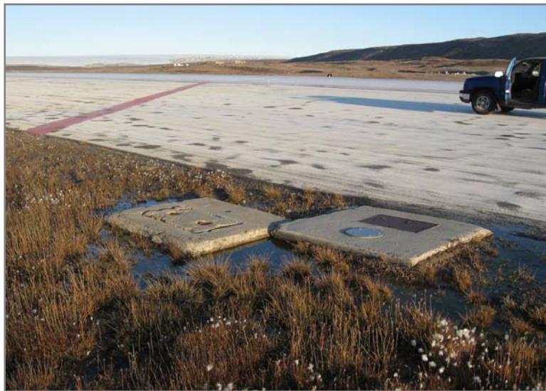
Figure 41. North shoulder of runway at 38+00. Seepage water is flowing from the electric vaults, and the visible splotchy asphalt of the shoulder is coincident with this area suggesting fatigue due to weakening of the base course or freeze–thaw problems. Water flows from the locations of the runway lighting early in the thawing season, slowly diminishing over the summer.
