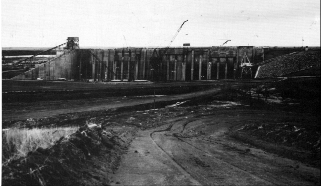
Photo 1-1. Upstream view of the Big Bend powerplant intake structure in final stages of construction prior to inundation.
