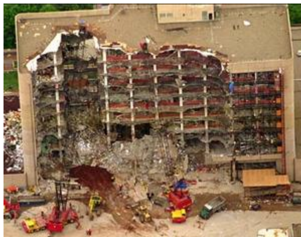
Figure 1: Damage done to Alfred P. Murrah Federal Building in Oklahoma City by 0.2 kiloton explosion. Source: wordpress.com
