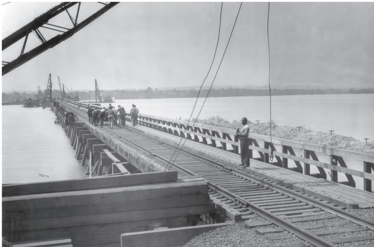
(Top) Emergency Railroad Bridge, August 1942. The Washington Engineer District built this additional, temporary crossing over the Potomac River from Shepherds Landing, D.C., to Alexandria, Virginia, to transport goods and troops in a national emergency. Authorities worried that the bridge immediately to the north was the only rail crossing of the southern Potomac River.
