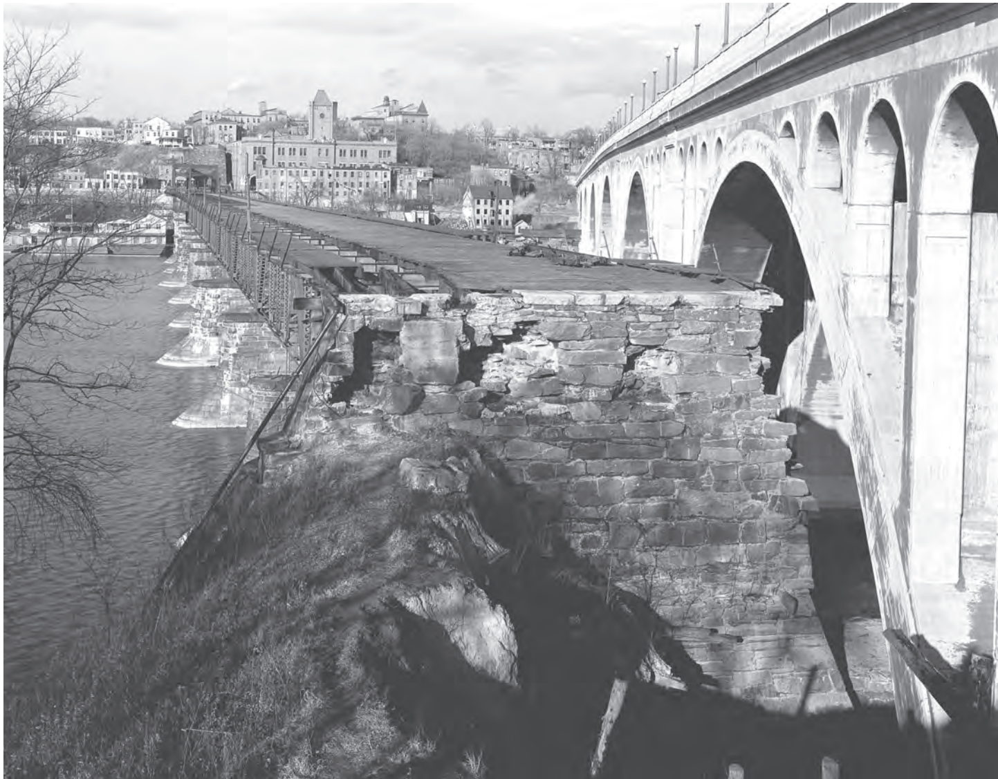
Aqueduct and Key Bridges intersecting near the Rosslyn shore, December 1929. The Aqueduct Bridge was largely dismantled several years after Key Bridge was opened for traffic in 1923. Office of History, Corps of Engineers
