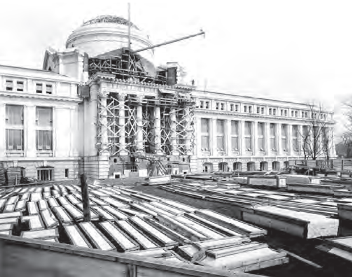
National Museum (later the Smithsonian's Museum of Natural History) under construction, March 1909. The dome and columns are partially completed and the stone slabs for the stairs encased in their wood shipping crates seen in the foreground.
