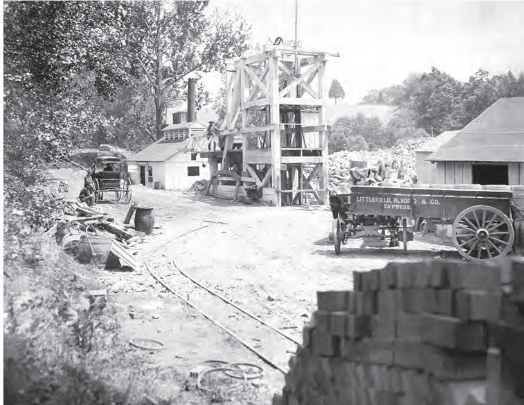
Foundry Branch shaft leading to the tunnel connecting the distributing reservoir and the new reservoir, 1884. The engineers built three shafts at Foundry Branch, Rock Creek, and Champlain Avenue. Washington Aqueduct Division, Baltimore Engineer District
