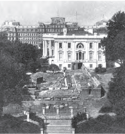
White House east entrance and terrace under construction, September 1902 Office of History, Corps of Engineers, Restoration of the White House Report
