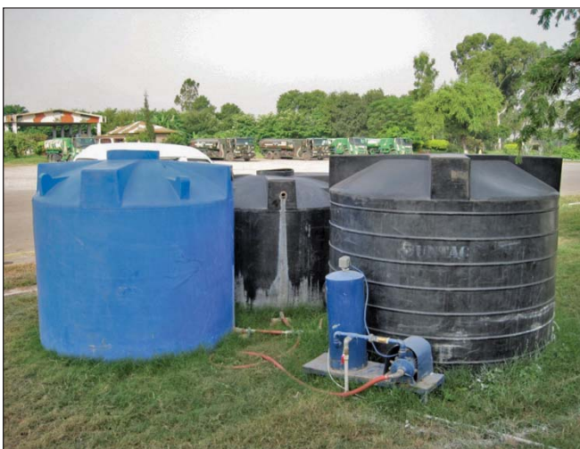
Figure 5. Bulk water tanks for the kitchen and dining facility.
