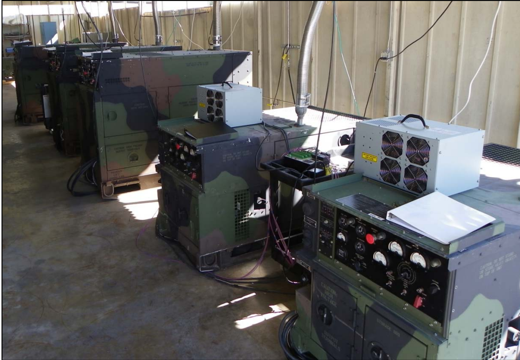
Figure 1. 10kW and 30kW Generators Ready for Testing
