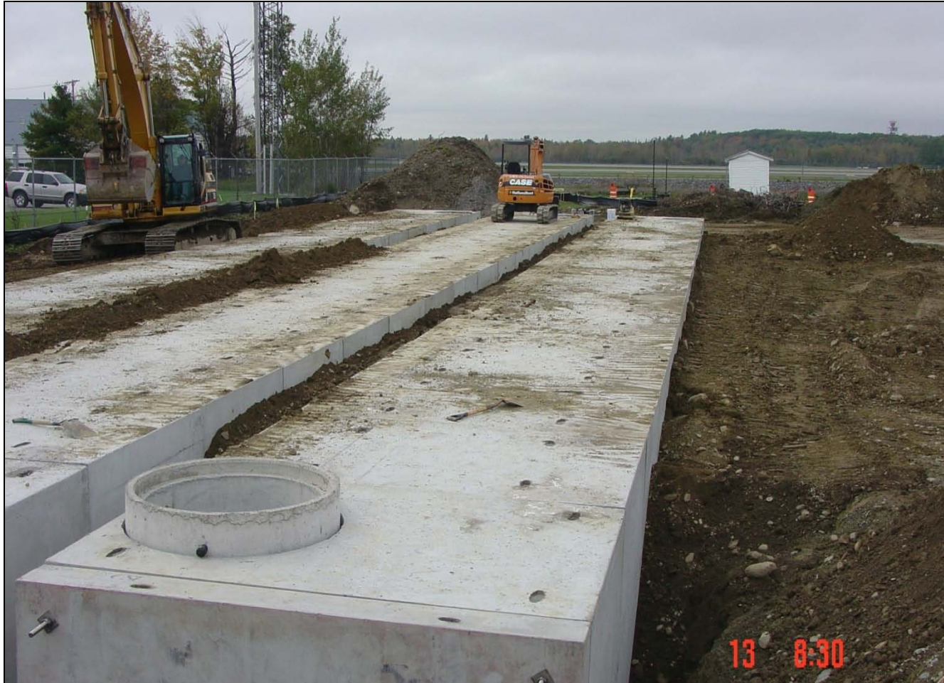
Three 57,000-gallon tanks that Maine ANGB uses as holding tanks prior to release of runoff to the POTW
