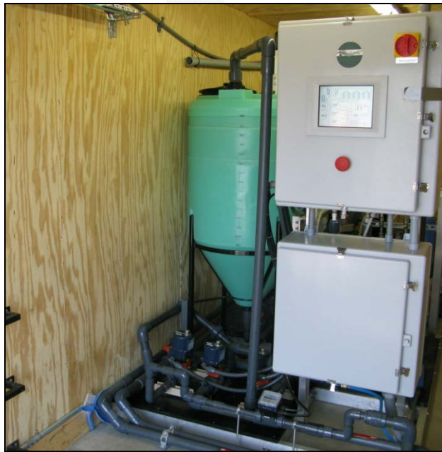
Control panel inside shed
