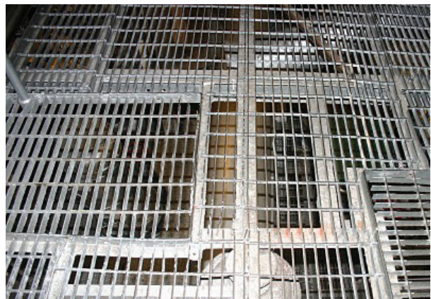
Figure 6. Deck grating between levels of an engine room. 3
