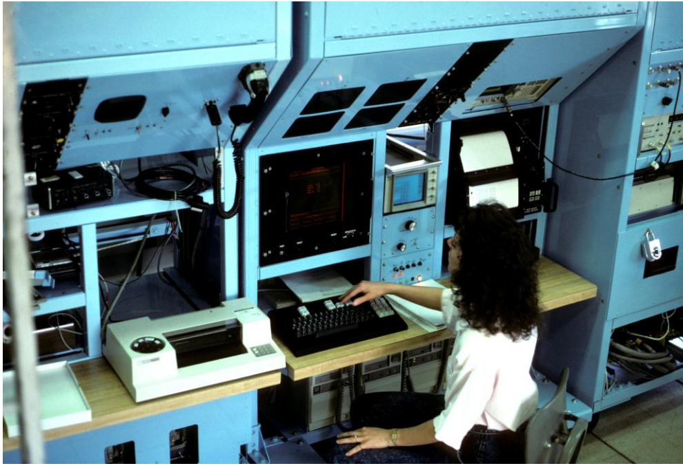
Figure 4 Milstar EHF SATCOM System in Rooftop Facility
