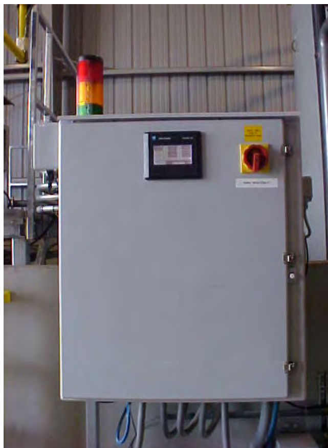
Figure 5-12. Motor control panel.
