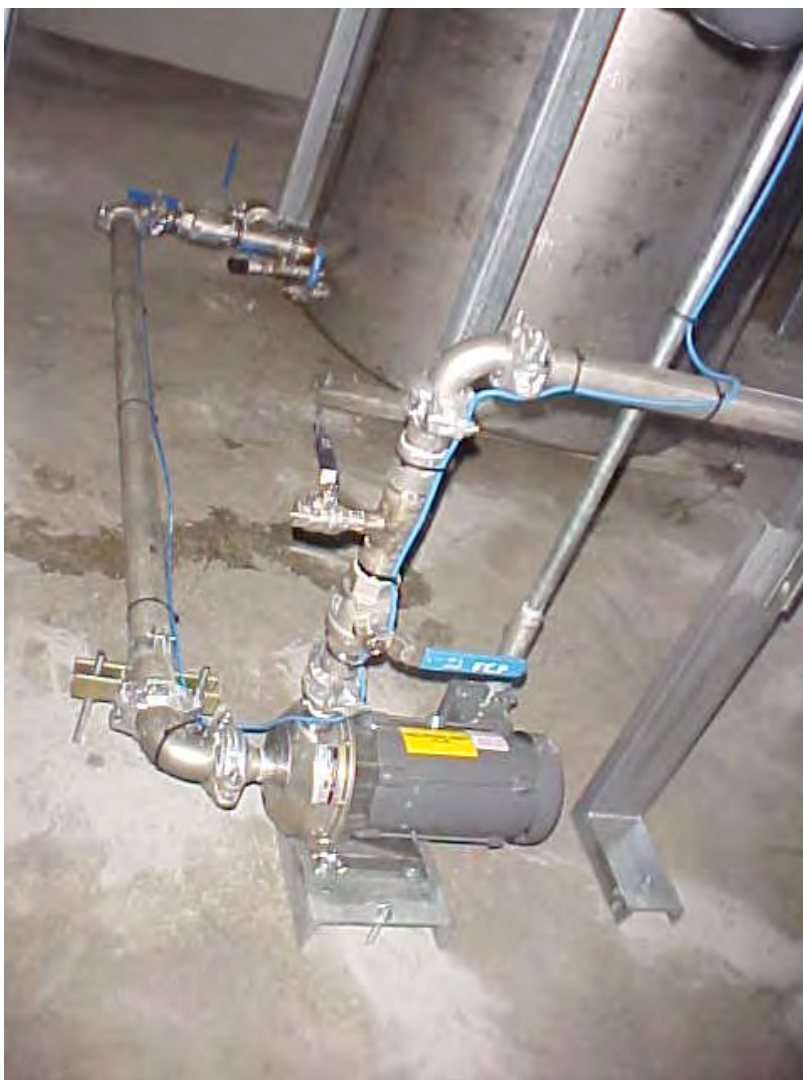
Figure 5-4. Mixing tank pump.
