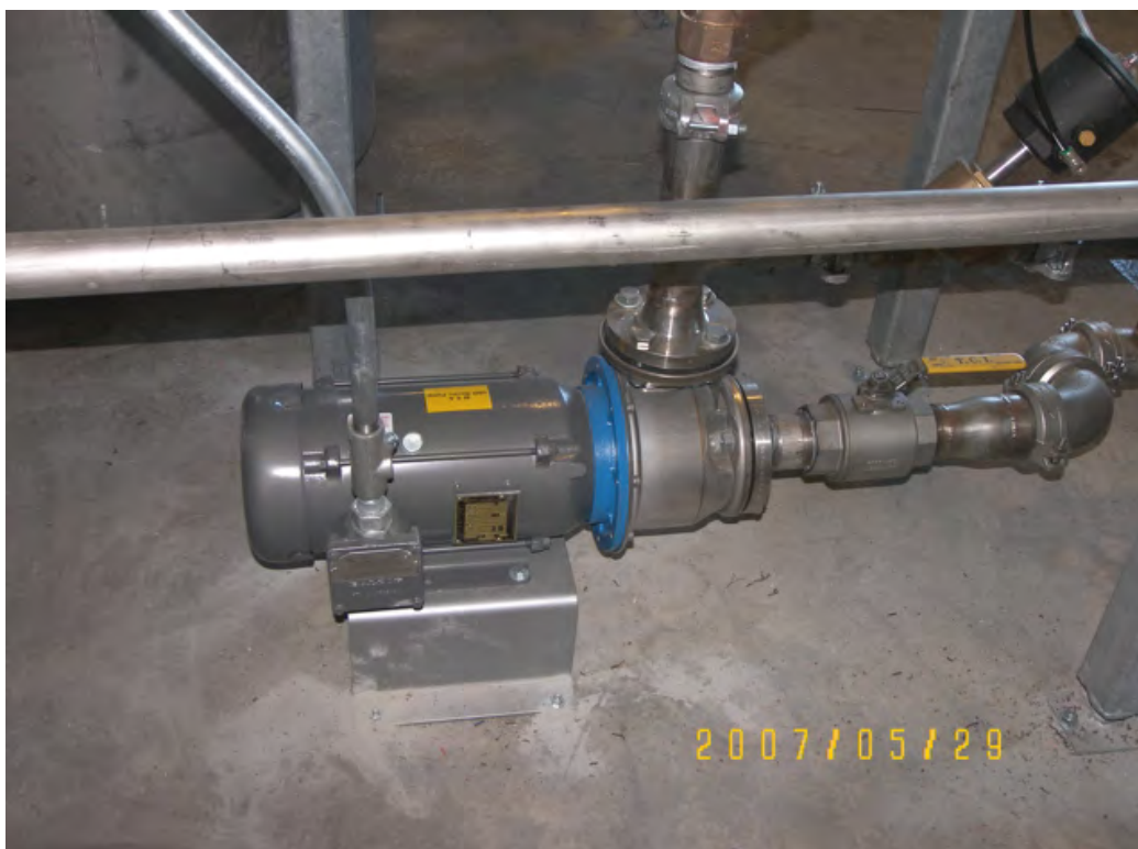
Figure 5-7. Reactor tank recirculation/transfer pump.
