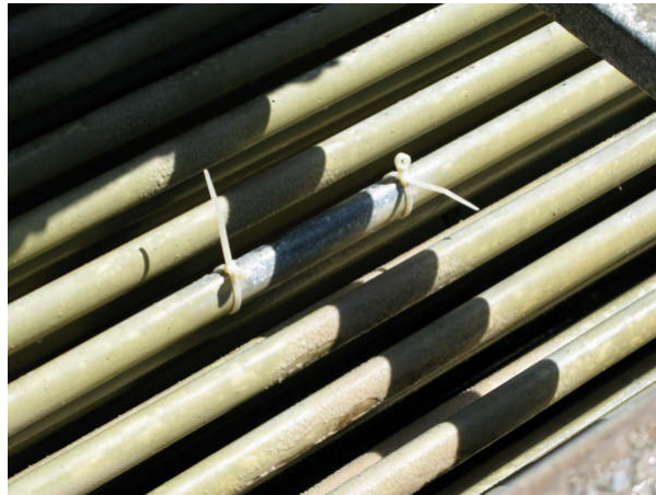
Figure 16. "After" photo of second clean section of upper tube of evaporative condenser at Zeta demonstration site (Davis Monthan AFB Fitness Center, September 2008).
