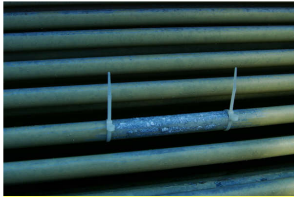
Figure 13. Mechanically cleaned section of upper tubes on the evaporative condenser at Zeta demonstration site (Davis Monthan AFB Fitness Center, July 2007).
