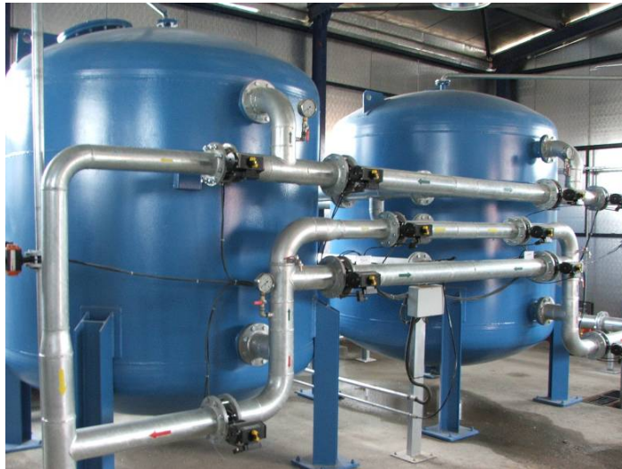
Site Photo 15. Tanks enclosing the 15 micron filters
