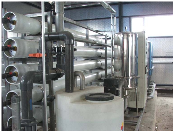
Site Photo 16. Reverse osmosis purification units
