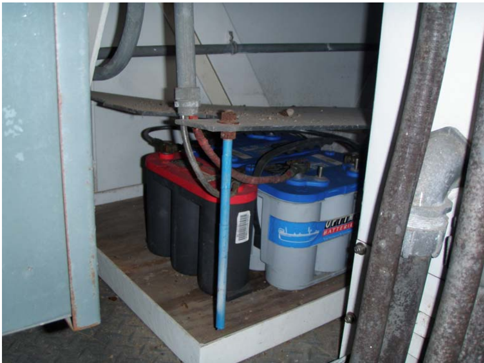
Photograph 82: Batteries located in the Tether Building.
