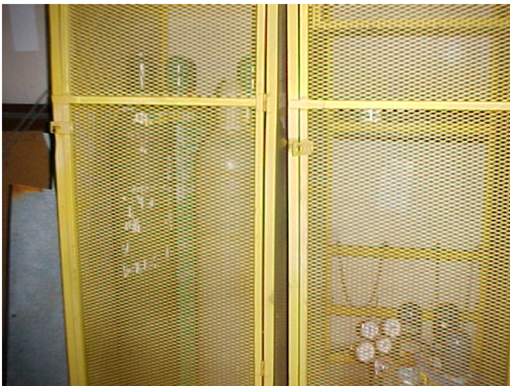
Photograph 48: Compressed cylinder storage in Payload Service Building #003. Oxygen, nitrogen, sulfur hexafluoride, and breathing air.
