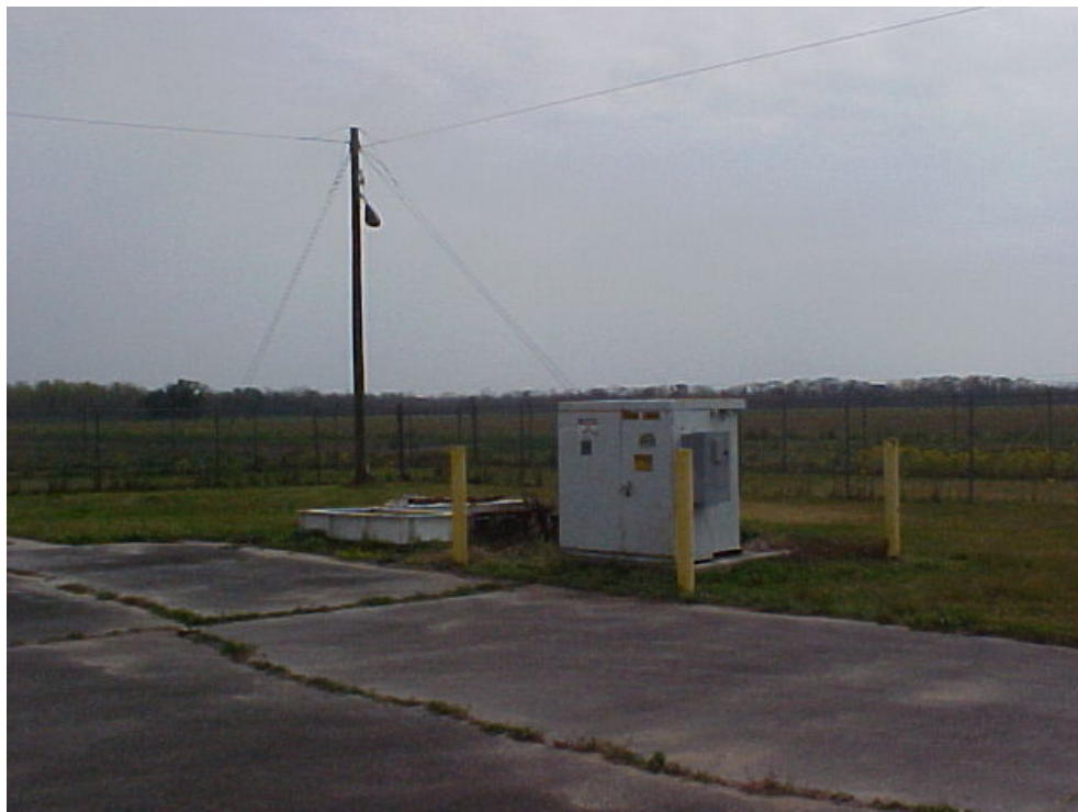
Photograph 83: Site Transformer. Southeast section of site.
