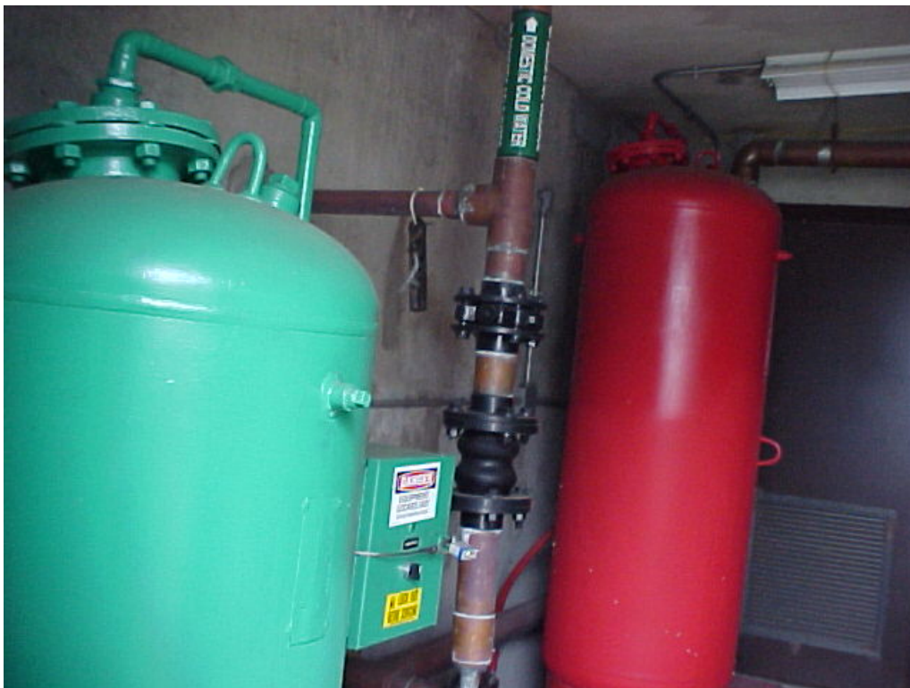
Photograph 61: Interior of the Pump House and pump equipment.
