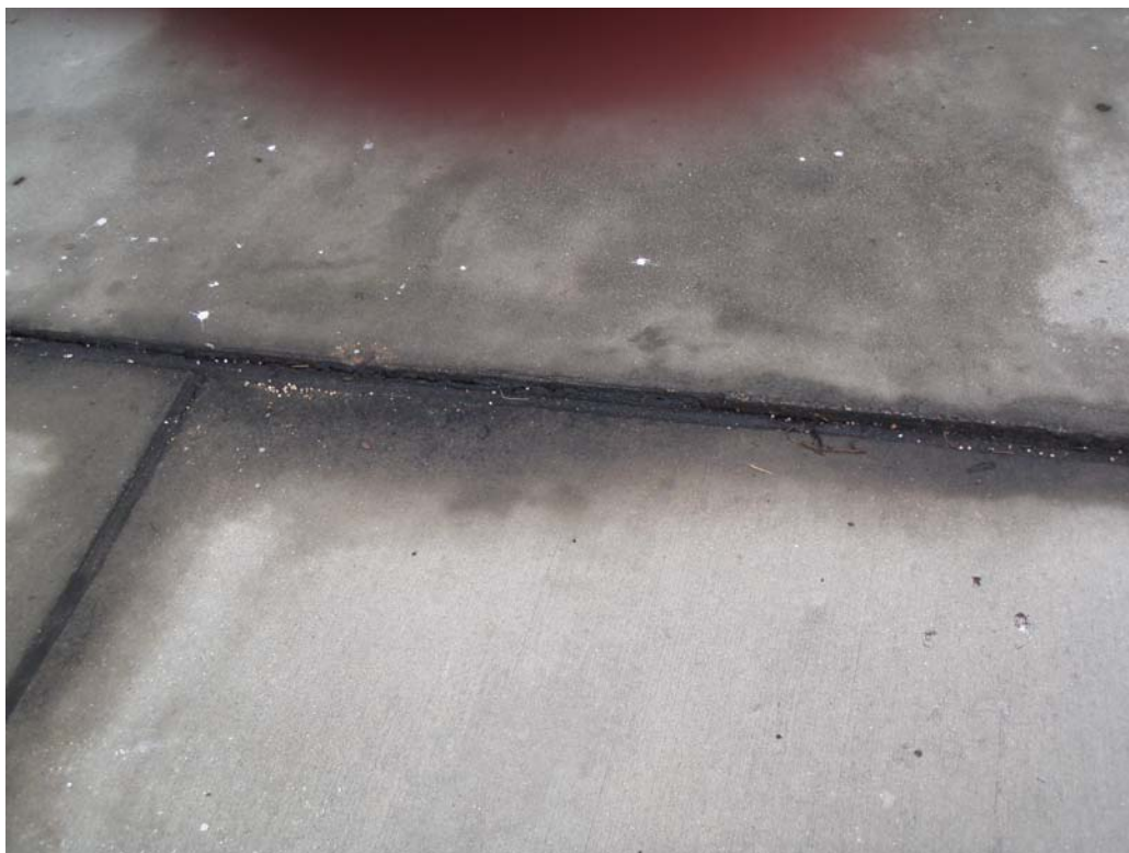
Photograph 74: Concrete staining immediately under the Tether Mooring Building pillar. Note: red at top of photo is finger in front of the lens, not staining.
