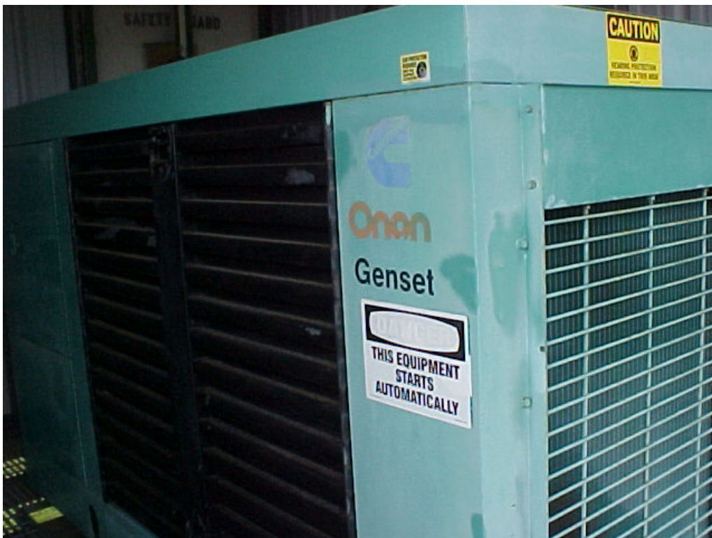
Photograph 64: Generator located in the Generator Enclosure.
