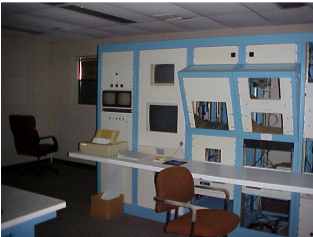
Photograph 13. Control center panel. Equipment removed. Located in the Operations Building #001.
