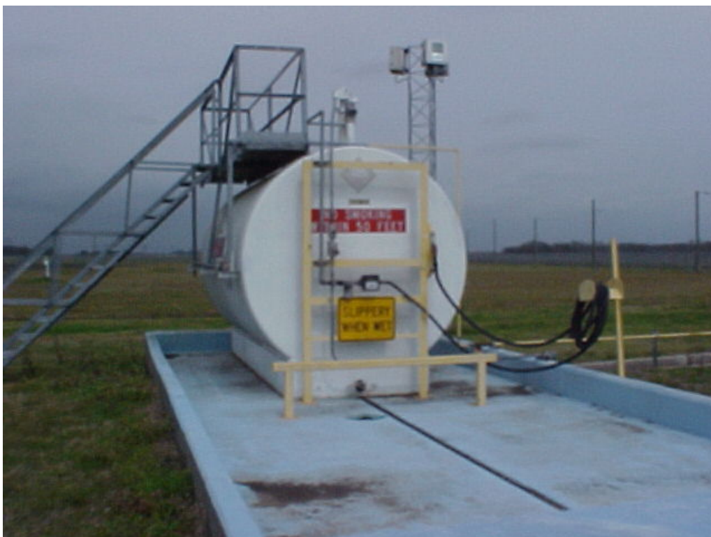
Photograph 66: Diesel Fuel Storage (4,750-gallon capacity), and secondary containment structure. Note aboveground fuel line in center right of the photograph.
