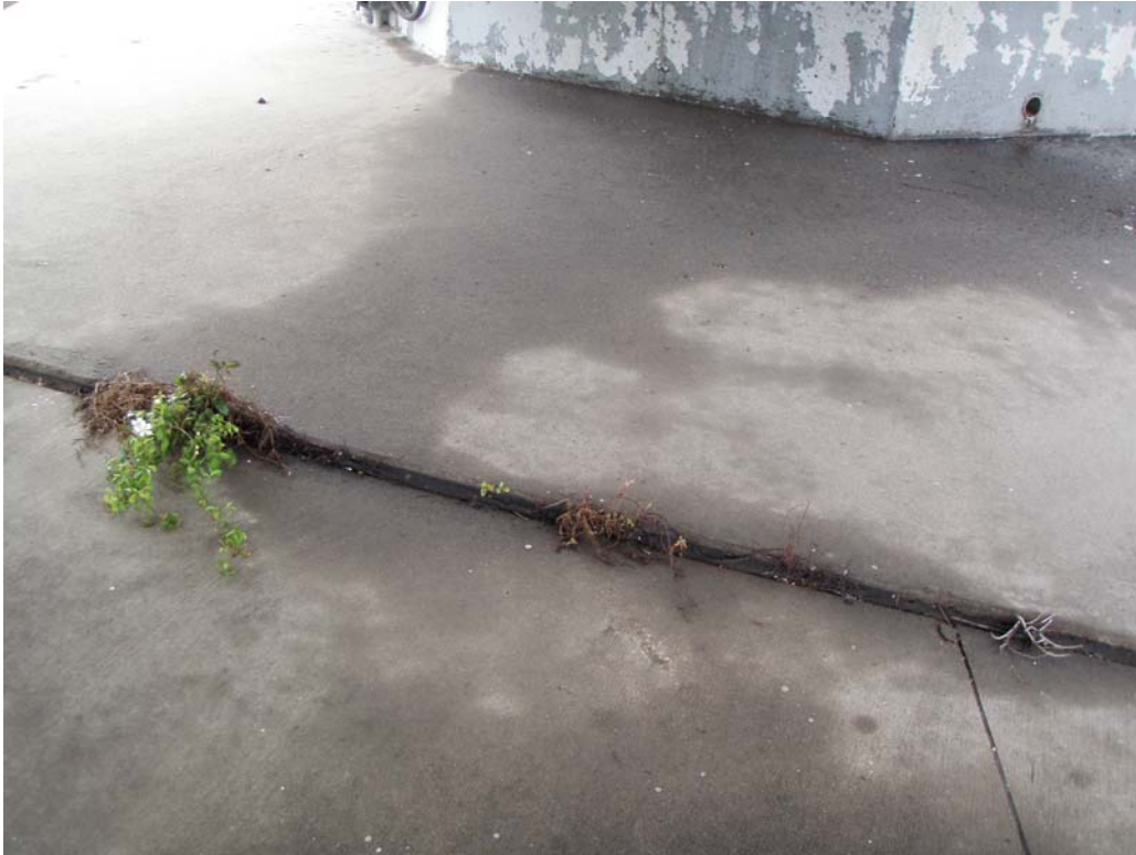
Photograph 75. Additional photo of concrete staining immediately underneath the Tether Building pillar.
