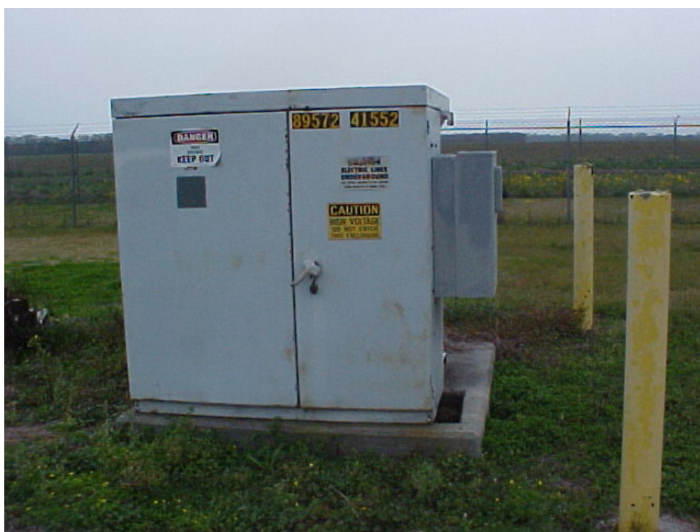
Photograph 84: Closer view of same transformer on southeast section of site.
