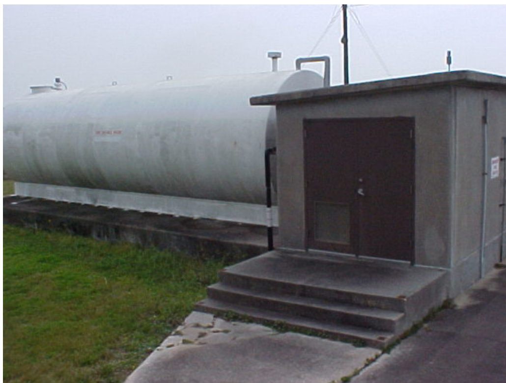
Photograph 60: Pump House and the 20,000-gallon water storage tank for firefighting.
