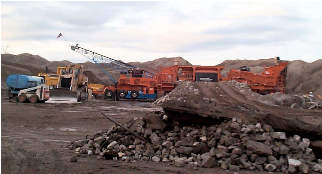
Figure 1. Overview of crusher plant.
