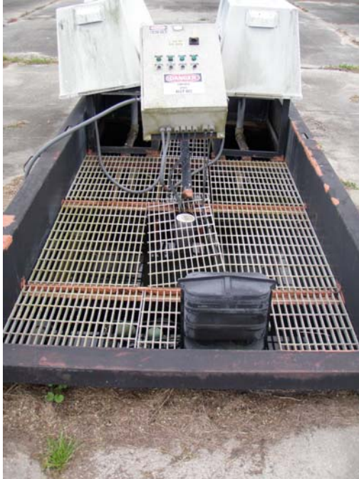
Photograph 69: Control panel and tanks for the wastewater treatment plant.
