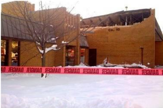
Roof collapse in Virginia at the Fairfax County Fire Department following heavy snowfall in February 2010.
