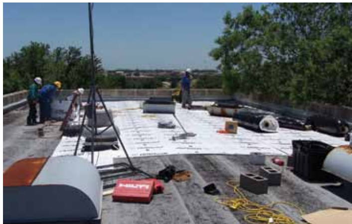
Workers finish the roof of a “green” building under construction at Fort Hood, Texas. The building is designed to meet the U.S. Green Building Council’s Leadership in Energy and Environmental Design (LEED®) silver-level criteria.
