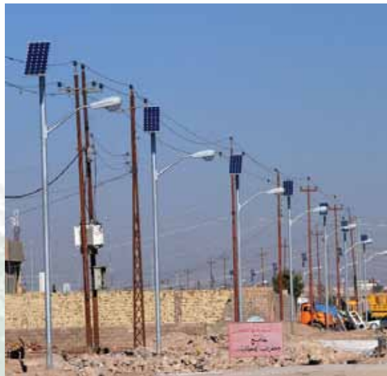
As many as 800 solar-powered street lights have been put up in Fallujah by the Army Corps of Engineers, and the Corps expects to place as many as 600-700 more.
