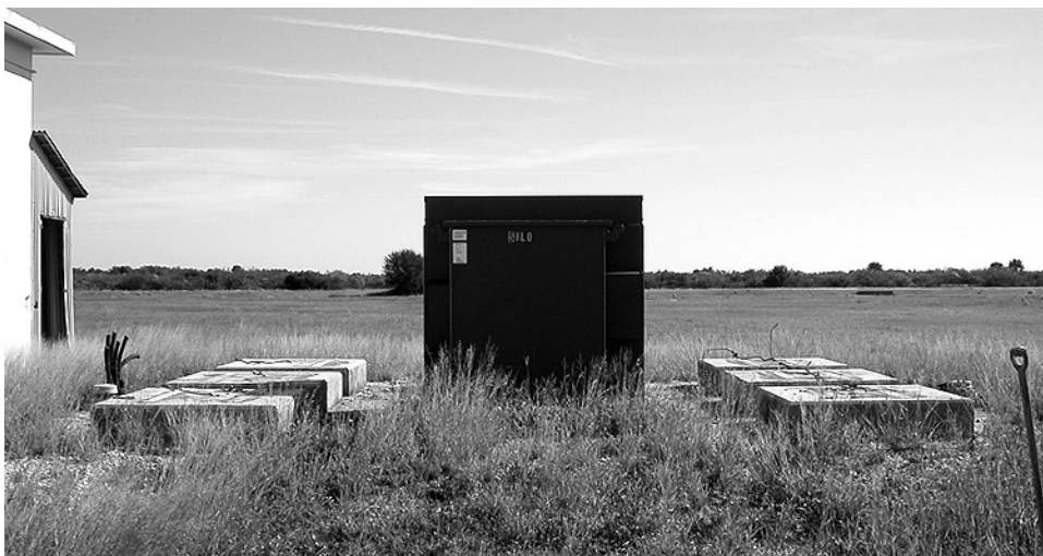
Figure 67. Launch support building transformer vault (ERDC-CERL 2007).
